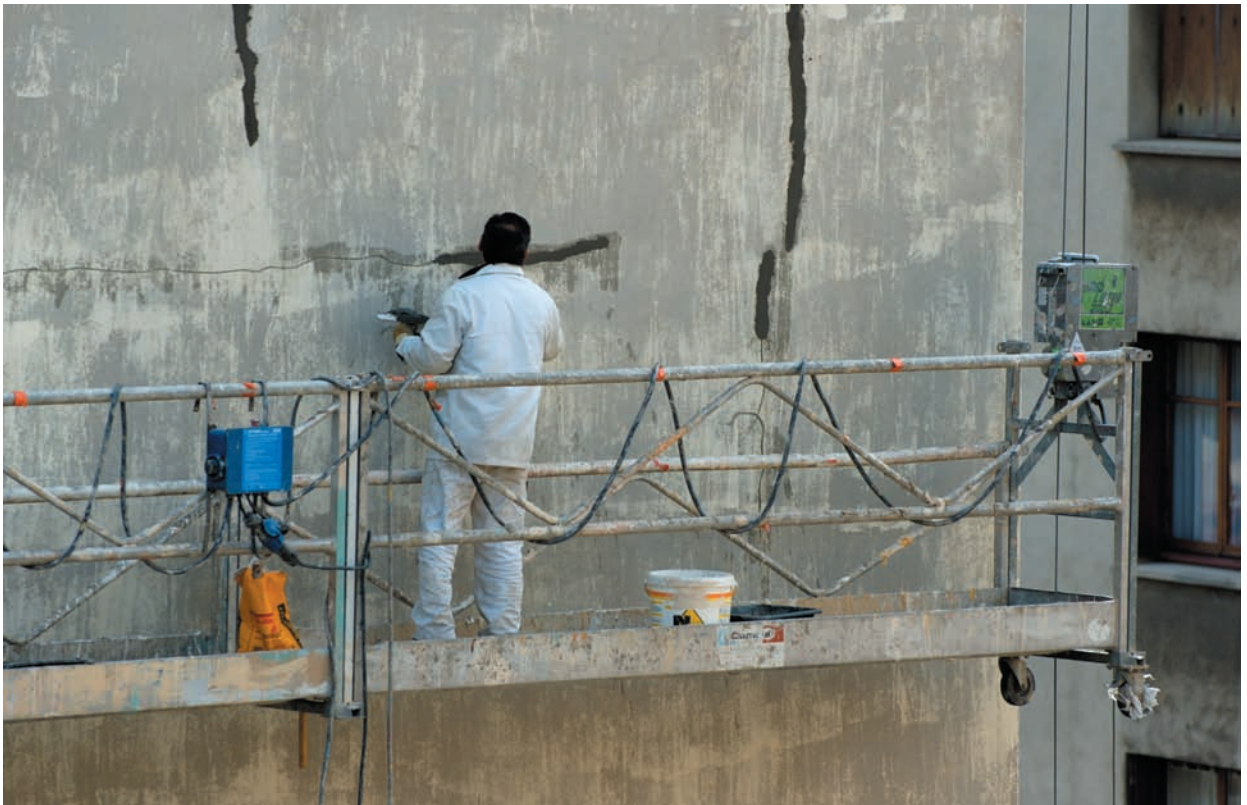
Figure 14.6 Is the man painting with cracks?
