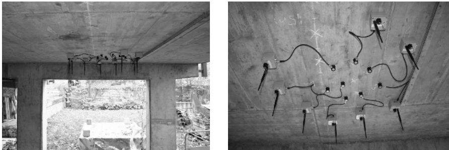
Fig. 15.5. Overview of setup for wireless AE measurements at the Stuttgart “ramp” ( left ) and wireless AE array setup ( right ).
