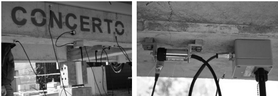
Fig. 15.4. “Concerto Bridge” in Brunswick equipped with wireless AE sensors (left) and with wireless strain sensors (right).
