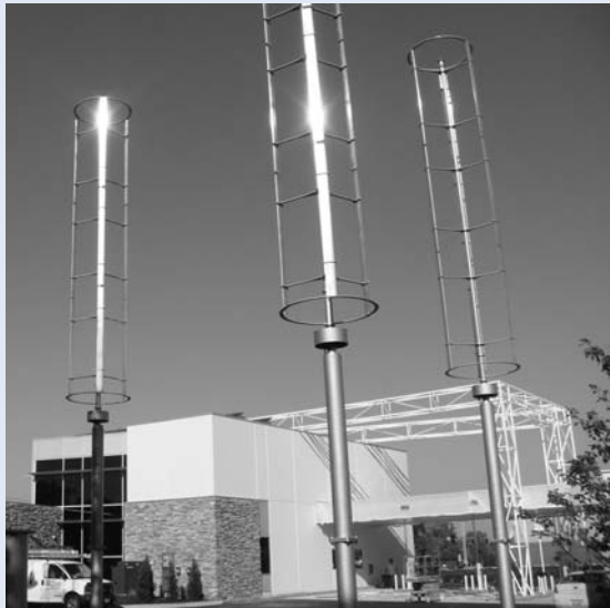
Windspire Turbines. (Picture Courtesy of Windspire Energy.)
