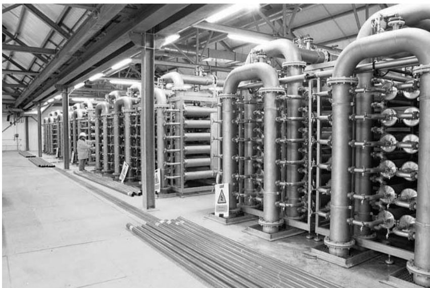
Figure 7.19 Photograph of a 25 million gal/day capillary hollow fiber module plant to produce potable water from a well, installed by Norit (X-Flow) in Keldgate, UK. Courtesy of Norit Membrane Technology BV
