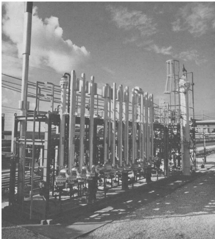
Figure 8.22 Photograph of an Air Products and Chemicals, Inc. PRISM ® membrane system installed at an ammonia plant. The modules are mounted vertically
