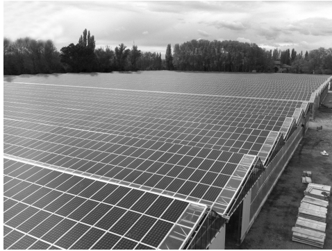
Figure 3.6 Greenhouse Solar Panel System (Courtesy of ININSA Greenhouses, www.fabricanteinvernaderos.com/english/ ).
