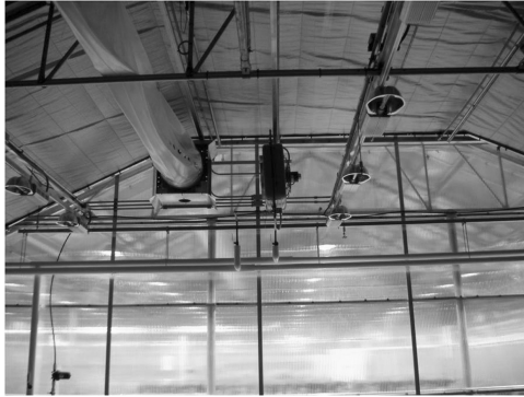
Figure 5.99 Unit Heater used with Convection-Tube Air Distribution System (Courtesy of American Plants Products & Services, Inc.).
