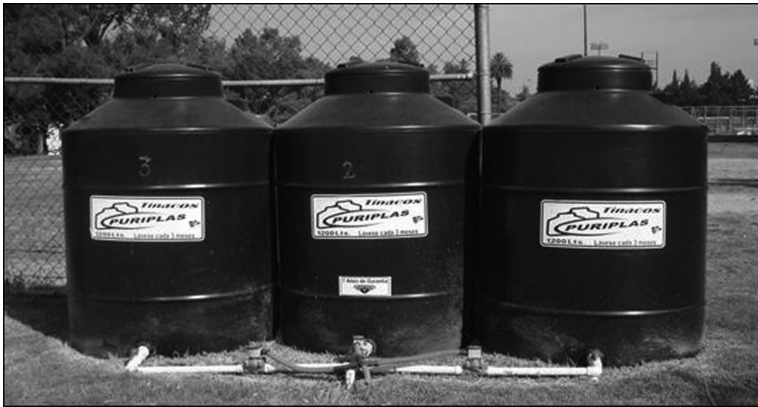
Figure 6.18 Nutrient Storage Tanks.
