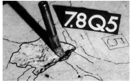
Fig. 4.62 Shell-shaped concrete spalling for a headed stud remote from an edge when subjected to shear (taken from Fuchs (1990) )
