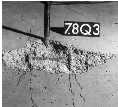
Fig. 3.2 Concrete cone failure of an anchor located close to an edge and loaded in shear towards the edge
