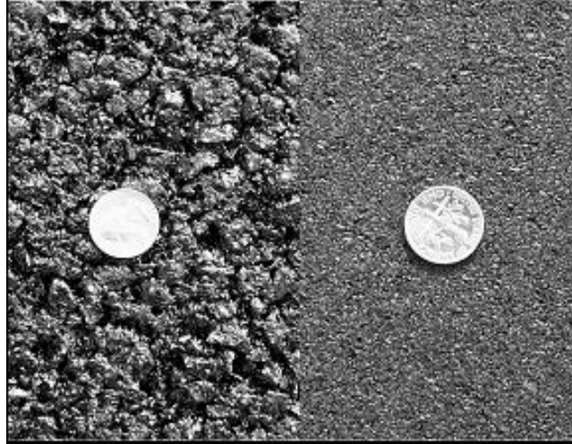
FIGURE B9 (Left) Thin open-graded hot-mix overlay surface; (Right) Dense-graded overlay surface. Diameter of the coins is 0.7 in.
