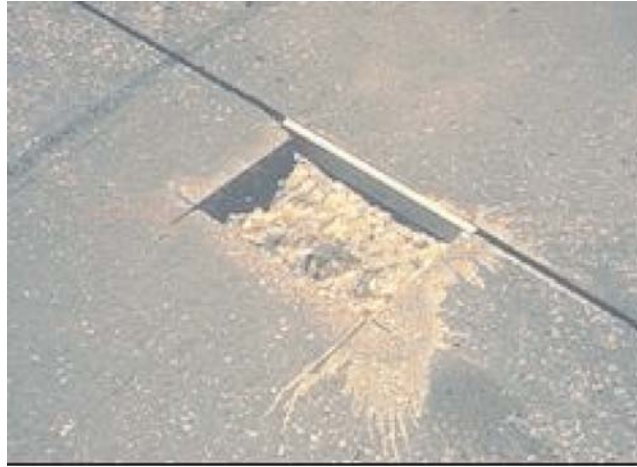
FIGURE B11 Prepared repair area; the insert, separating the repair area from the joint, extends beyond the saw cut into the existing longitudinal joint.
