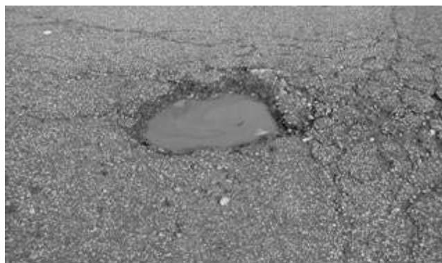
FIGURE B5 Untreated pothole collects water and accelerates pavement deterioration.
