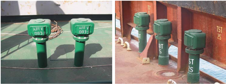
FIGURE 149 DB tanks' ventilators.
