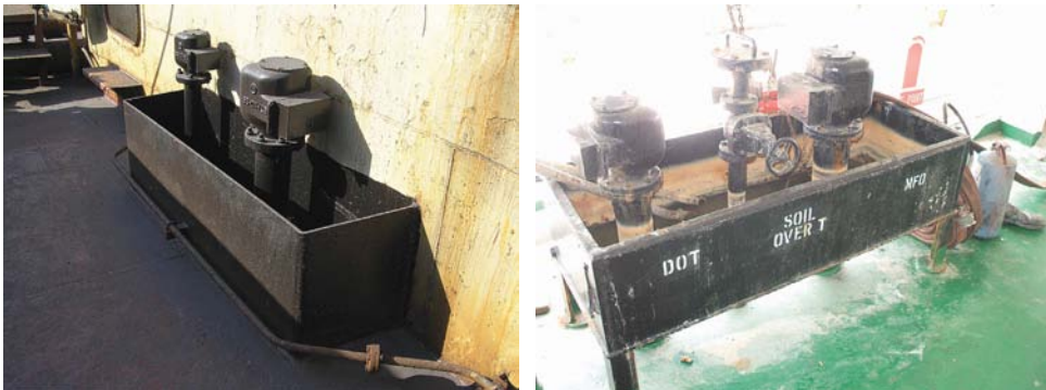
FIGURE 150 Save-all for DB tanks' vents.
