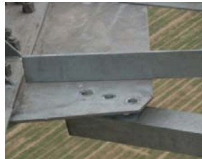
Figure 12. Loosen bolts at cross arms
