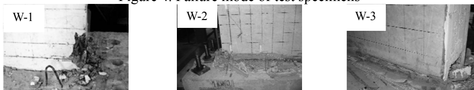
Figure 5. Damage of the wall toes on W-1, W-2 and W-3
