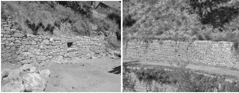
Figure 1.1. Dent repairs on two dry stone retaining walls. Left, repair in progress, granite (photo: Bruno Durand); right, after restoration, limestone (lighter part on the right) (photo: Paul McCombie)
