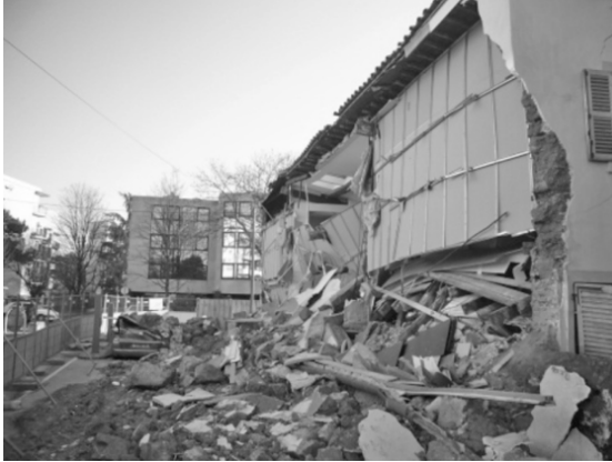
Figure 1.4. Collapse of a rammed earth house wall due to excessive water content of the walls at the base as a result of capillary action which was then unable to evaporate
