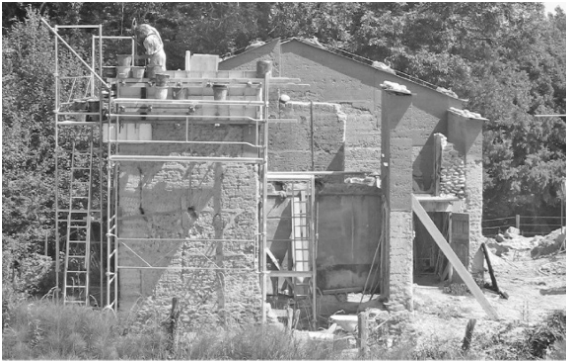
Figure 1.2. Renovation of a rammed earth house, raising walls by the Nicolas Meunier company (photo: Nicolas Meunier)
