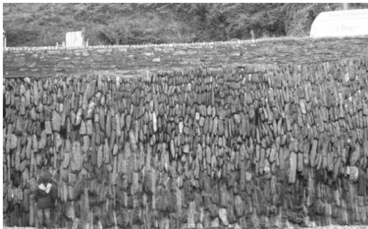
Figure 11.4. Roadside retaining wall with typical claved masonry walls in contact with water. The wear of the stone (shale) by the tide in the lower part of the wall is very visible. About 4 meters high (Cornwall, UK)
