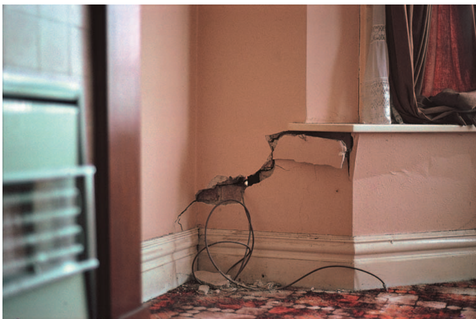
FIG 3.12 Subsidence damage inside house.
