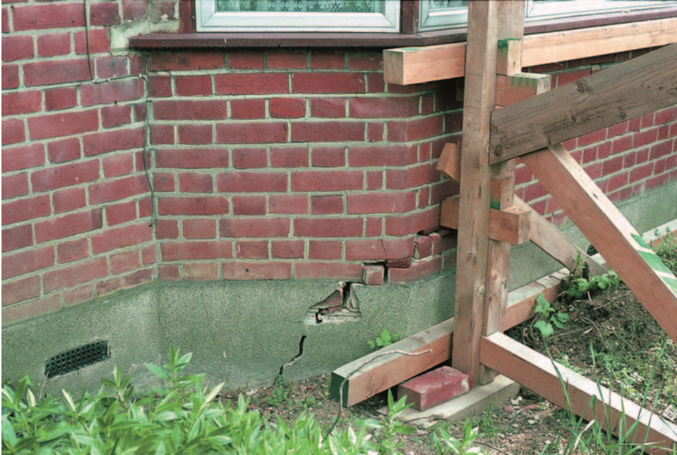
FIG 3.13 Subsidence damage outside house.
