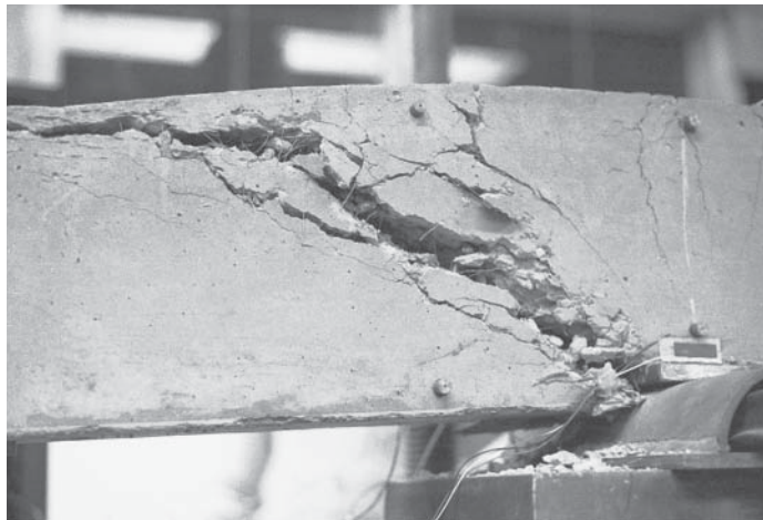
Shear failure near a middle support.
