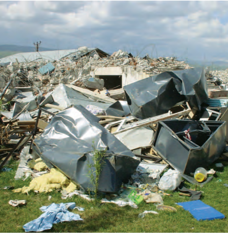
The Celtiksuyu Boarding School lay in ruins after the May 2003 earthquake (Richter scale 6.4) hit Bingol, Turkey.
