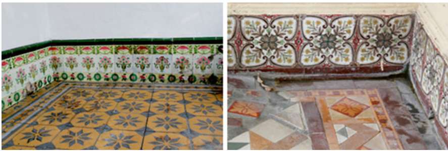
Fig. 42.7 Façade wall and floor tiles of shophouses along Heeren Street in Malacca (Photos by Wang Cheng Yong in October, 2014)
