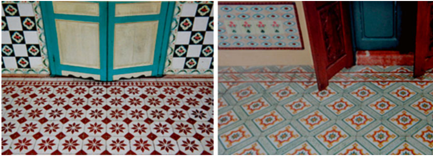
Fig. 42.6 Façade wall and floor tiles of shophouses at Blair Plain in Singapore (Extracted from Singapore Shophouse by Davidson ([15], p. 57). Singapore: Talisman Publishing Private Ltd)
