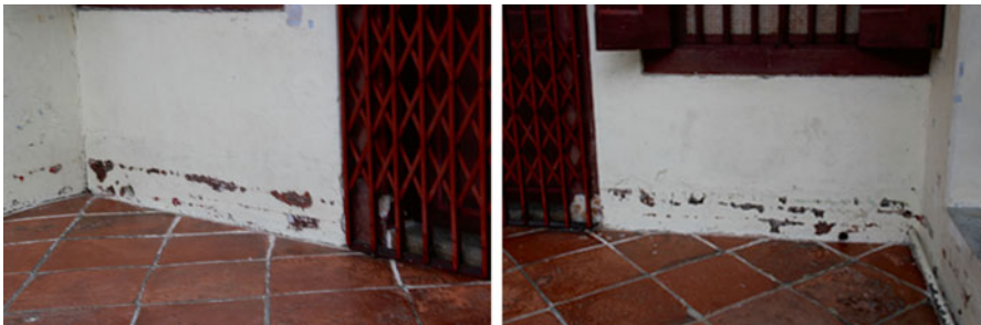
Fig. 42.3 Telling signs that tiles could be ripped off the façade wall of a Peranakan shophouse in Malacca (Source: photos by Wang Cheng Yong, 2014)
