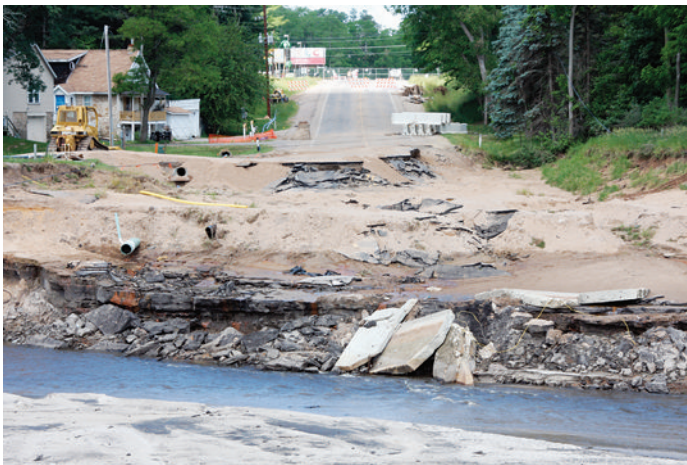
FIGURE 3-3. Lake Delton, Wisconsin, June 23, 2008. Bridges, roads, and houses are damaged at Lake Delton as flood waters compromised a dam that eroded the lake basin and walls, draining the lake into the nearby Wisconsin River. Damage to local infrastructure may compromise the hospital's ability to access warehouses and other outside sources of aid in a disaster. Photo by Robert Kaufmann/FEMA.
