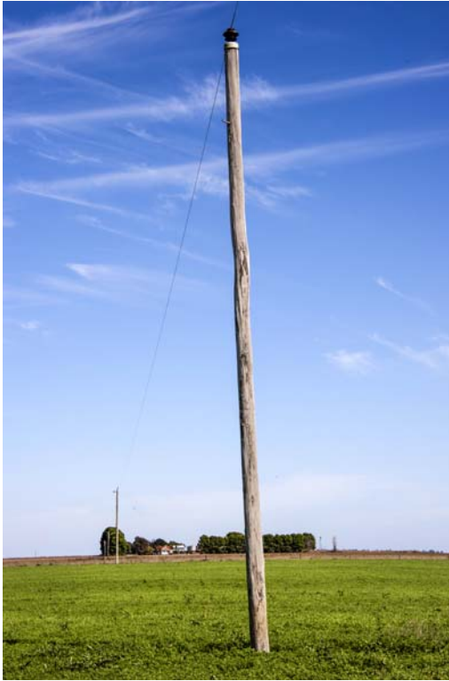
Figure 12.4 Typical timber utility pole used for power transmission.
