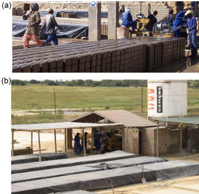
Figure 8.16 Curing of CSEB in a block yard. (a) Newly produced blocks are sprayed with water in preparation for curing. (b) Blocks are covered with black plastic sheeting. Hydraform, 1988. Building Breakthrough – Product Information . Hydraform Africa, Johannesburg.
