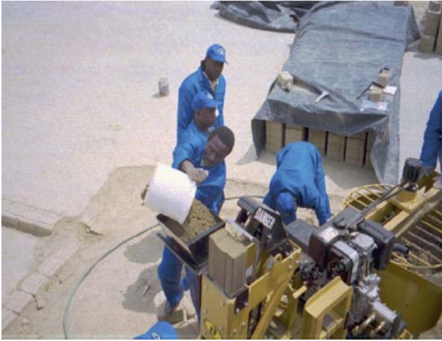
Figure 8.11 Soil-cement mix being loaded into the hopper. African Standards Organisation, 1996. Standards on CEB Construction: Compressed Earth Block Masonry ARS 670: Part 4: Code of Practice for Production and Construction.
