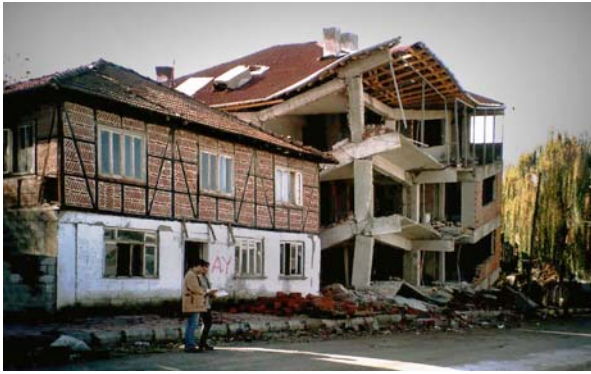
Figure 1.26 View after the 1999 Düzce, Turkey, earthquake showing collapsed reinforced concrete building immediately adjacent to a traditional humuş residence with only one panel of brick infill missing. Photographer unknown, image provided courtesy of Adem Dogangun.
