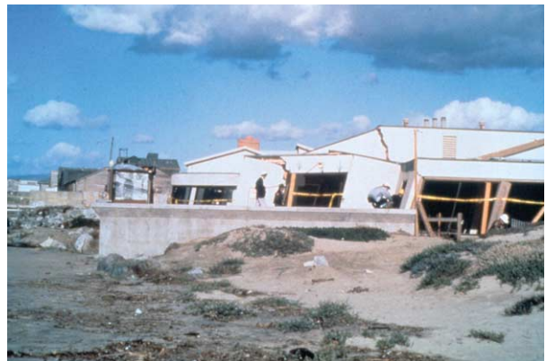
Figure 14 Damage to the Marine Laboratory at Moss Landing, Monterey Bay, California, during the 1989 magnitude 6.9 Loma Prieta earthquake. Lateral spreading caused the building pad foundations to spread apart. The laboratory was subsequently demolished. Photograph by Leslie F. Harder, Jr.
