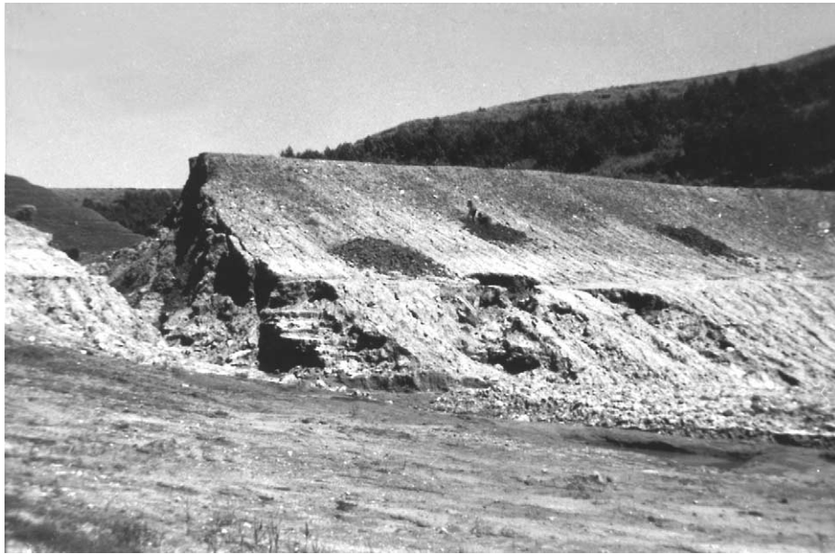
Figure 6 Failed earth dam constructed of dispersive soil, showing piping outlets on the downstream side, near Ramsgate, South Africa.
