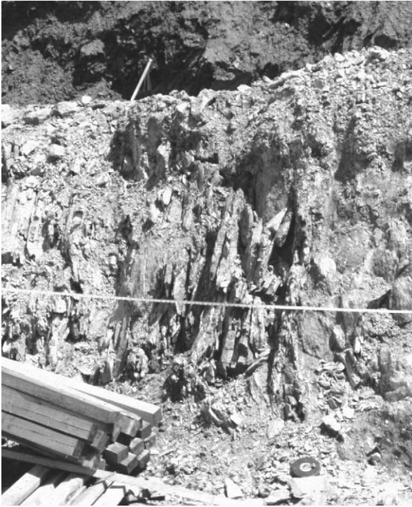
Figure 2 An example of a zone of ‘bad ground’ discovered and delimited in an engineering geological site characterization exploration. This zone represents poor engineering properties of foundation materials in terms of their ability to support structural loads that would be imposed by engineered works. Shown is a shear zone of ancient tectonic origin, as it perpendicularly enters the foundation excavation for the Lahey Medical Clinic, urban Boston, Massachusetts. Such features are important when they are planar to and cross one or more dimension of the foundation excavation, because they have the potential to induce instability of the surrounding ground and existing buildings. Timbers are 200 mm 2 in section; survey tape in midview. Photograph by the author.
