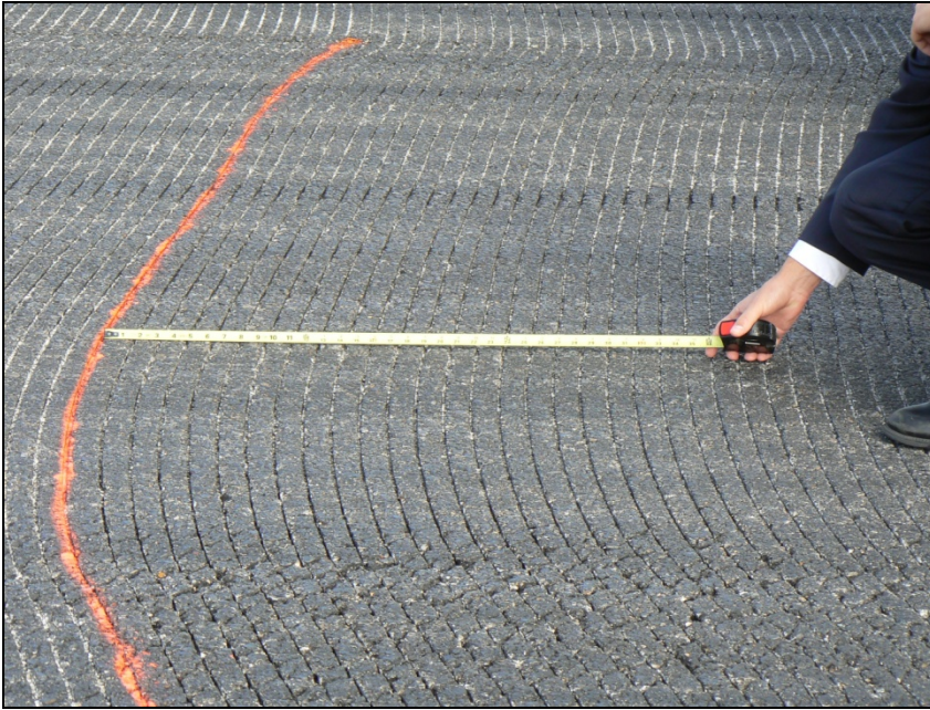
Figure 3-2. Shoving of Wearing Course on Runway 9-27
