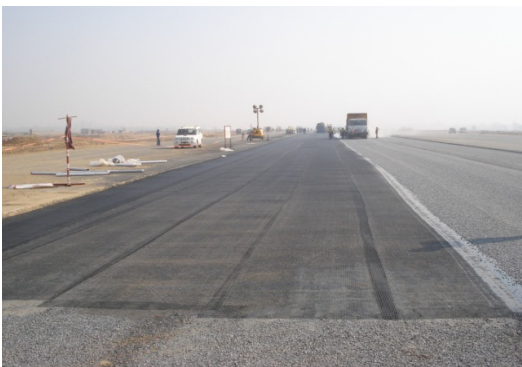
Figure 1-8. Imported glass grid Source: Delhi International Airport Limited (DIAL); reproduced with permission
