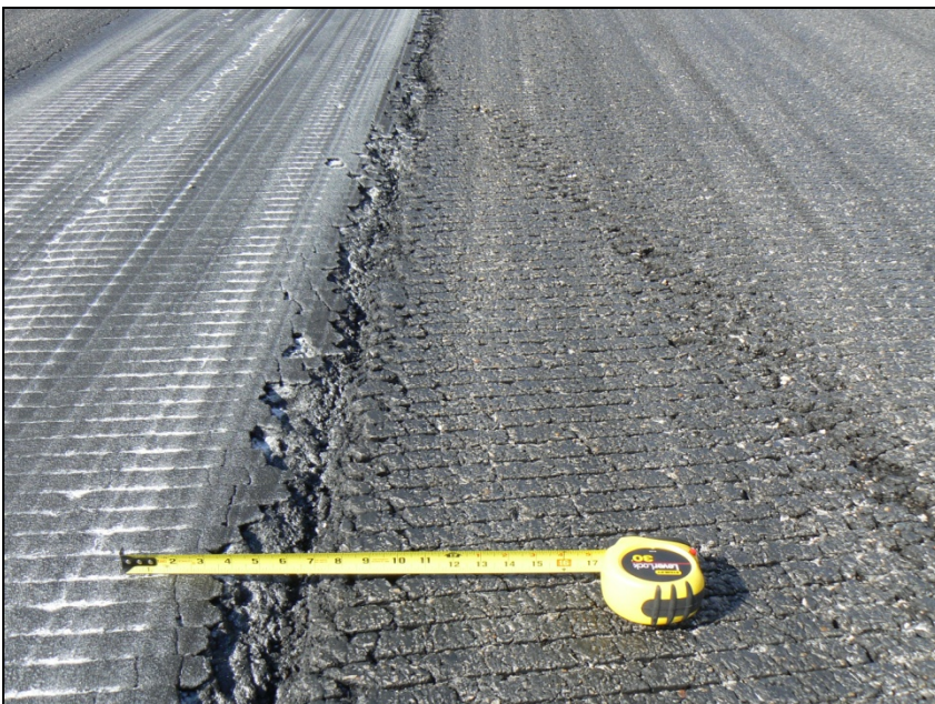
Figure 3-3. Longitudinal Fatigue Cracking of Wearing Course on Runway 9-27
