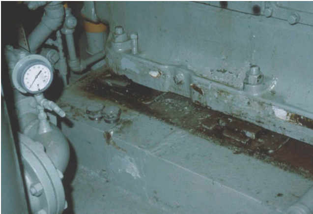
Figure 13.1 Steel chocks were the accepted method for setting large pieces of equipment. This has changed significantly with today's technology for machinery installation.
