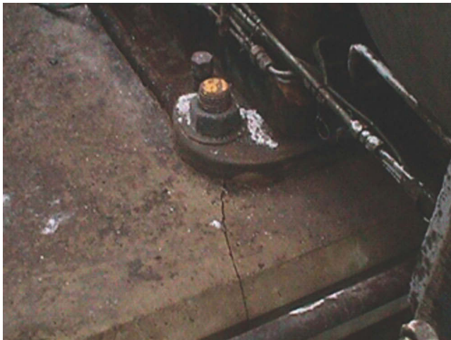
Figure 13.5 Grout crack from thermal growth or unwrapped anchor bolt.
