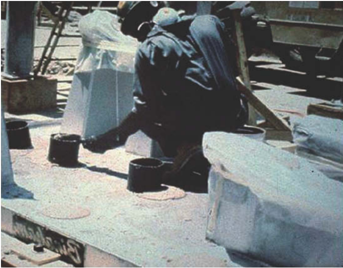
Figure 11.13 Utilizing PVC standpipes to maintain a constant head pressure on epoxy grout when utilizing a single-pour method on a pump baseplate.
