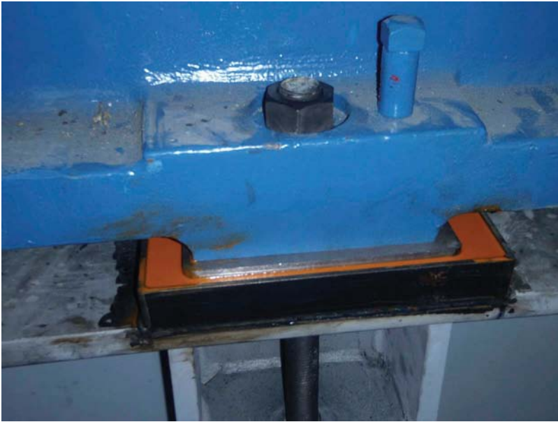
Figure 12.16 Once alignment is obtained the epoxy chocking compound is installed to secure the soleplate.
