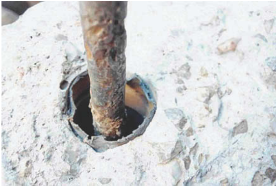
Figure 2.3 Severe bolt corrosion due to sleeves not being filled with a suitable filler.
