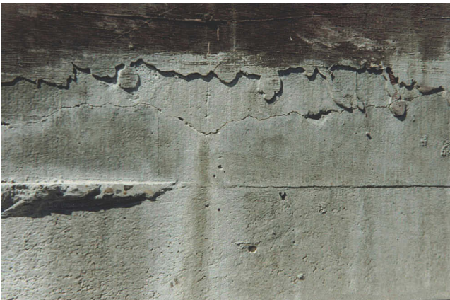
Figure 7.2 Edgelifting or curling cracks appear just at or slightly below the grout-to-concrete interface.
