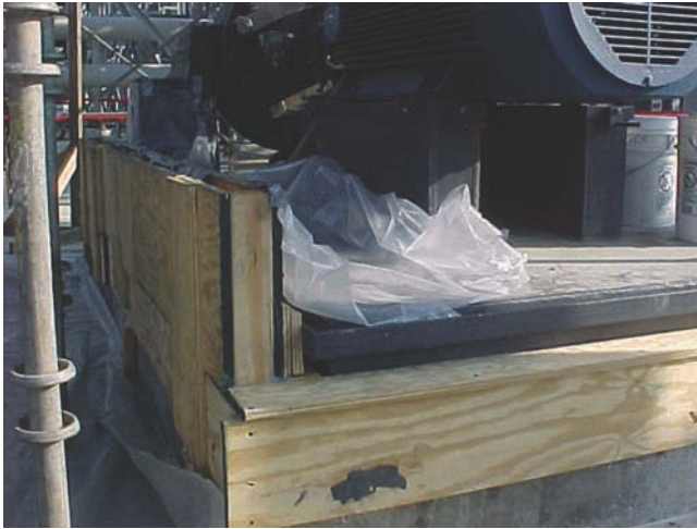
Figure 11.18 PregROUTed baseplate ready for field grouting. Note the head box incorporated into the form design to enhance flow.
