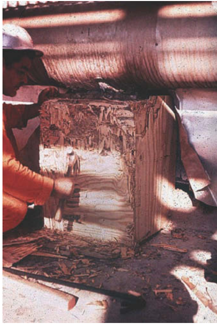
Figure 11.7 Failure to wax forms when using epoxy grout will result in excessive man hours for cleanup.
