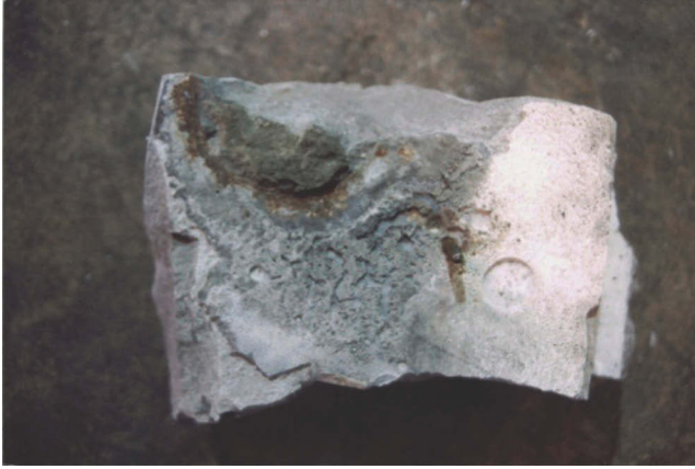
Figure 10.1 This piece of cement grout clearly shows that water trapped against the underside of the baseplate will cause voids.
