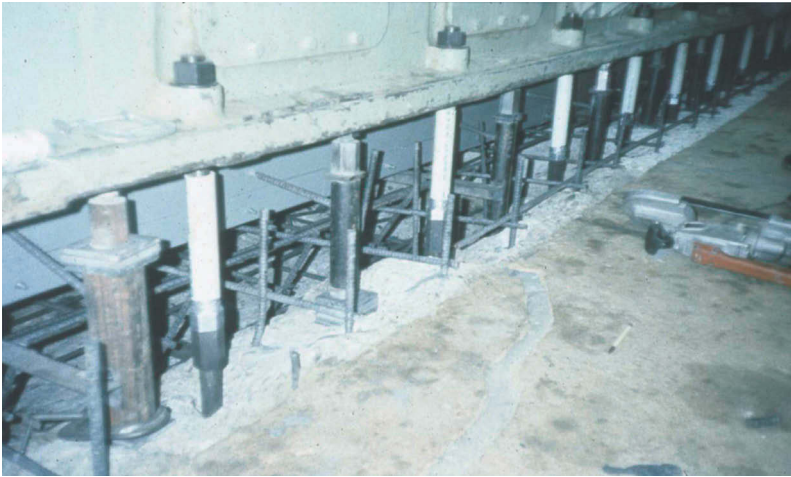
Figure 1.12 Machinery supported by supports fabricated from pipe.
