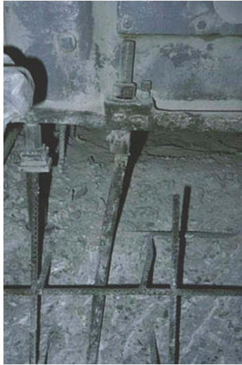
Figure 2.4 Noncustomer approved correction for a misaligned anchor bolt by the installing contractor.
