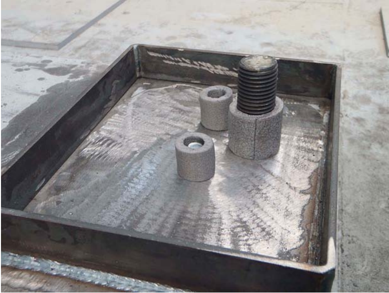
Figure 12.12 The epoxy chock is sized and the angle iron forms are welded to the skid around the anchor bolt. Soleplate jackscrews and the anchor are wrapped with pipe insulation to isolate them and prevent bonding of the chocking compound.
