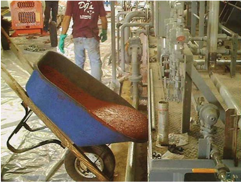
Figure 12.7 Grout placement may require more wheelbarrows than mixers since it may take longer to place than to mix.
