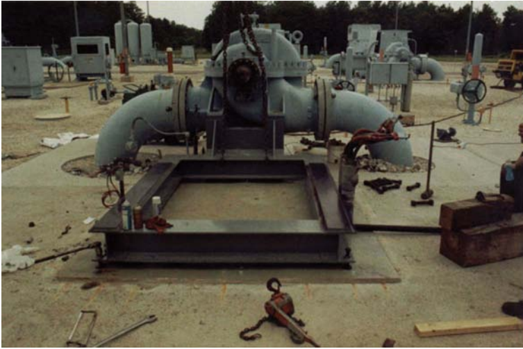
Figure 12.10 Set the pump and connect it to the piping prior to pouring chocks.
