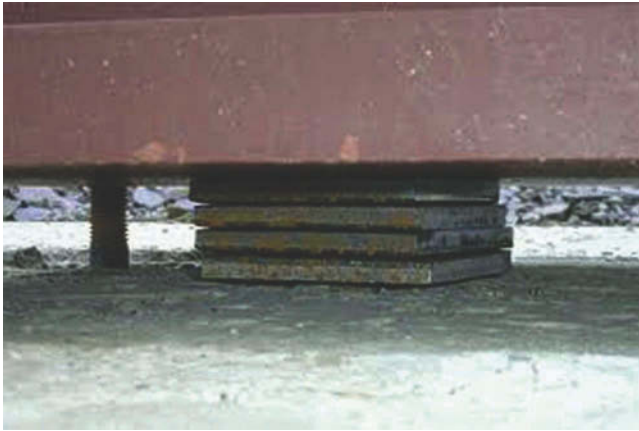
Figure 11.3 Using flat plates is not the best method for setting and leveling a baseplate. The grout will not support the baseplate.
