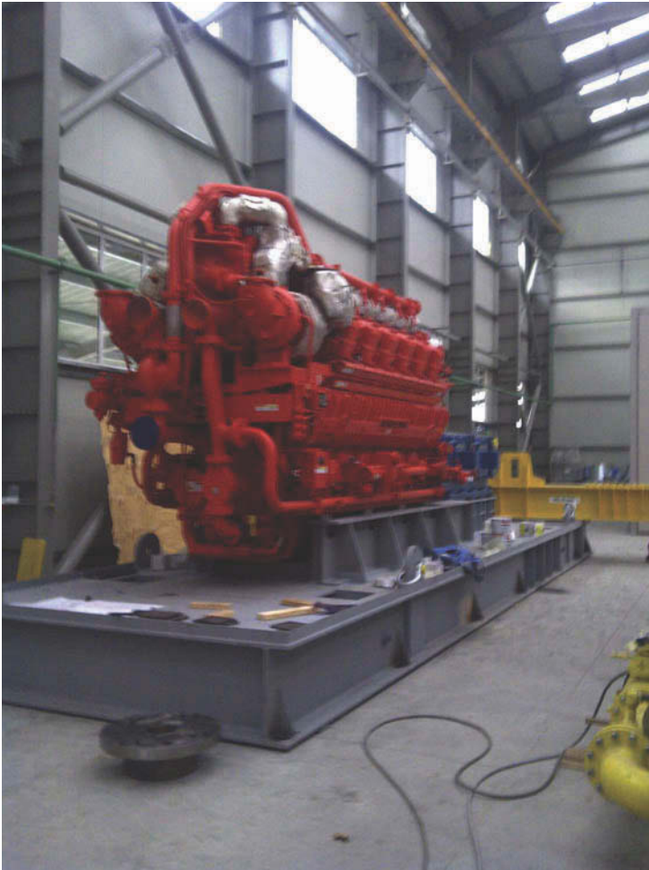
Figure 1.3 Skid-mounted compressor unit.
