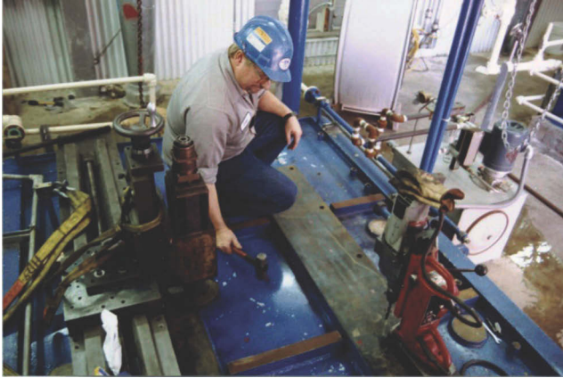
Figure 10.3 Gently tap around on the baseplate to locate void areas. Voids will have a hollow sound.
