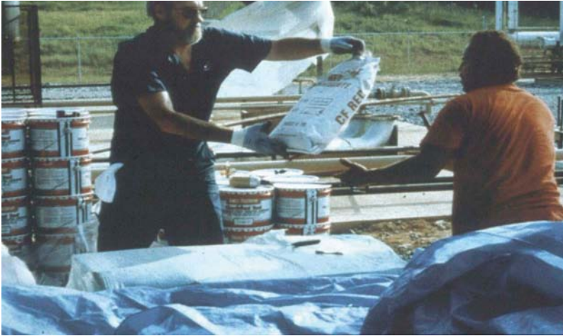
Figure 12.4 Have enough people at the job site to accomplish the various tasks associated with grout placement.
