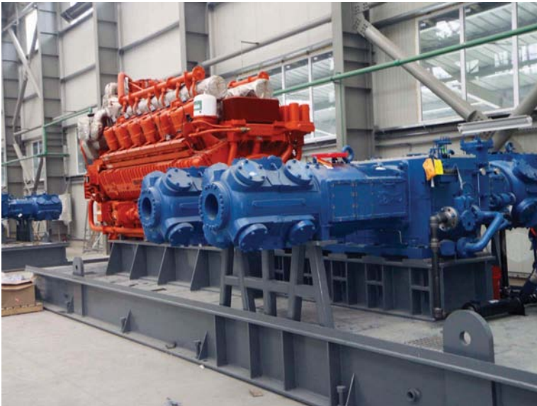
Figure 12.11 Skid-mounted engine driven compressor unit.
