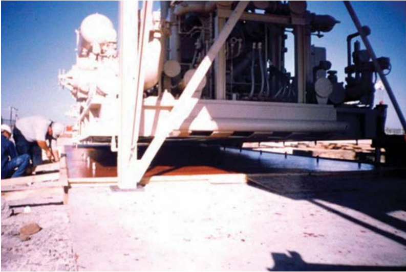
Figure 12.8 Pouring the grout and setting the skid will probably require some planning but is possible.
