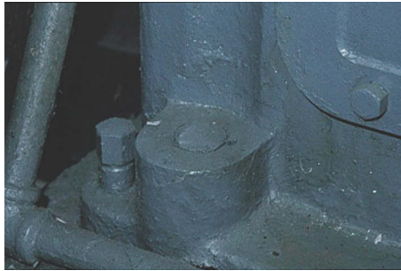
Figure 2.12 Nut only making contact on one side caused rapid failure at the thread root for this anchor bolt.
