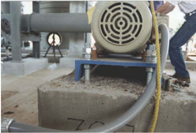
Figure 11.4 Mounting pumps this way shows a distinct lack of understanding about machinery installation.
