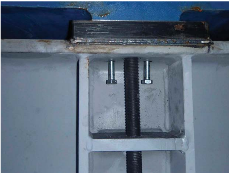
Figure 12.13 They are careful to allow enough free length to the anchor bolt to gain maximum clamping force.
