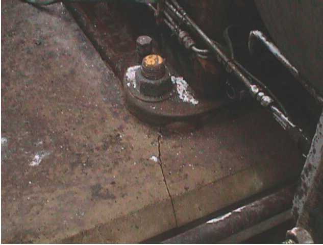
Figure 7.7 Cracking due to unwrapped anchor bolt.
