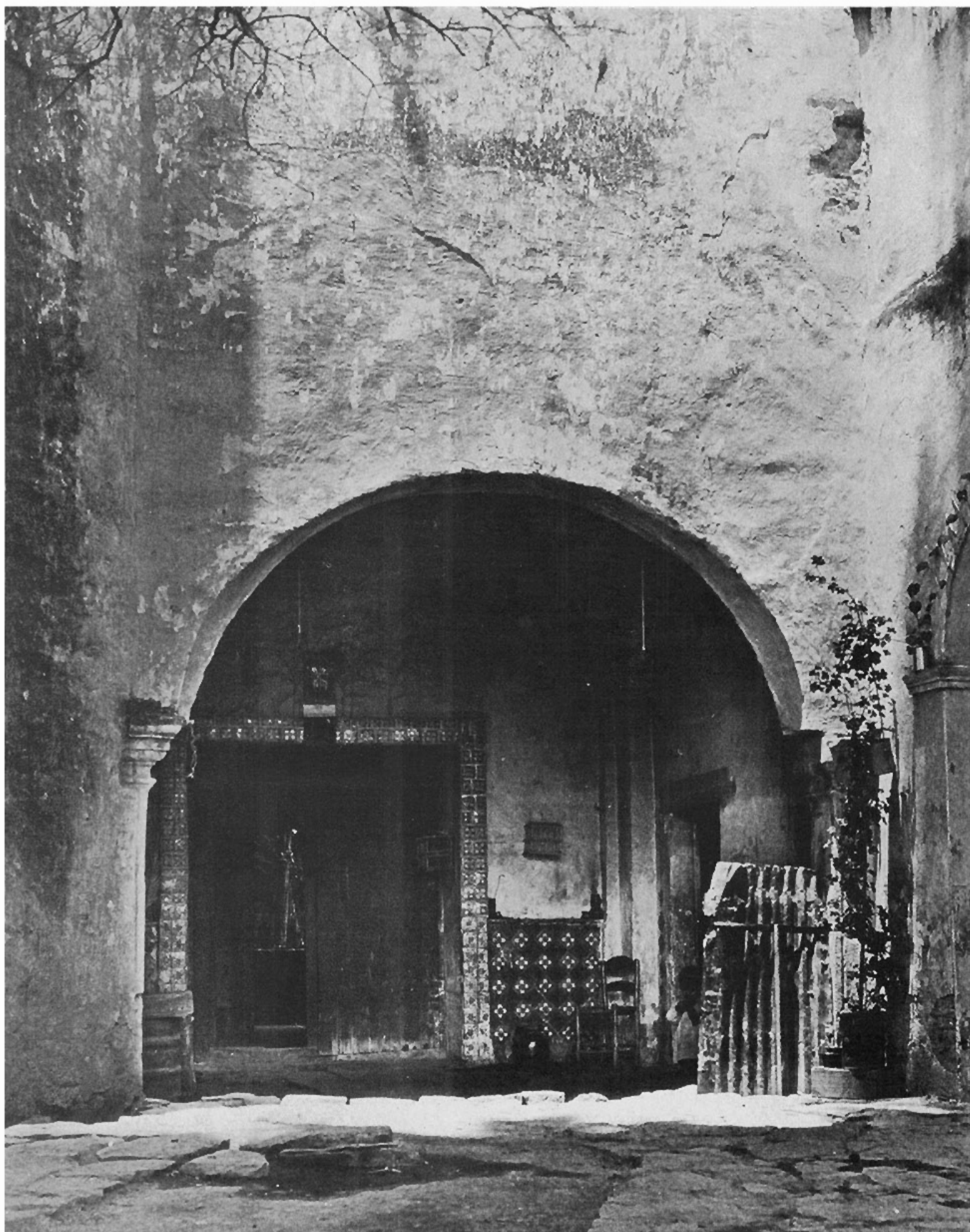
The arched entrance at San Antonio. The wall recently painted yellow, has scaled off in patches, showing grey blue and rose paint of former seasons. The tile trimmed door beyond leads to a garden patio
