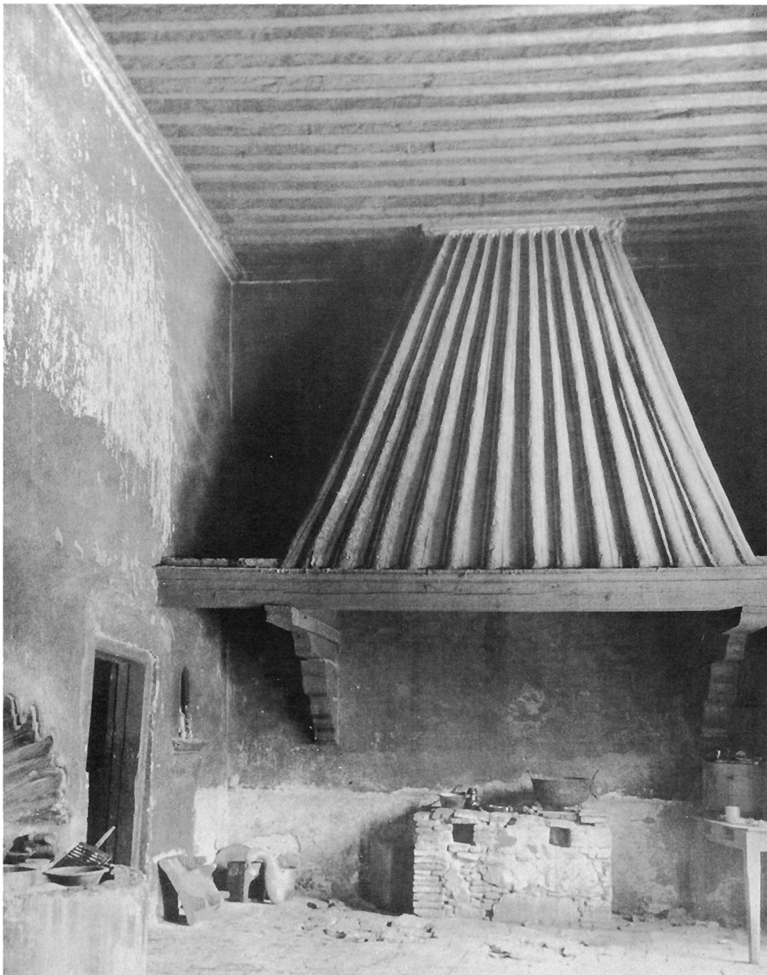
Kitchen in the Casa de los Condes de La Cadena at Apaseo. The brasero formerly extended across the entire end. Part of the stone sink with shell back shows on the left
