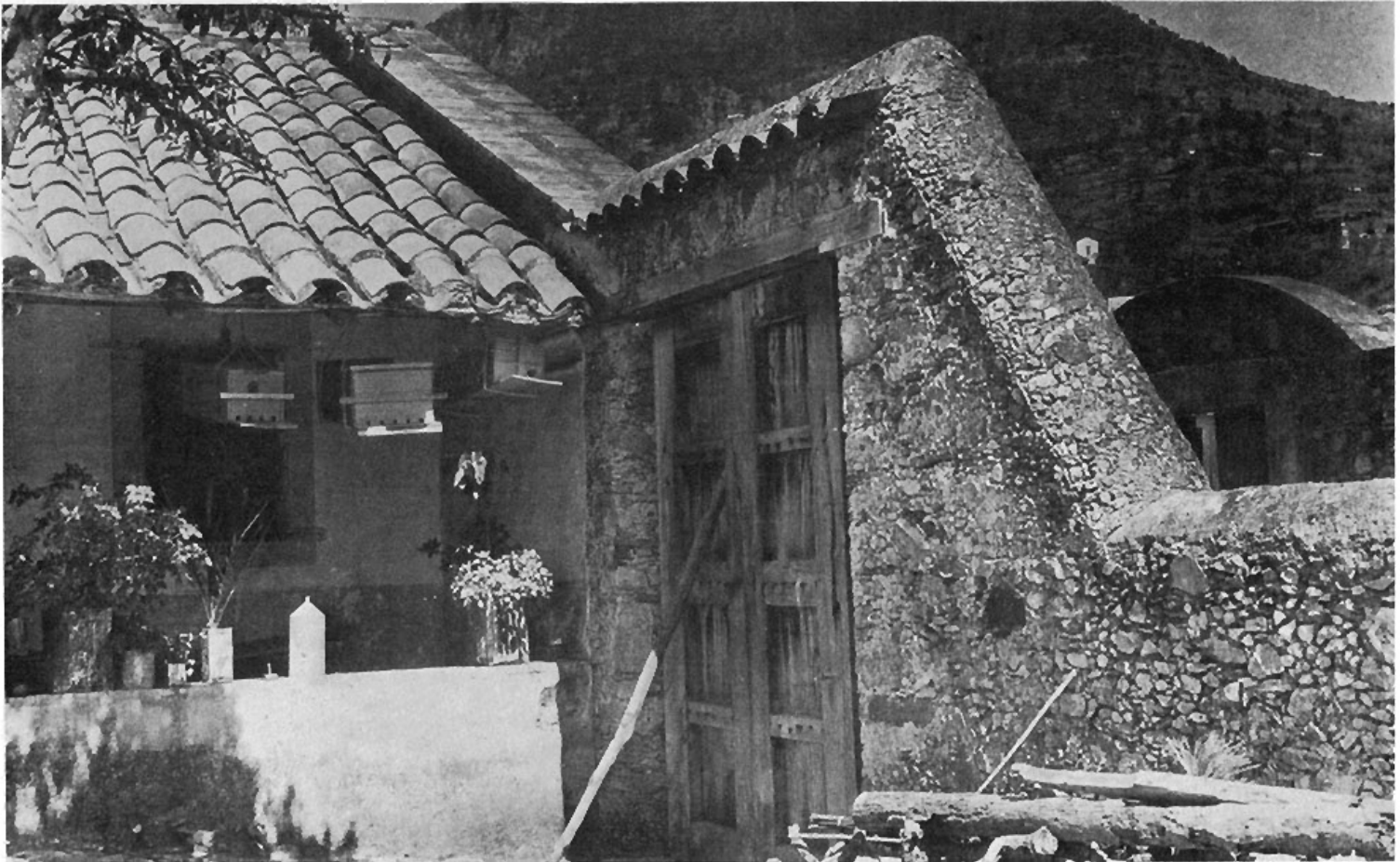
House of the Bees. Above. Interior view of the corridor. Under side of roof is left exposed. Floor of paving tile ten inches square. Below. Detail of wall treatment showing paving tile coping over end wall and roof tile drip over entrance
