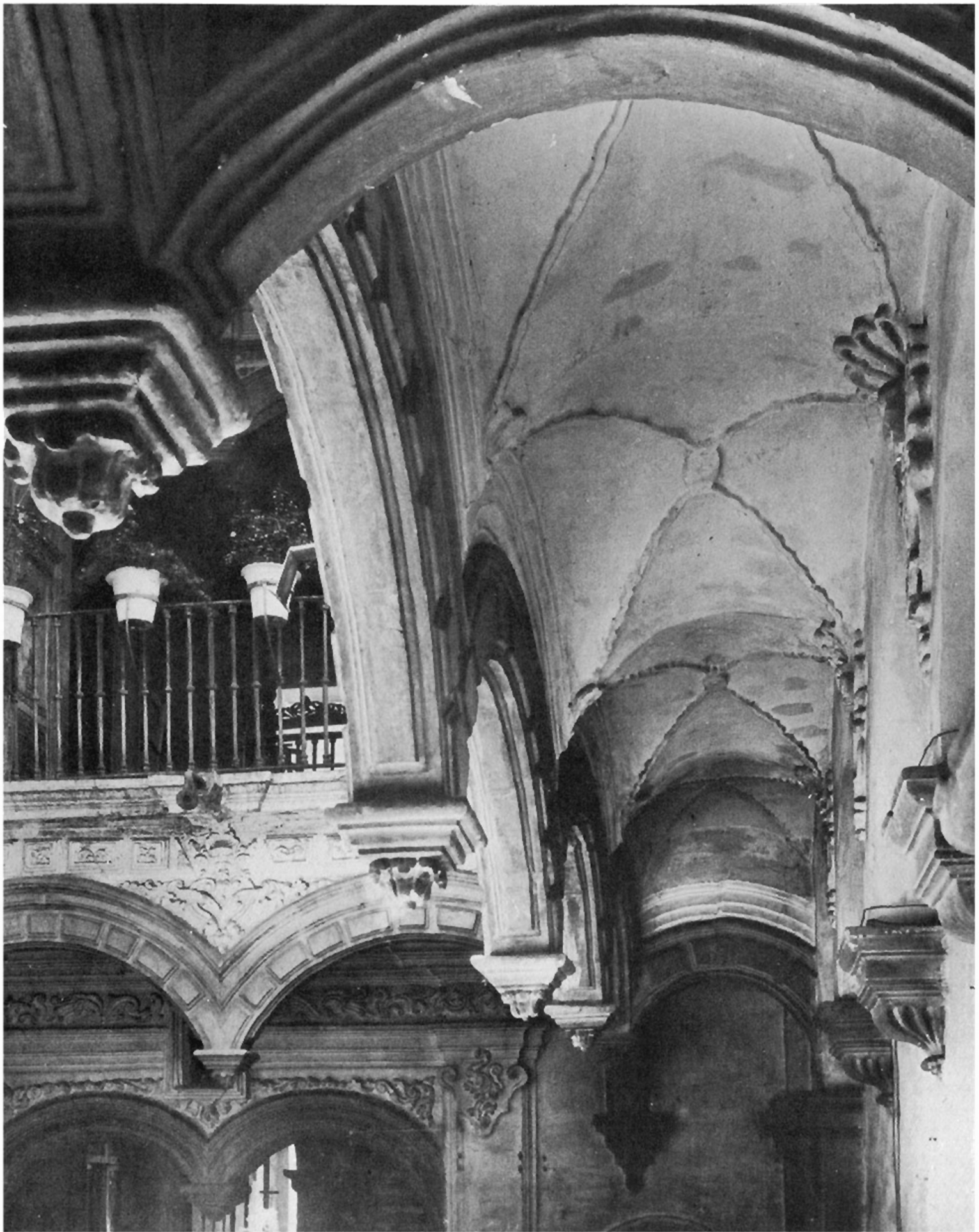
House of the Marquesa de Uluapa. Detail of the main patio, looking toward the rear from the entre suelo or mezzanine level, showing the arches which support the main floor corridors. The stone of the apparently unsupported arches is so cut that the thrust carries through from wall to wall
