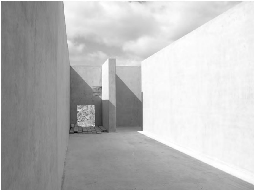
Figure 1.2 A concrete tank (before construction of the roof) illustrating the simplicity of the structural form (Photo: M.J. Kirby).
