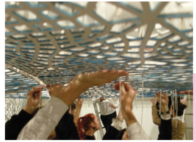
ABOVE: Laser-cut panels, test mock-up, installation. BELOW: Panel-cutting templates. BOTTOM: Details showing converging pattern. Photos: Brennan Buck
