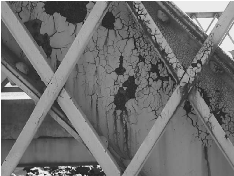
FIGURE 9.16 Blistering and peeling of protective coating subjected to regular deicing salt application.
