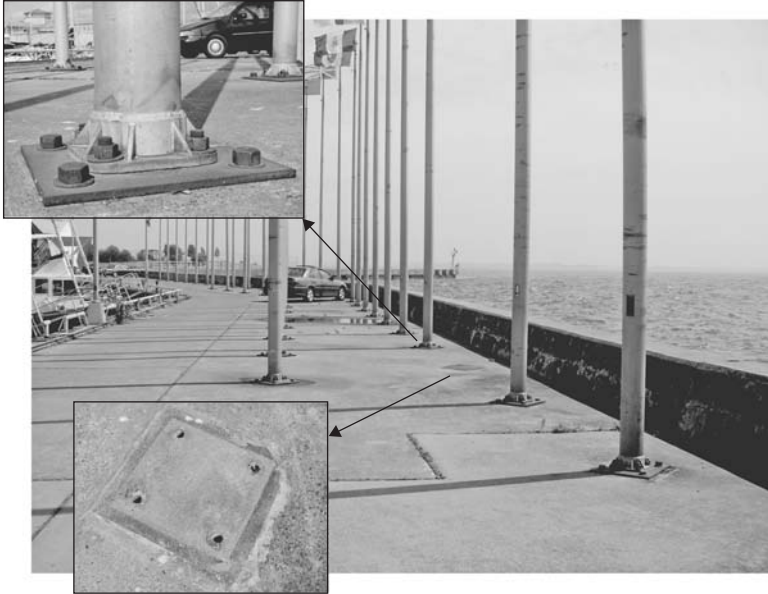
FIGURE 11.18 Steel flag posts with steel base sitting on concrete with close-ups of pack rust area and missing post due to corrosion of the base.
