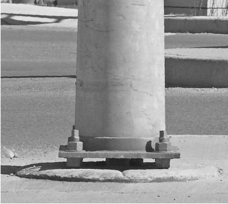
FIGURE 11.20 Lamppost galvanized steel base with a gap over the concrete to prevent crevice corrosion and pack rust.
