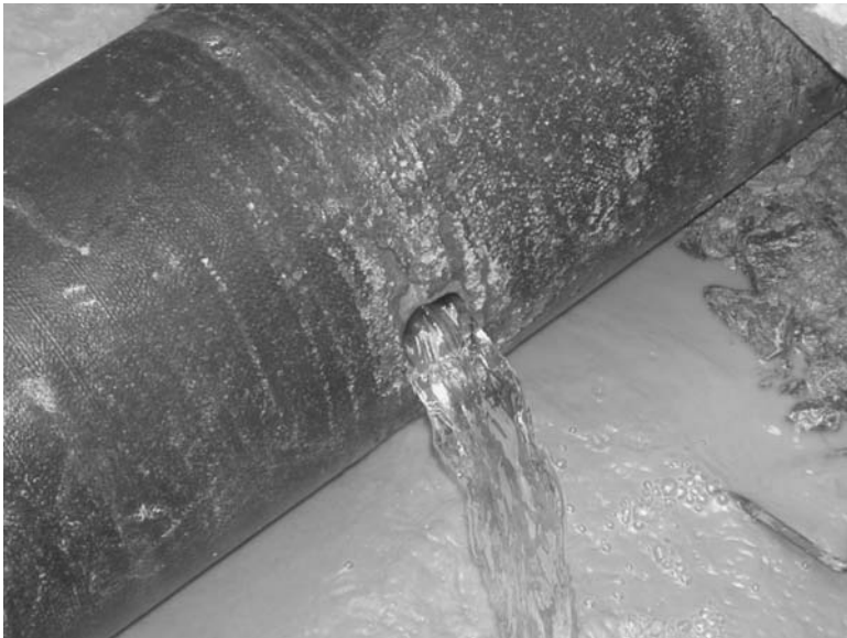
FIGURE 10.5 A corrosion pit that led to the perforation and leak of a water main. (Courtesy of Drinking Water Services, City of Ottawa)
