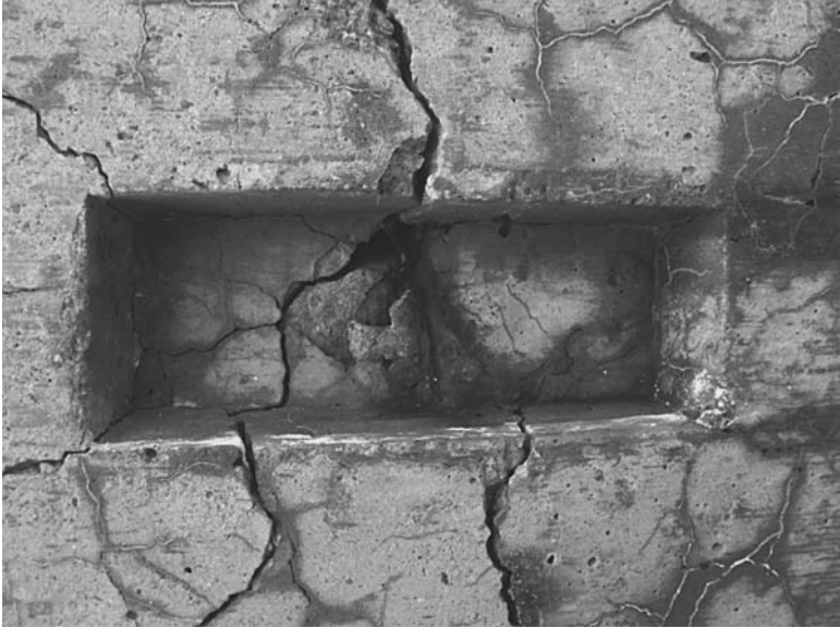
FIGURE 7.24 Cracking of concrete cover in marine environment.
