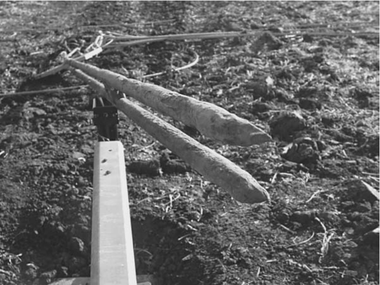
FIGURE 7.15 Anchor assembly cut by corrosion at the concrete anchorage. (Courtesy of Anchor Guard)
