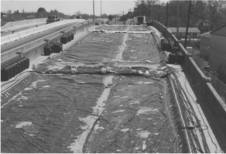
FIGURE 5.46 Bridge deck energized for electrochemical chloride extraction. (Courtesy of Vector Corrosion Technologies)
