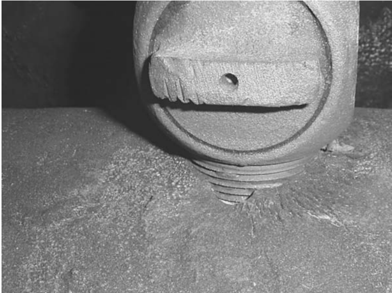
FIGURE 7.21 Corrosion of a water main ductile iron adjacent to a copper fitting. (Courtesy of Drinking Water Services, City of Ottawa)
