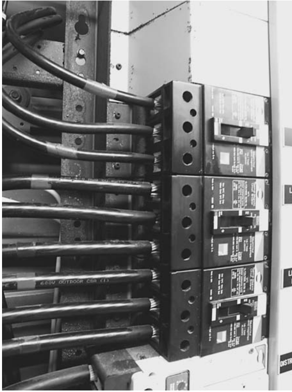
FIGURE 9.5 Electric junction box badly corroded only four years after a new residence was completed. (Courtesy of Kingston Technical Software)
