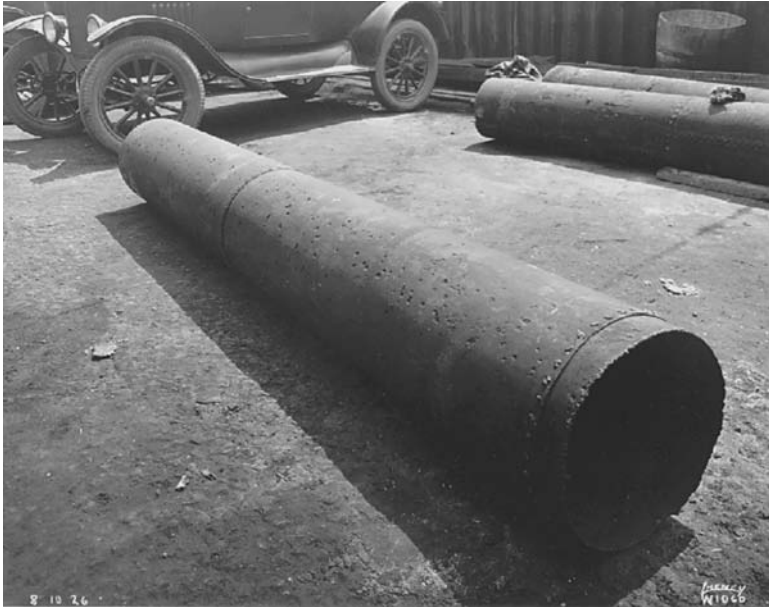
FIGURE 7.5 Pits in 16-inch sheet iron water main in San Francisco's East Bay that failed in one month due to leakage of current from electric streetcars. (Photo dated August 10, 1926, Courtesy of East Bay Municipal Utility District).
