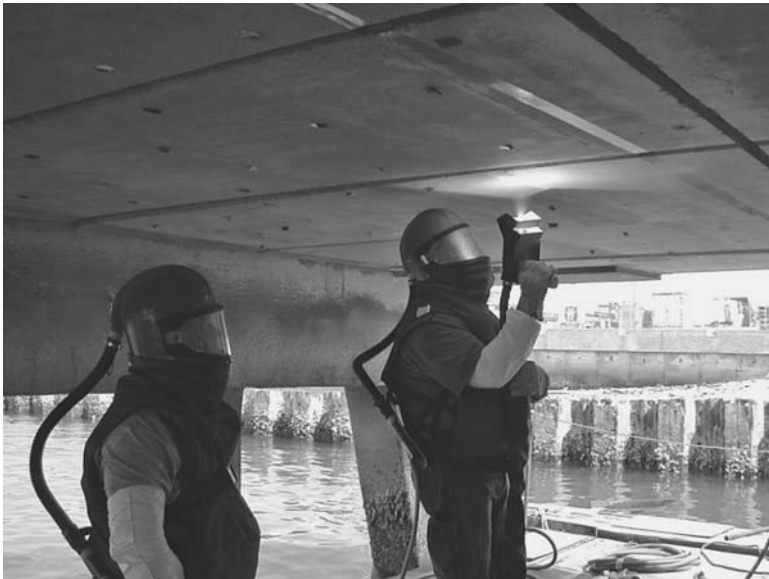
FIGURE 13.21 Application of activated arc sprayed zinc on a reinforced concrete structure. (Courtesy of Vector Corrosion Technologies)
