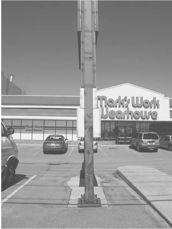
FIGURE 9.21 Decreasing corrosion of a sign post as a function of height.
