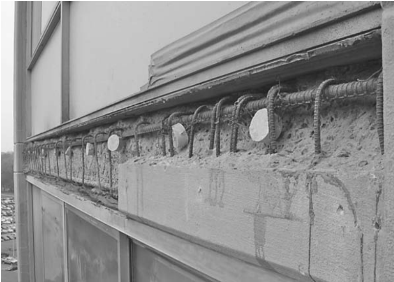
FIGURE 13.23 Embedded zinc anodes used in concrete rehabilitation to prevent the formation of new corrosion sites adjacent to completed patch repairs. (Courtesy of Vector Corrosion Technologies)
