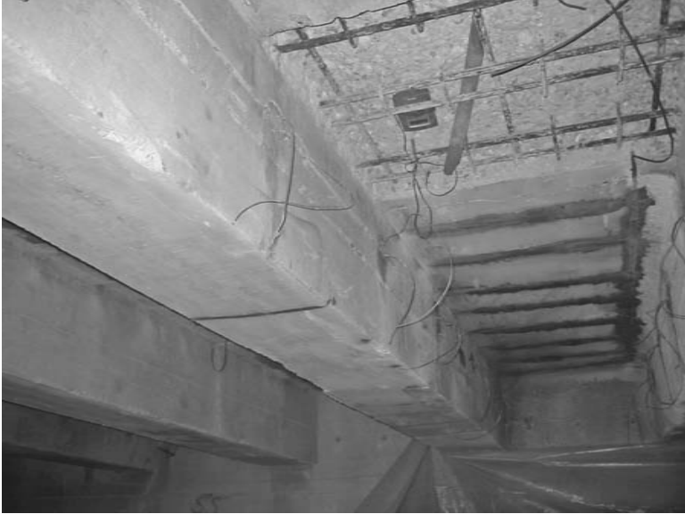
FIGURE 13.20 Impressed current cathodic protection being retrofitted on an old bridge structure: note vent tubes and drill holes anodes. (Courtesy of Vector Corrosion Technologies)
