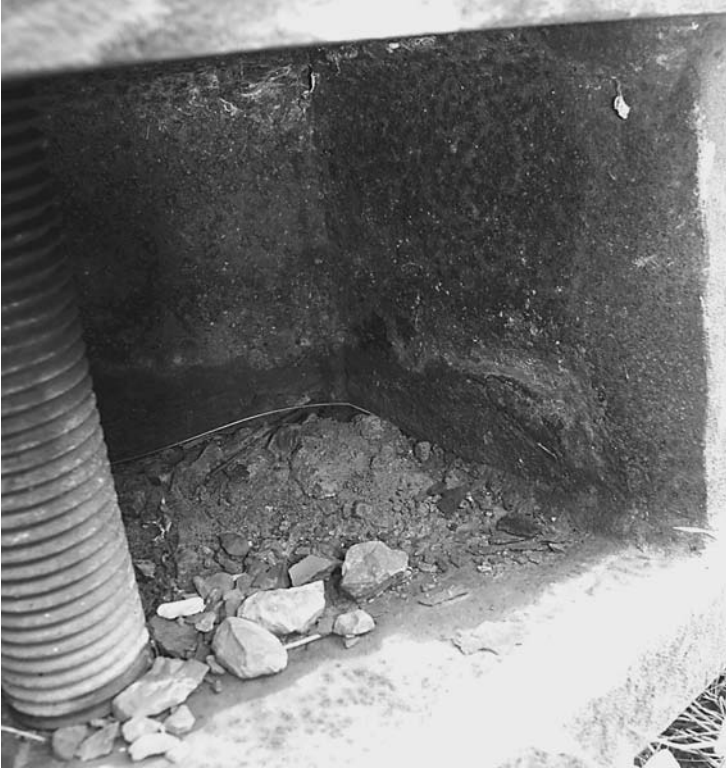
FIGURE 9.46 Pack rust developing at the base of the weathering steel highway lamppost shown in Fig. 9.45, only 15 years after its installation.
