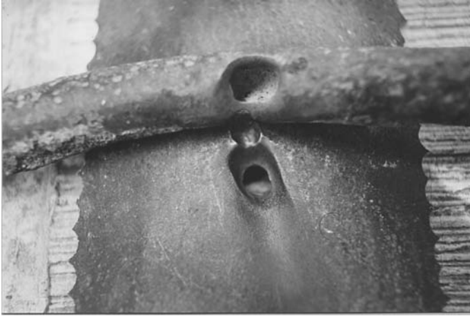
FIGURE 6.9 Pits in the galvanized water pipe that contributed to the erosion-corrosion of the gas line and the subsequent leak in a sewer main that caused the Guadalajara 1992 explosion [6]. (Courtesy of Dr. Jose M. Malo, Electric Research Institute, Mexico)
