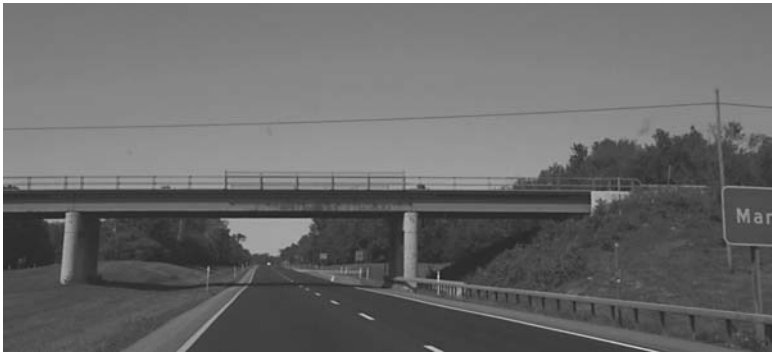
FIGURE 9.22 Corroded overpass steel bridge above the most traveled lane of a two-lane highway, a telltale symptom of deicing salt corrosion.
