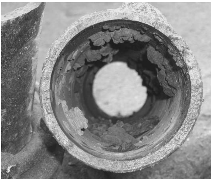
FIGURE 6.10 Corrosion products forming nodules or tubercles over pit cavities. (Courtesy of Drinking Water Services, City of Ottawa)
