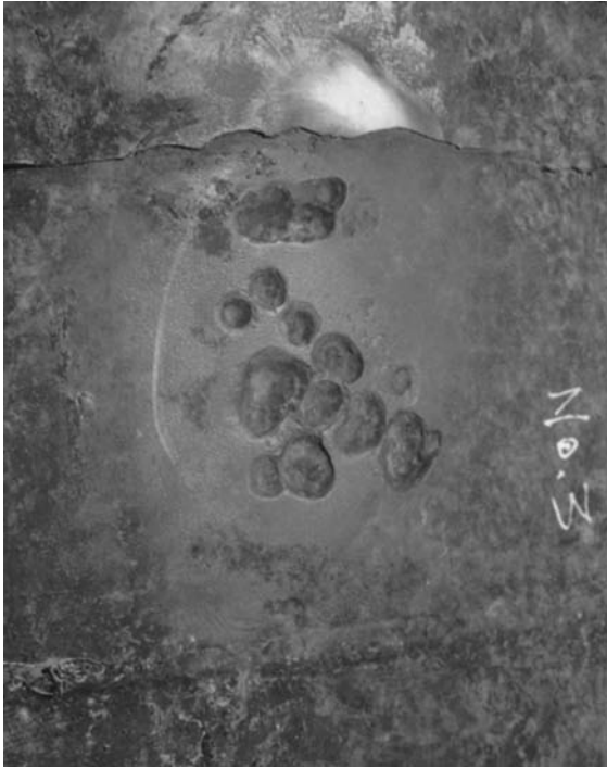
FIGURE 10.3 Typically deep, sharp-sided pits usually found under disbonded coatings or hard accumulations on a pipe surface. When disturbed the area may smell of hydrogen sulfide, a telling sign of microbial activity. (Courtesy of MACAW's Pipeline Defects, published by Yellow Pencil Marketing Co.)
