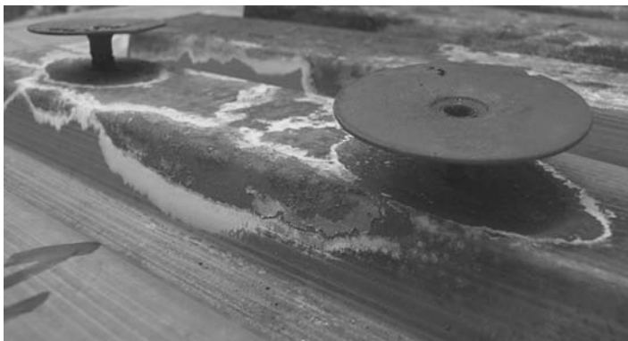
FIGURE 6.25 Section of galvanized roof panel after five years under PFRI.
