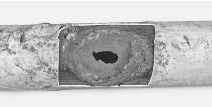
FIGURE 13.34 Pipeline perforated by a large fault current. (Courtesy of MACAW's Pipeline Defects, published by Yellow Pencil Marketing Co)
