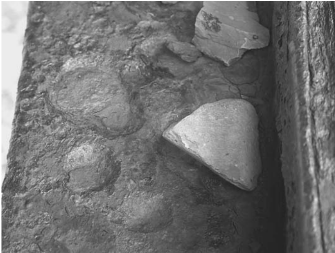
FIGURE 6.20 Large holes created in a bridge structural steel by the presence of rocks. (Courtesy Kingston Technical Software)
