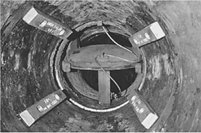
FIGURE 13.5 Sacrificial zinc anodes on the interior wall of a drydock water handling pipe. (Courtesy of Defence R&D Canada-Atlantic)
