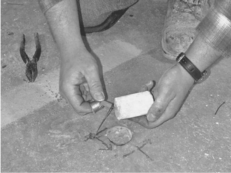
FIGURE 13.22 Zinc anode being connected to the rebar structure to control on-going corrosion and prevent the initiation of new corrosion activity in concrete structures. (Courtesy of Vector Corrosion Technologies)
