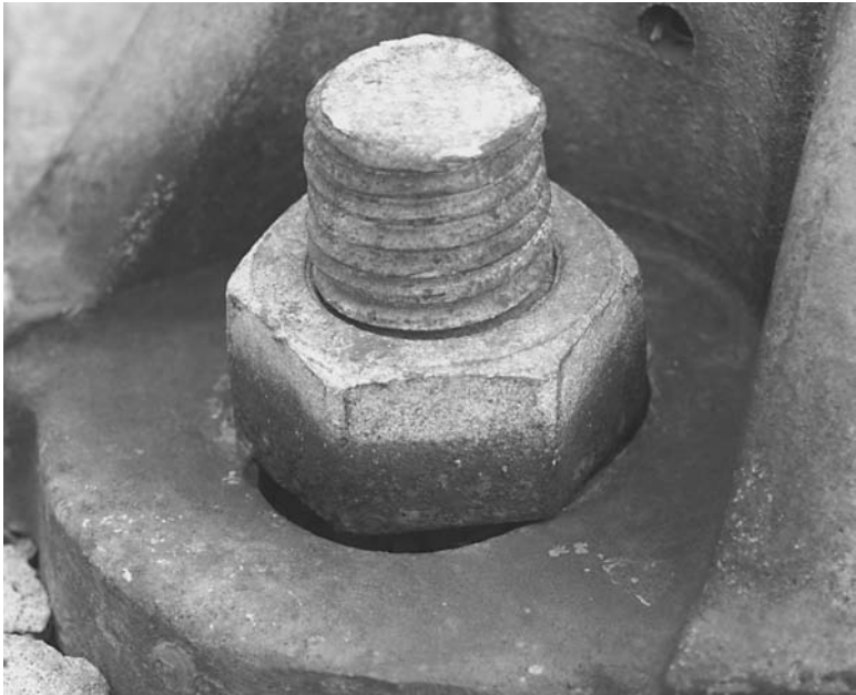
FIGURE 9.6 Galvanized bolting assembly after 10 years of exposure to a deicing salt environment.
