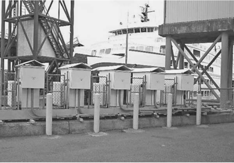
FIGURE 13.28 Five 300 ampere marine oil cooled rectifiers supported by an automatic dewatering oil spill containment pan. (Courtesy of Dean Rookes, West Coast Corrosion Prevention Ltd.)
