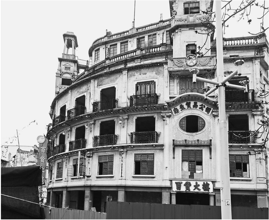
Plate 6.5 The dilapidated city center of Shantou. The old city center is located in the 'little park' ( xiaogongyuan ). The population moved very fast towards the new areas in the special economic zone, leading to population decline in the central area. This is rare in China, because the development of suburbs usually coexists with a prosperous city center, which remains an attractive location. The Chinese suburbanization process is in contrast to strong nostalgia for the countryside in Britain or white flight and inner city decline in the U.S.
