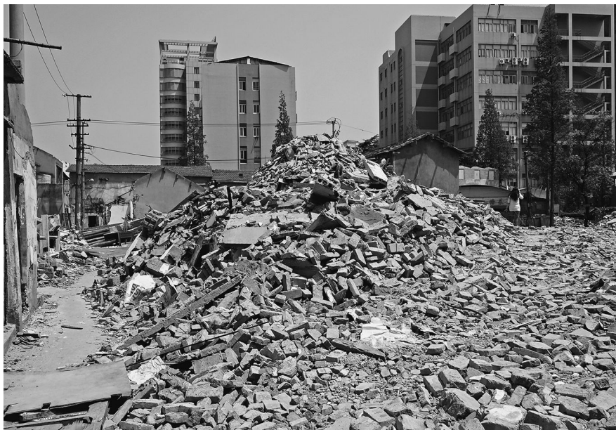
Plate 7.4 The demolition of an informal settlement that accommodated rural migrants in Shanghai. The neighborhood has been demolished, and the space is becoming part of the Caohejin High-tech Park. The redevelopment, however, is not for instant land profit. The new space is used for office buildings, which generate long-term business taxes for the local government.
