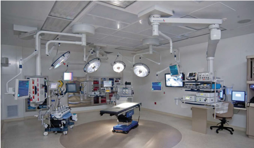
Fig. 4.124 National Heart Centre, Singapore—Operating theatres 3—Integrating advances in medical technology within the operating theatre environment in a way that supports staff while enhancing the patient's healing process is a key design priority for any new solutions: high definition solutions include seamless connection of cameras, video switching, audio-visual infrastructure, media storage and high definition video conferencing ( Source Broadway Malyan Singapore 2012)
