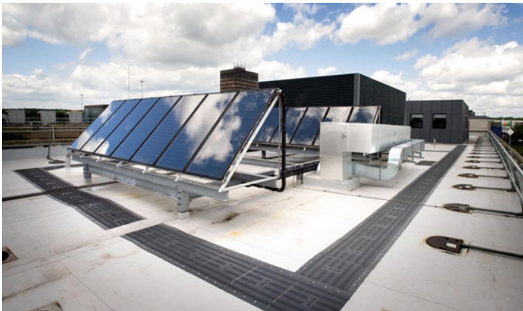
Fig. 4.36 Houghton Le Spring Primary Care Centre—Roof-mounted solar pre-heater arrays (Source P + HS Architects 2012). Advantages of building-integrated PV are enhancement of building appearance, solar gain control, thermal insulation, roof or façade material replacement, passive ventilation and electricity generation
