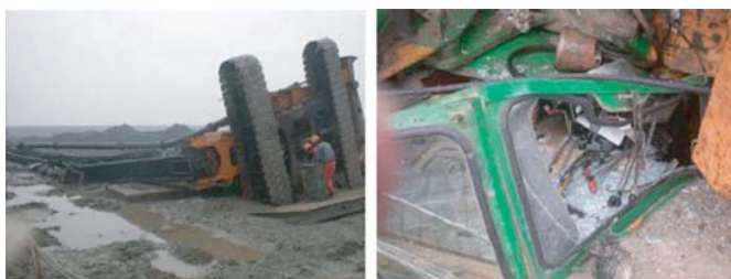
Fallen pile-driving rig
