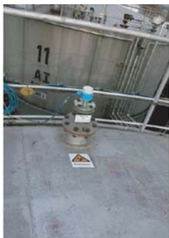
Level gauge on top of tank
