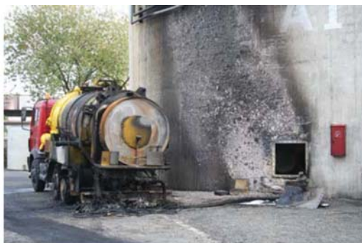
Destroyed truck and fire damage on concrete bund wall
