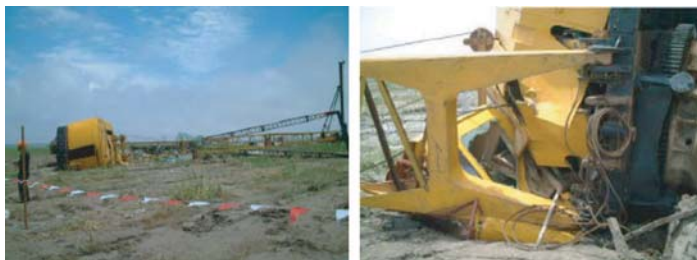
Overturned crane at construction site
