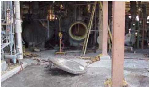
The cover plate blew off this polymer catch tank, killing three workers
