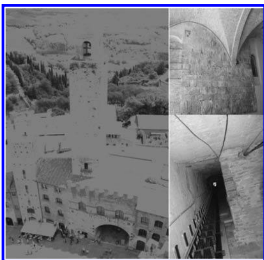
Figure 1. The “Rognosa” tower in San Gimignano, general view (left), some vaults bearing down on the tower (top right), the interior of the tower (bottom right).
