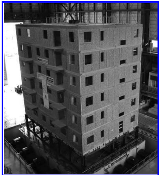
Figure 1. The NEESWood Capstone test building ready for testing at the worlds' largest shake table in Miki, Japan in July 2009. The building represents the largest building ever tested on a shake table.
