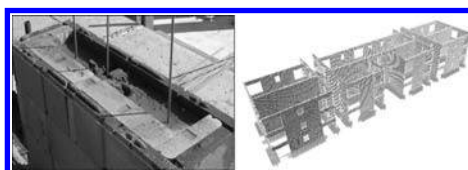
Figure 1. (a) Formwork blocks filled with concrete; (b) model of the torsionally-unbalanced building.
