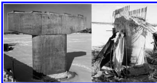
Figure 1. Bridge Pier Cap Failure.
