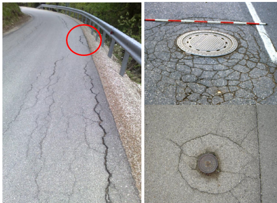
Fig. 2. Longitudinal edge cracks at the edge of the pavements (left) and circular shaped cracks at the shafts (right)
