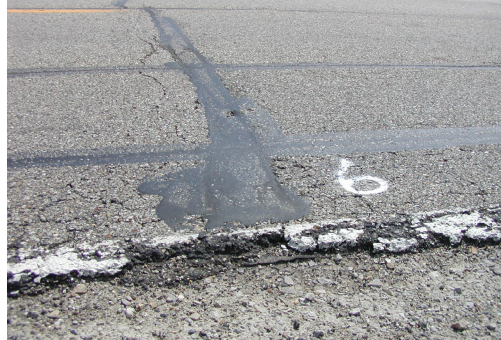
Fig. 1. Band-type reflective cracking on US 136 near Peoria, IL
