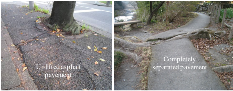
Fig. 1. Damage to asphaltic pavement caused by the growth and thickening of plant roots
