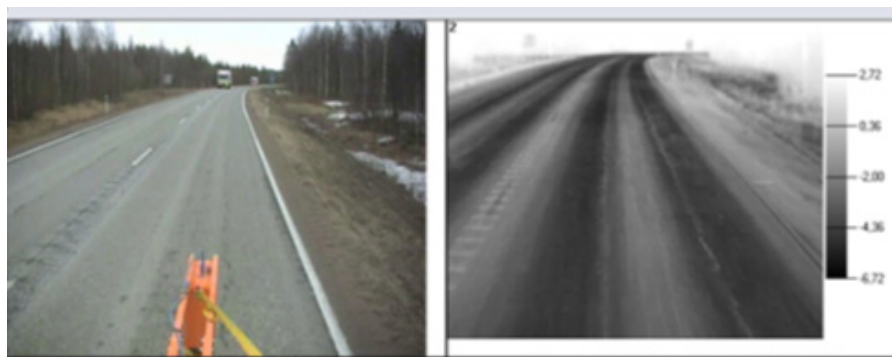
Fig. 6. Example of top down cracking and water being pumped through the pavement by heavy vehicle loading.
