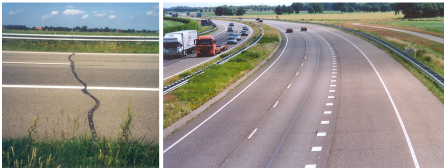
Fig. 1. Typical reflective cracking on a cement treated base (left) and concrete slabs (right)
