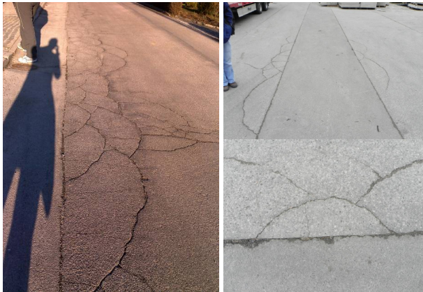
Fig. 1. Semi-circular shaped cracks at the edges of the pavements (left) and excavations (right)
