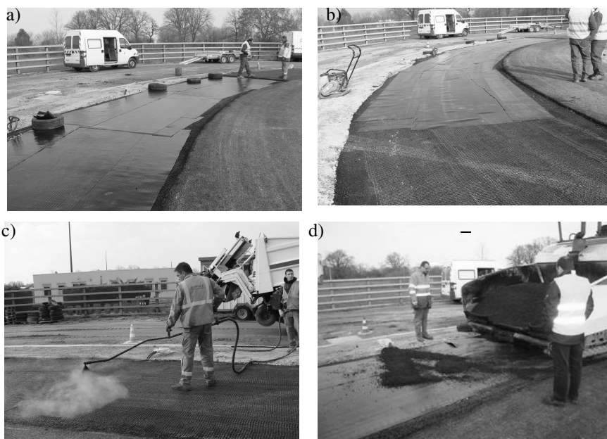
Fig. 2. Construction: a) Grids of section A and B ; b) Grids after compaction; c) Tack coat application; d) Placement of strain gauges before overlay
