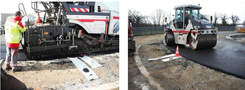
Fig. 7. Pouring asphalt concrete on top of the sensor enabled geotextile strips (left) and compaction (right)
