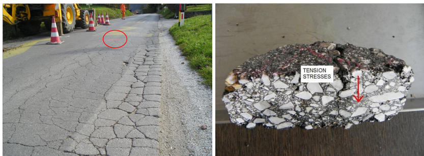
Fig. 5. The location of asphalt core taken on semi-circular shaped cracks (left) and presentation of semi-circular shaped cracks propagated top to bottom through the cross section (right)
