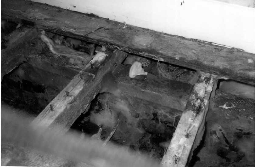
Figure 4.10 Ground floor joists attacked by cellar fungus – coniophora puteana (photo courtesy of Bob Caille)
