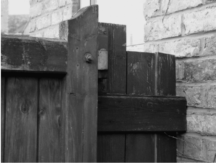
Figure 7.5 Exterior stain finish showing some erosion – but no peeling or flaking
