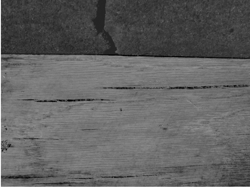
Figure 4.2 Cracking in skirting caused by over-drying in situ
