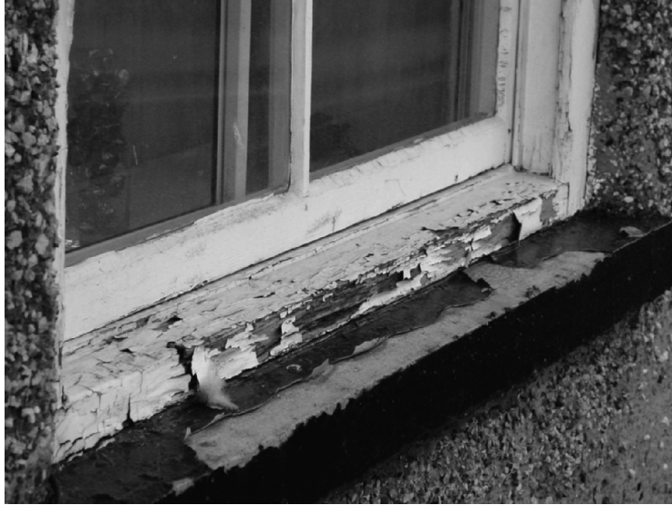
Figure 7.4 Failure of film-forming exterior paint by peeling and flaking
