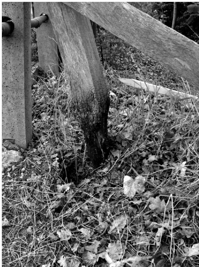
Figure 4.9 Post rotten at the ground line
