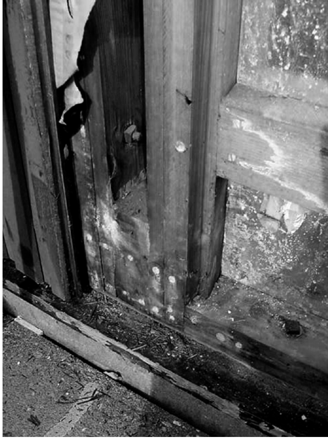
Figure 4.4 Studs and rails in a timber frame wall – possibly at risk from interstitial condensation
