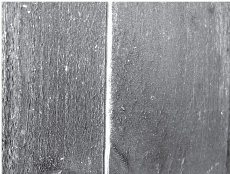
Figure 7.7 Shrinkage on dark-stained boards showing paler joints
