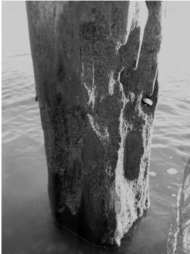
Figure 4.11 Pile attacked by limnoria (gribble) (photo courtesy of Simon Cragg)
