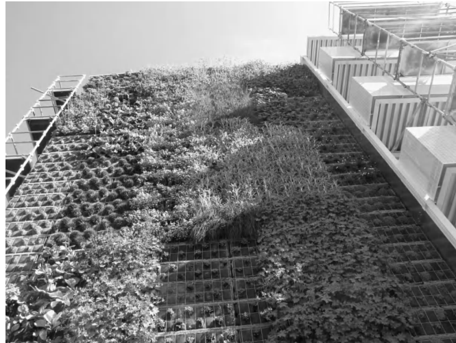
Figure 7.1. Living wall in Nantes (France) with different varieties of plants, and a heterogeneous shading effect
