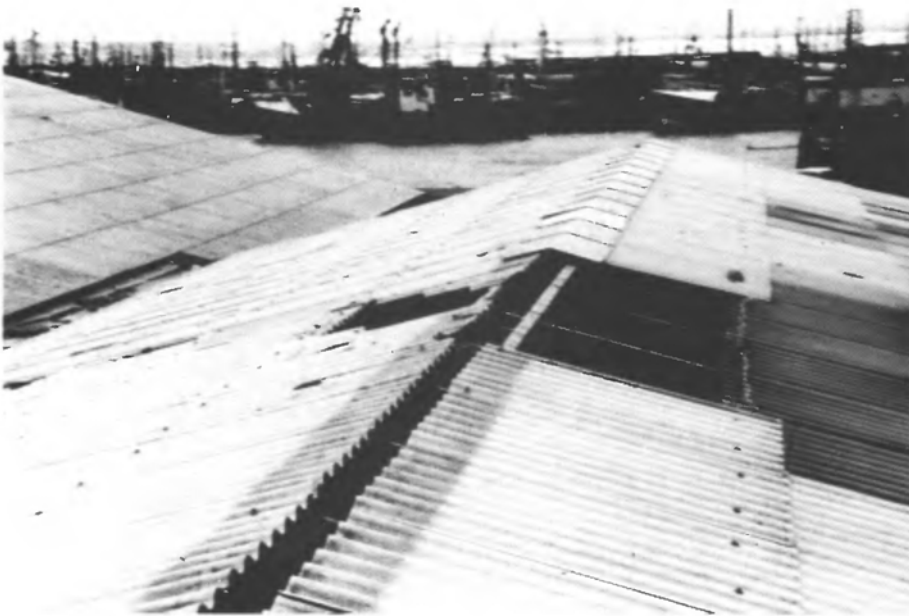
Fig. 4.6 When the wind blows perpendicular to the longitudinal direction of the building, the ridge is prone to a considerable amount of suction. (Reproduced by permission of Danish Building Research Institute. Photo: H.H. Knutsson).
