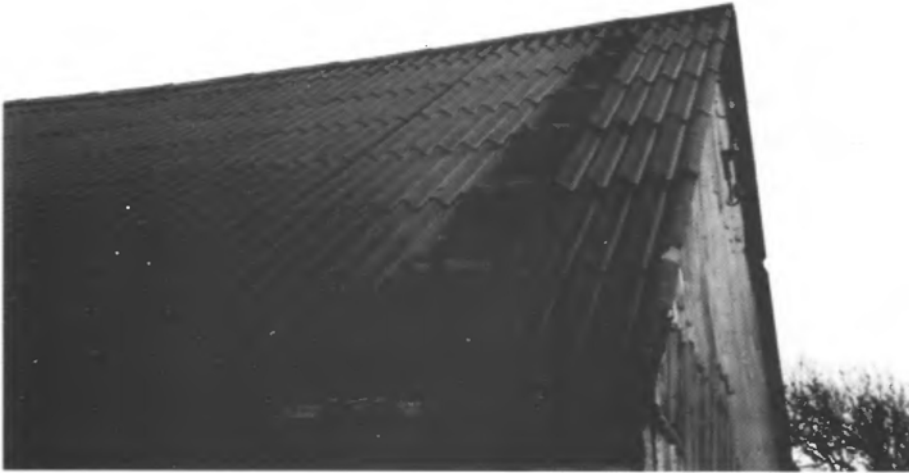
Fig. 4.5 When the wind blows along the building, the foremost part of the roof is subjected to considerable suction. (Reproduced by permission of Danish Building Research Institute. Photo: H.H. Knutsson).
