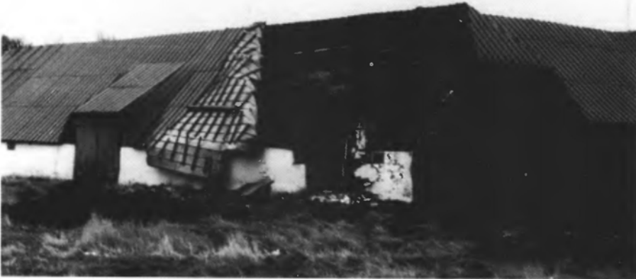
Fig. 4.7 When the wind approaches the gable, the roof at the corner is worst hit by suction. (Reproduced by permission of Danish Building Research Institute. Photo: H.H. Knutsson).
