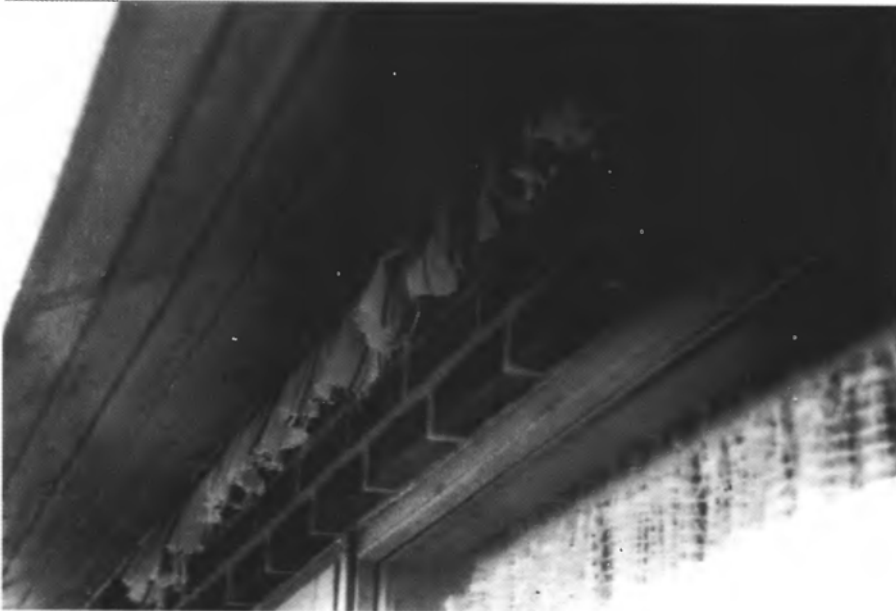
Fig. 4.8 Suction lifted the roof off entirely and the curtain was sucked out before the roof settled back in position. This could have been avoided if the roof had been properly anchored. (Reproduced by permission of Danish Building Research Institute. Photo: H.H. Knutsson).
