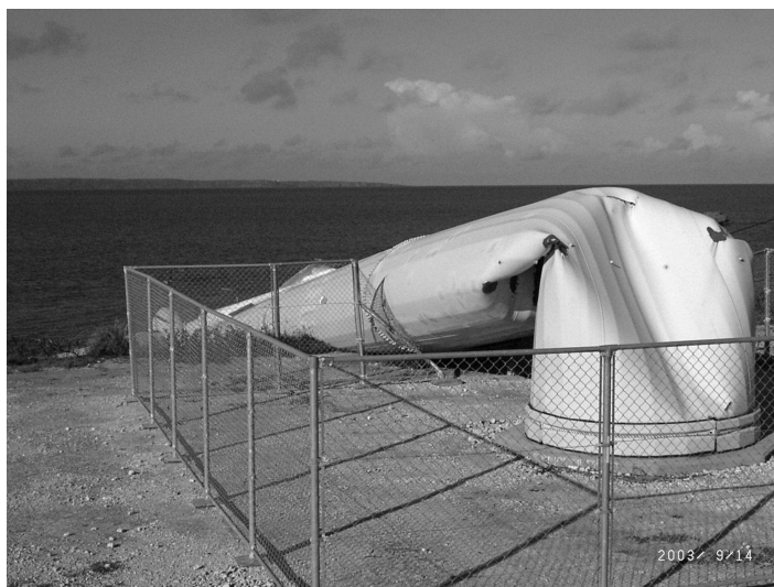
Figure 11.6 A failed wind turbine tower following a typhoon. (Picture by Dr. M. Matsui, Tokyo Polytechnic University. With permission.)
