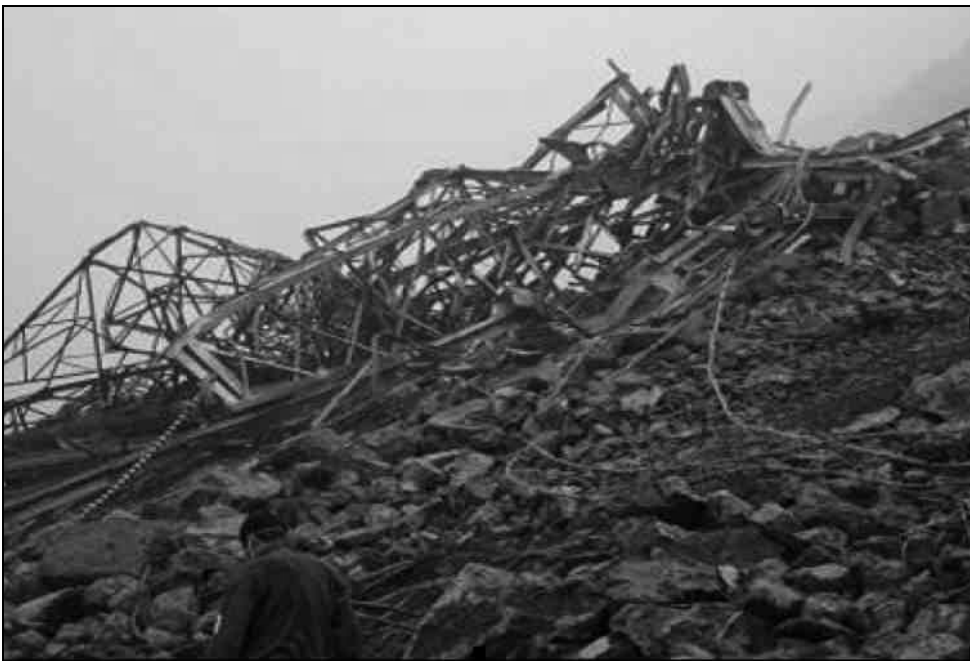
Fig. 4.65. Collapsed tower, #123, 500 Maotan line
