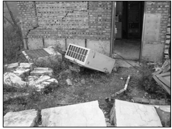
Fig. 6.5. Air-conditioning units were damaged; note the building debris in the foreground
