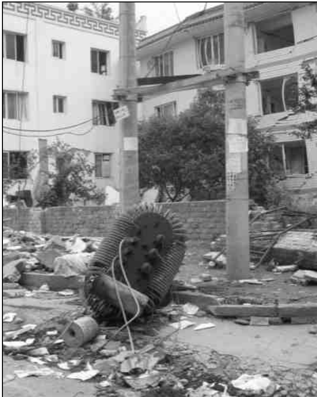
Fig. 4.74. Fallen distribution transformer
