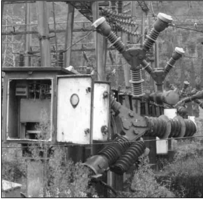
Fig. 4.21. Damage to live tank CBs
