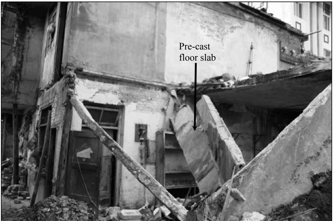
Fig. 9.48. Two-story URM building with pre-cast concrete floor slabs collapsed, which was common in the older part of the city.
