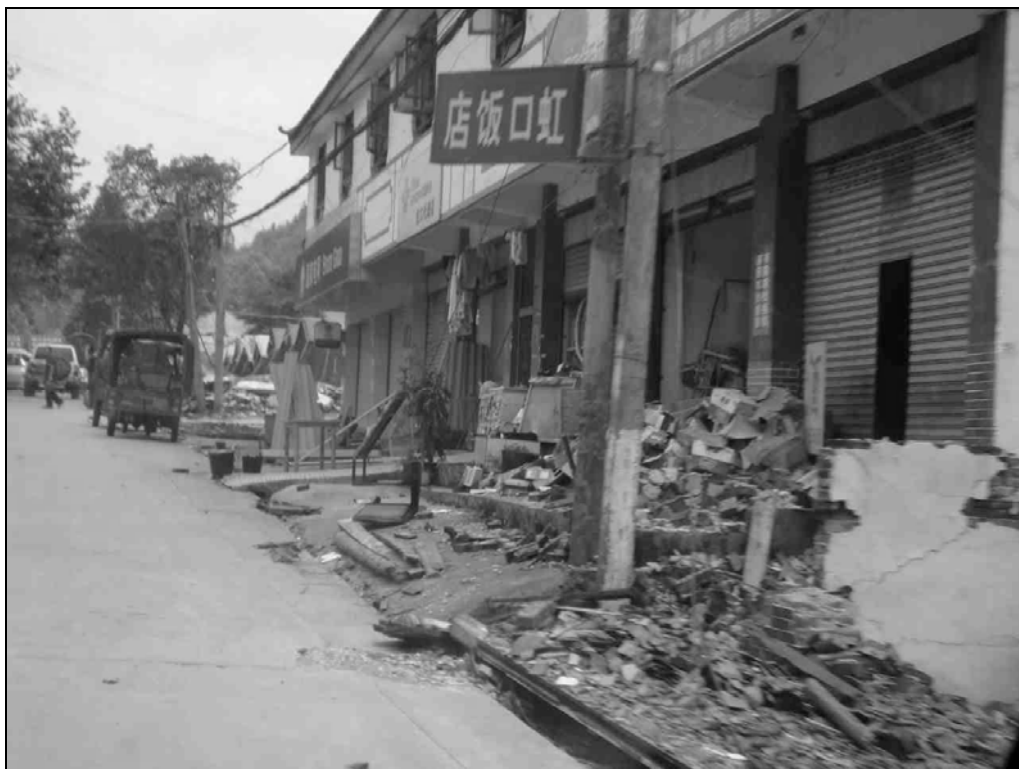
Fig. 9.36. A strip of houses that sustained rather minor damage. Note tents were set up for people whose houses were destroyed.
