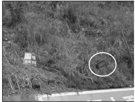
Fig. 6.59. The temporary emergency cable was hanging quite low, with the splice case supported by the cable instead of a guide wire between the poles.
