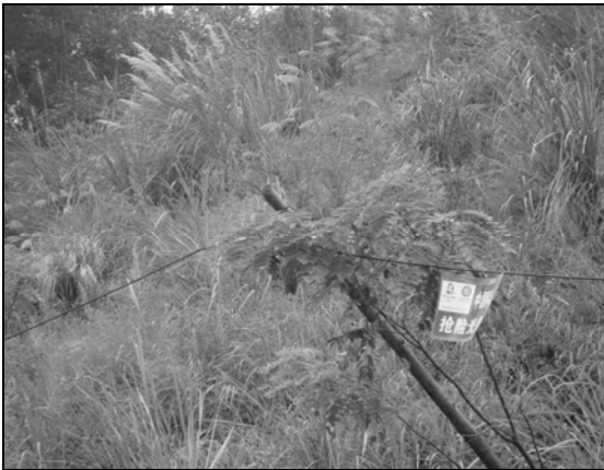
Fig. 6.58. The temporary emergency cable was wrapped around the pole with a very tight bend radius.
