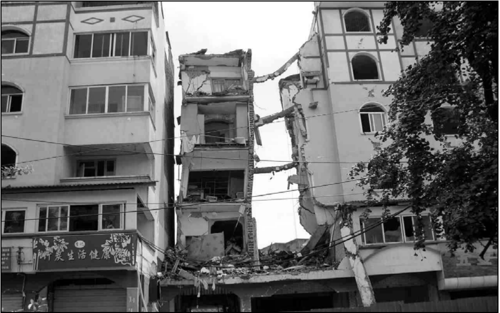
Fig. 9.57. The second floor of the building collapsed with the top four floors resting on it. It appears that the remaining structure is leaning towards the collapsed section.
