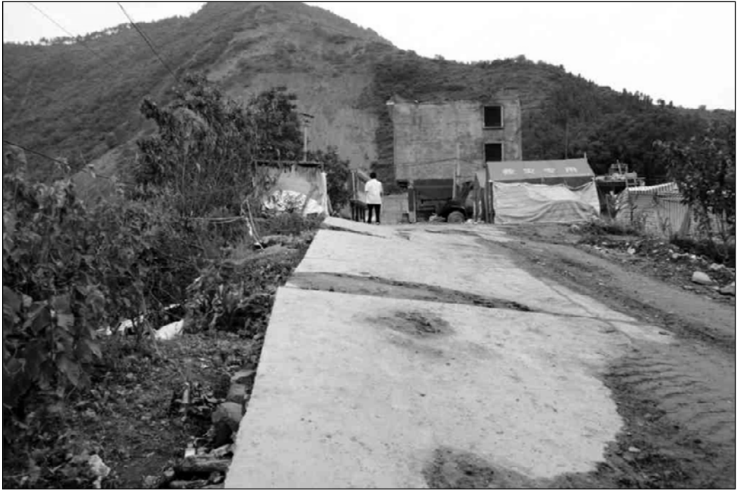
Fig. 3.60. Surface fault in Hejiaba; the road used to be level and a few houses on the right of the photo collapsed
