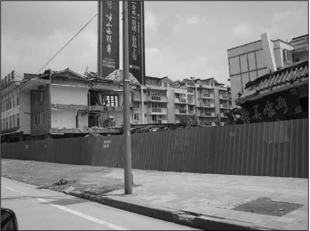
Fig. 9.55. A three-story restaurant building collapsed. Part of the tiled roof shows on the right.
