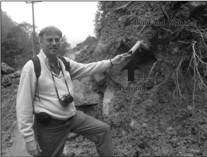
Fig. 5.6. Damage mechanisms to water pipes at one side of a landslide, Shenxigou Village
