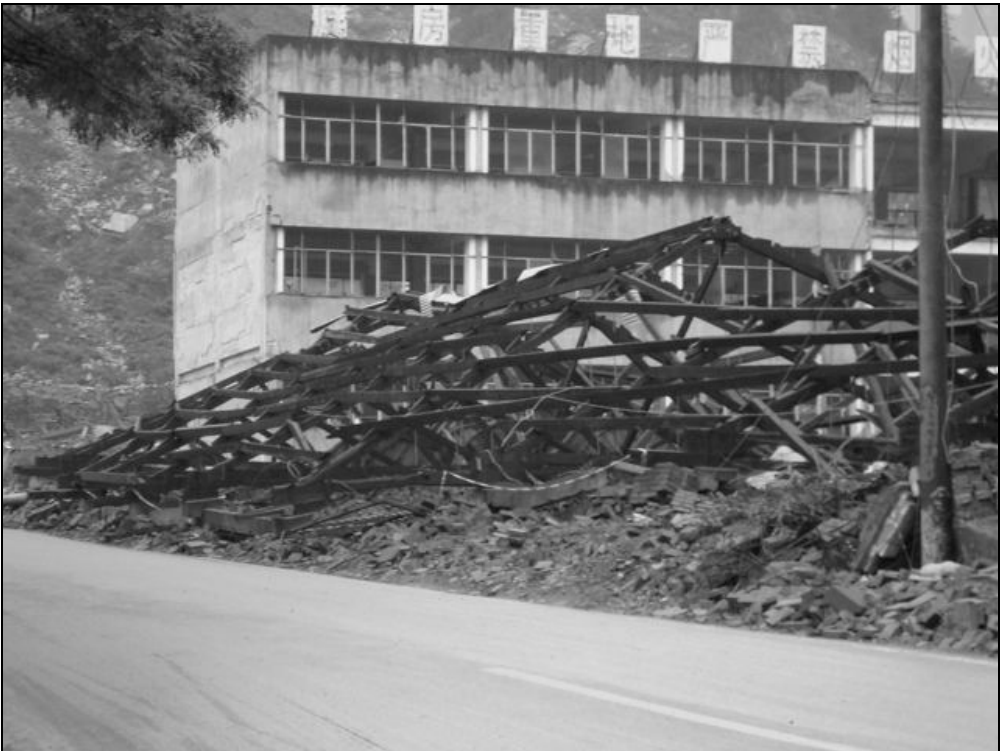
Fig. 9.63. A collapsed manufacturing facility with a standing, but heavily damaged, office building in the background.
