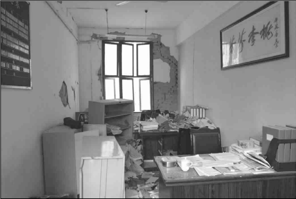
Fig. 6.32. Inside a cell site administrative office, book cases and file cabinets and documents were scattered on the floor. (Courtesy of IEM)
