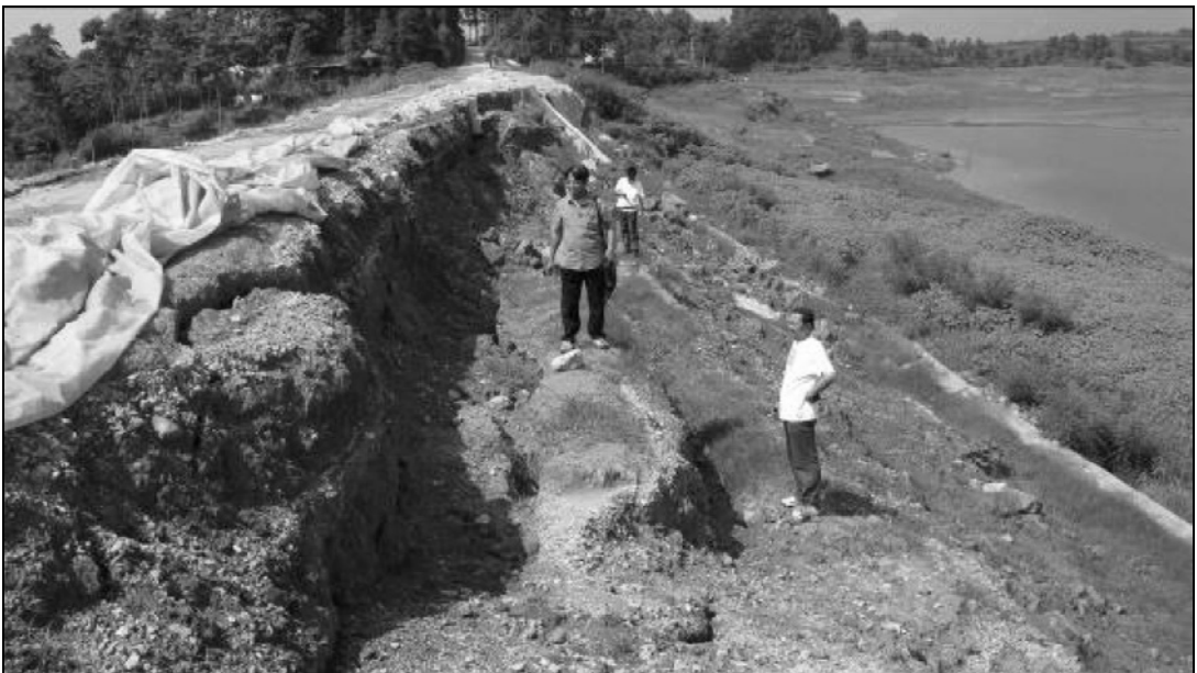
Fig. 8.16. Upstream slope movement of earthen dam, Fengshou Reservoir, Anxian County (Courtesy IEM)
