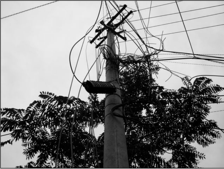
Fig. 6.50. The power lines on the top portion of this pole were not energized. Note the temporary telecommunication cables and the splice case mounted at about mid-height of this pole.
