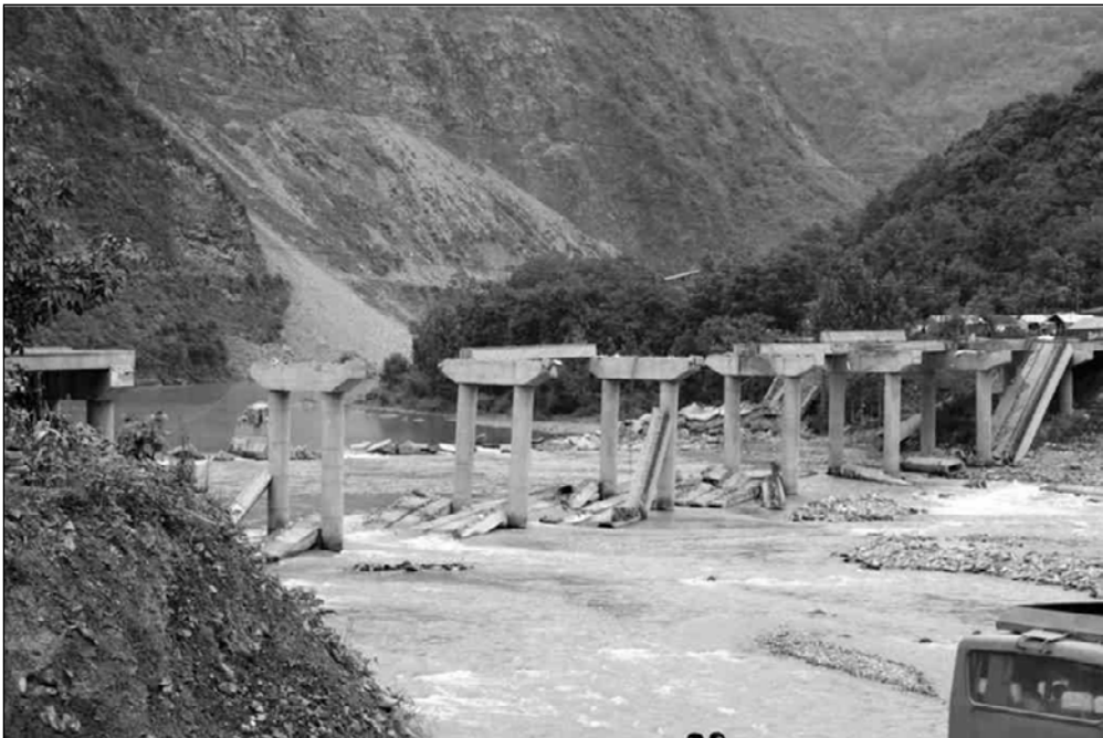
Fig. 3.57. All spans of this partially completed nine-span bridge fell into the river except the two spans on abutments
