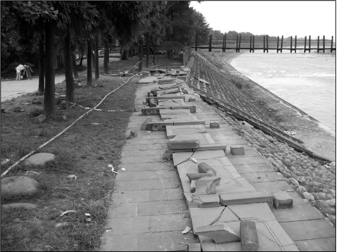
Fig. 5.22. Broken railing wall, note the posts snapped at the base
