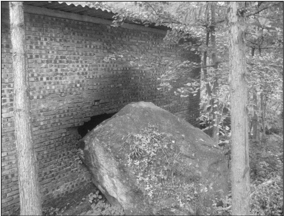
Fig. 9.47. Another boulder impacted one of the building's exterior brick walls.
