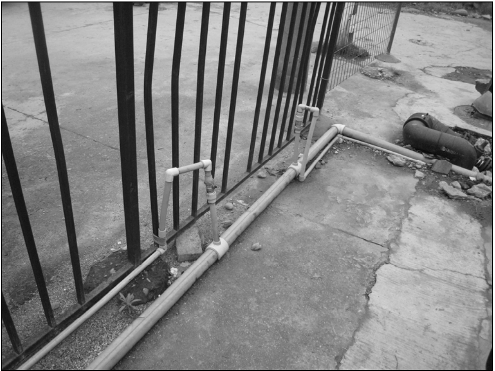
Fig. 5.18. New above ground water pipes (Dujiangyan)
