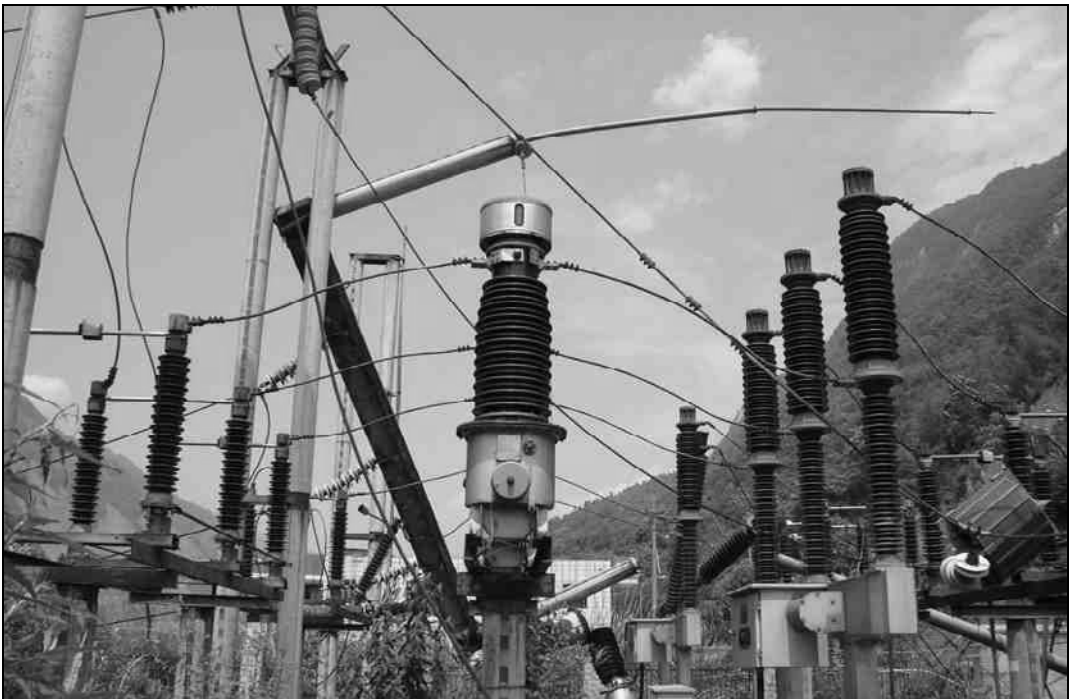
Fig. 4.36. Damage to Beichuan substation, 110 kV (May 2009 photo)
