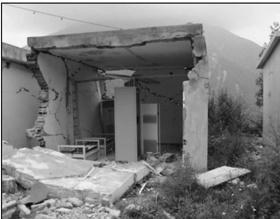
Fig. 6.2. The unreinforced masonry (URM) building was damaged and almost collapsed
