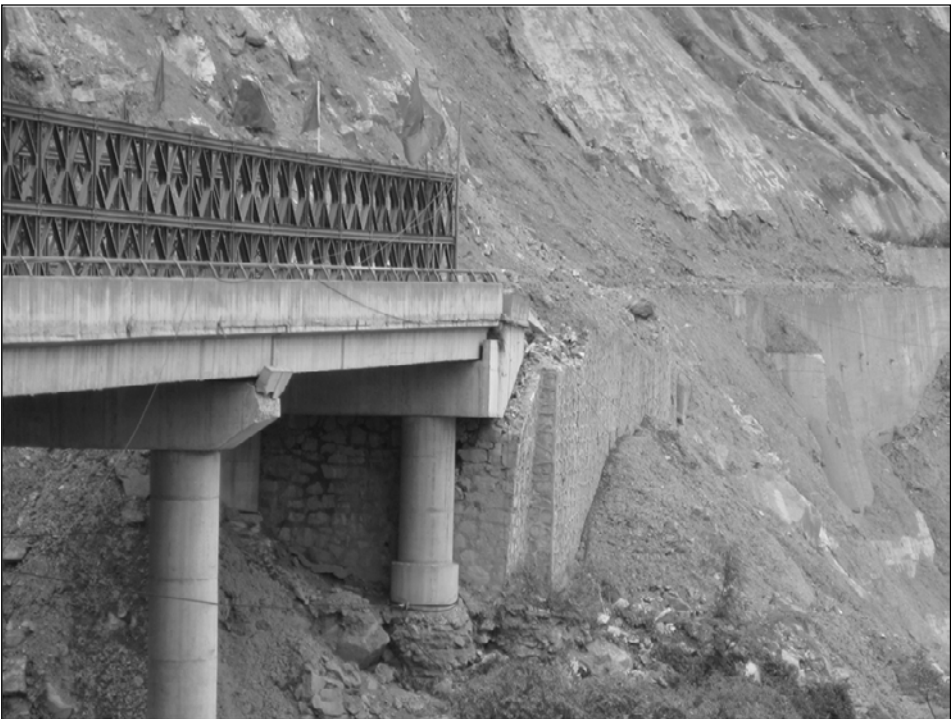
Fig. 3.16. Landslide and ground shaking damage at Zhonghi Bridge near Yingxiu
