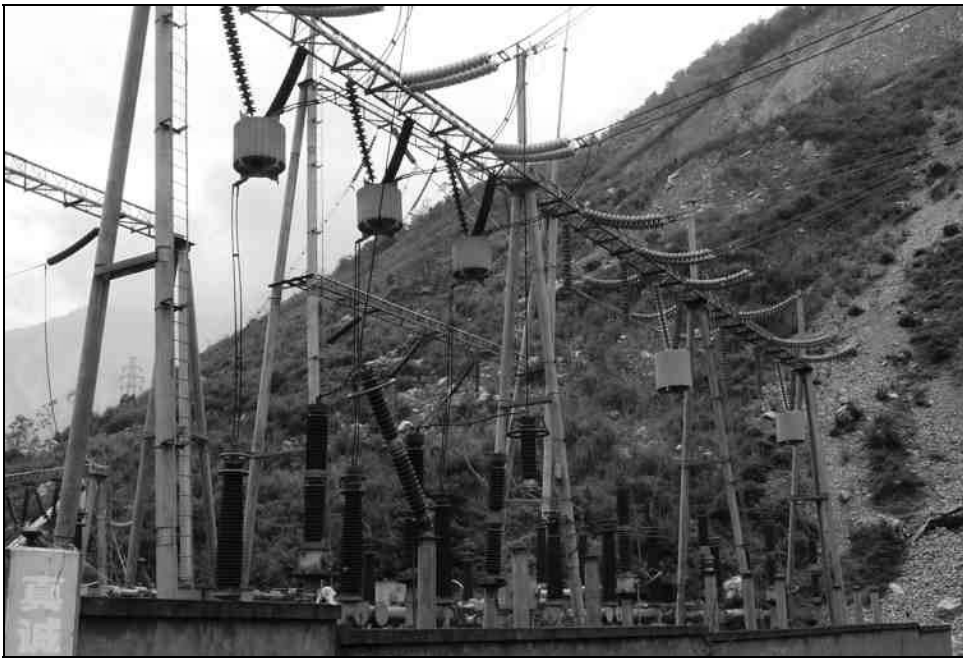
Fig. 4.49. Suspended wave traps, arrester damage (July 2009)
