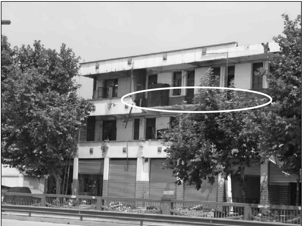
Fig. 9.50. This concrete frame building performed well except for the masonry railing on the third floor.
