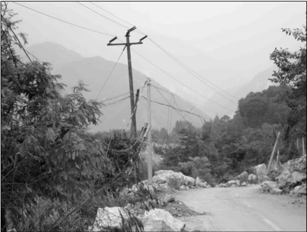
Fig. 6.42. Both concrete and wood poles were damaged at this section of the road leading to Hongkou. Fallen rocks were pushed to both sides of the road to clear the road for cars.
