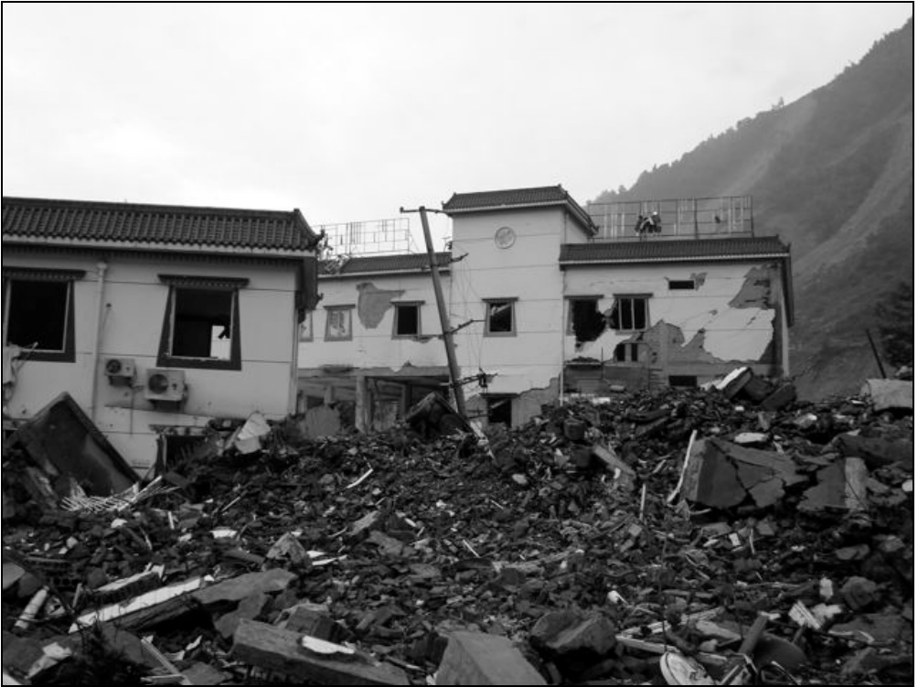
Fig. 9.62. Partially and totally collapsed buildings were seen everywhere in this small town.
