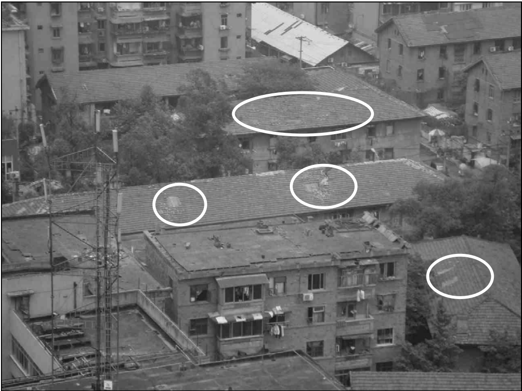
Fig. 9.70. Tiles fell of the roofs of these buildings in the center of Chengdu.
