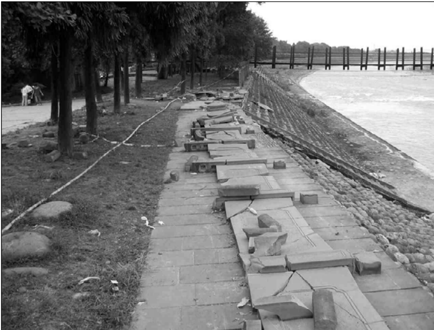
Fig. 3.68. The poles of the stone railing close to the flexible pedestrian bridge were sheared off the stress riser close to the base
