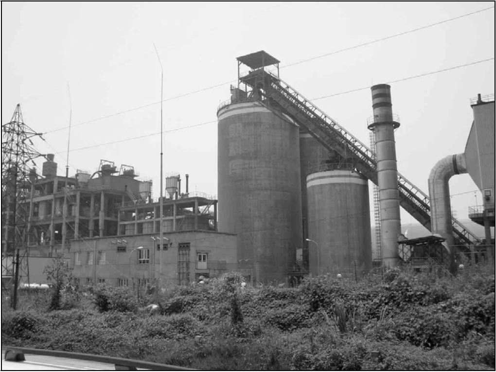
Fig. 9.74. The silos for processed material, located about 200 m apart, showed no signs of damage. The damaged silo is located to the right of this group of silos.
