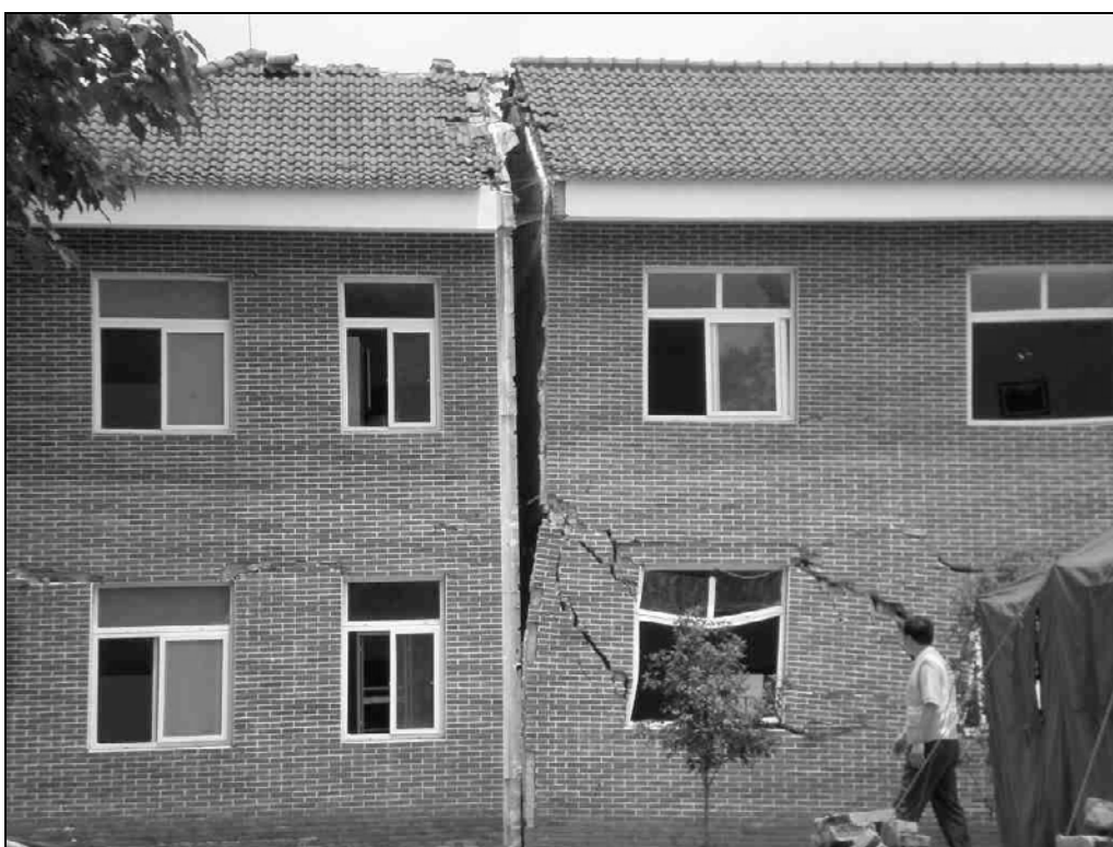
Fig. 9.37. These houses showed significant structural damage but did not collapse.
