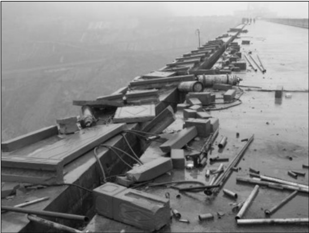
Fig. 8.7. Collapsed guardrail on dam top (Courtesy IEM)
