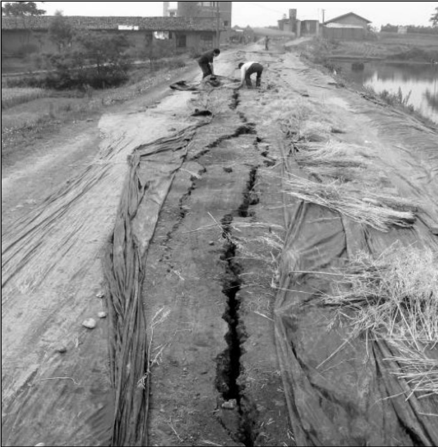
Fig. 8.13. Longitudinal cracks at crest of earthen dam, Dasongshu Reservoir (Courtesy IEM)
