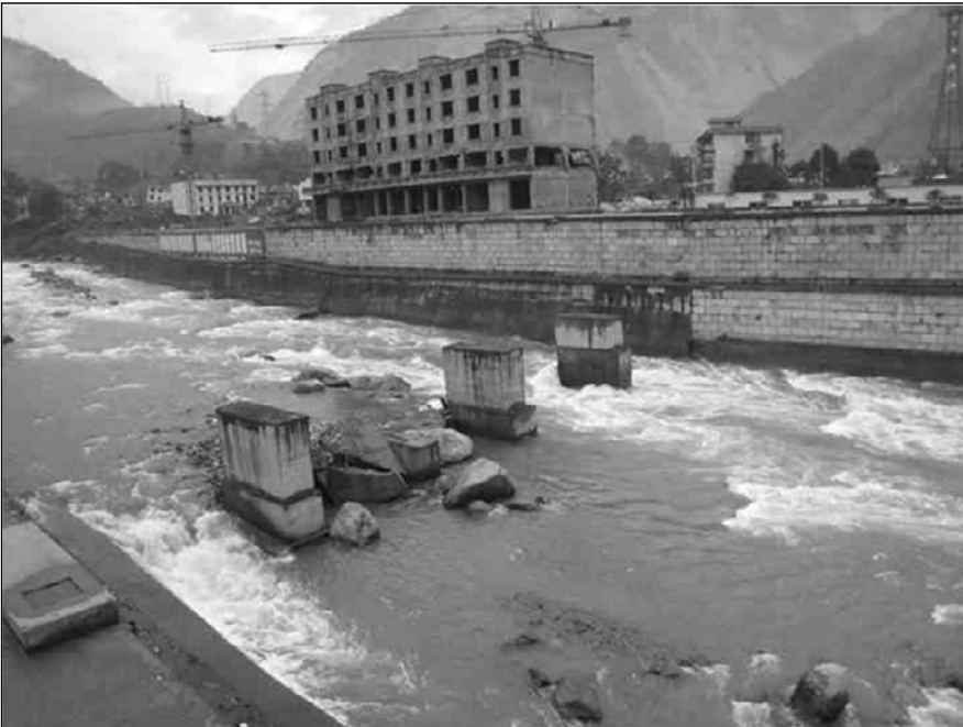
Fig. 3.38. Collapsed four-span bridge at Yingxiu
