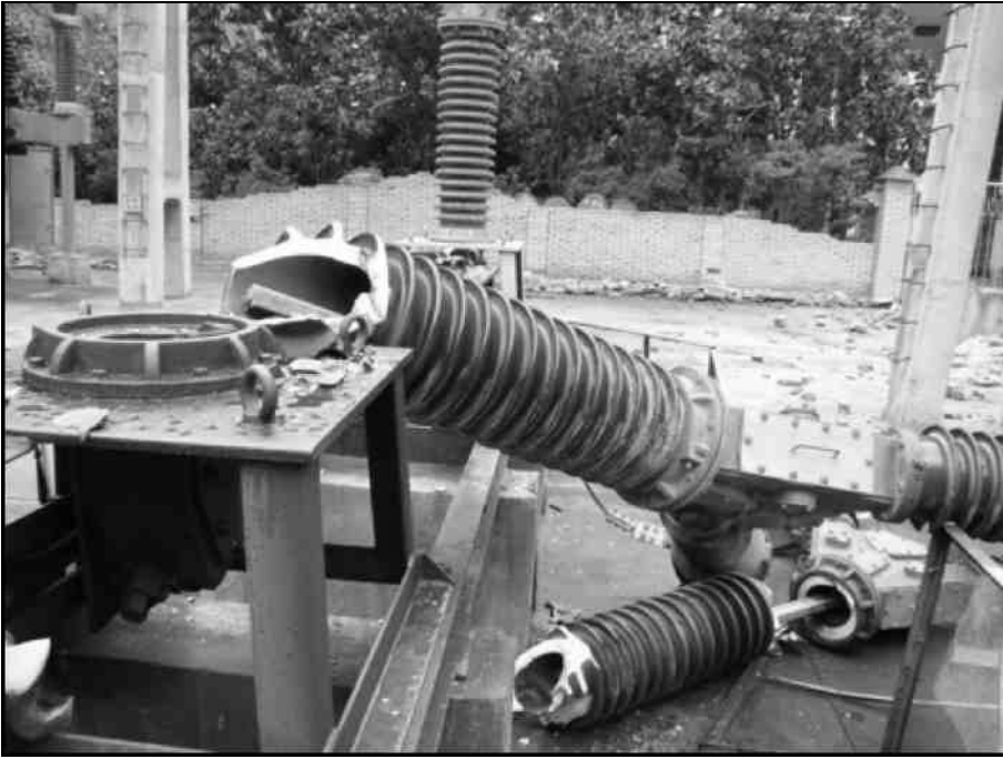
Fig. 4.6. Close-up of damaged live tank circuit breaker (110 kV)
