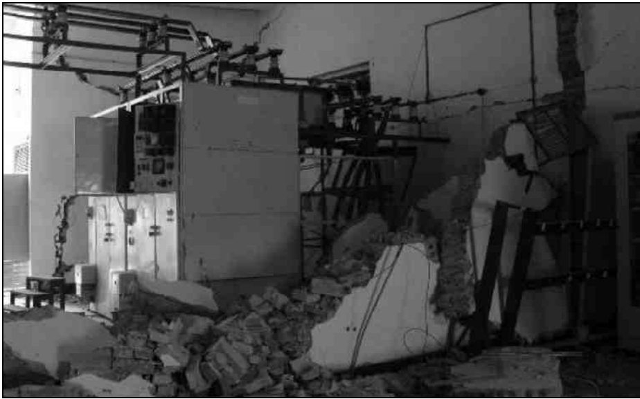
Fig. 4.42. Control Building Equipment Damage, Yuanmenba Substation
