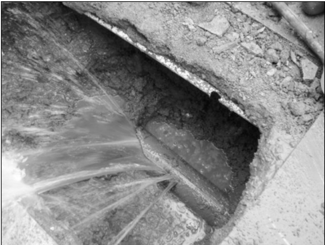
Fig. 5.1. PVC water pipe with split
