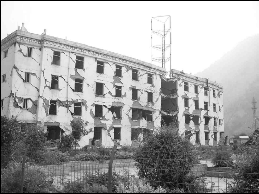
Fig. 9.3. Yingxiu, Xuan Kou High School student residence was heavily damaged but did not collapse.
