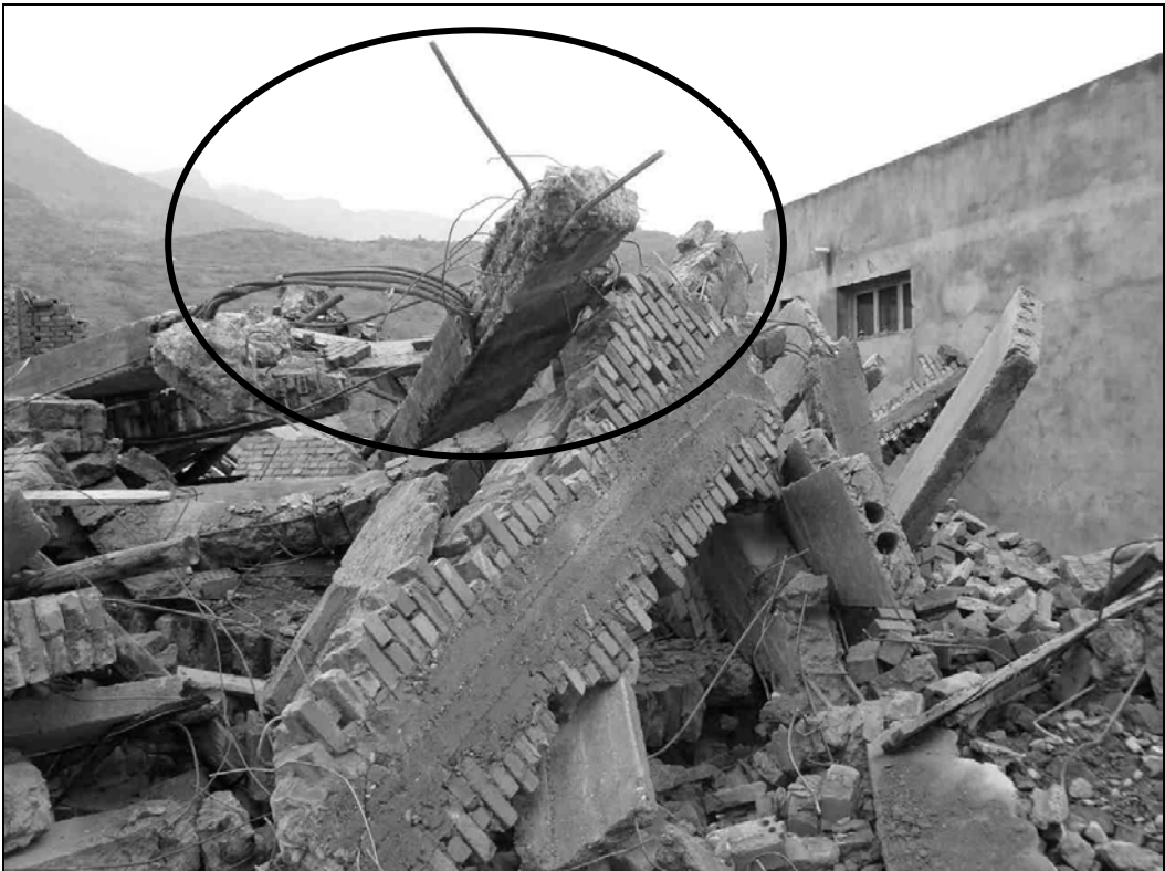
Fig. 9.84. A collapsed concrete frame building showing the reinforcement bar. The pre-cast floor slabs were resting on beams without structural connection to the concrete frame.
