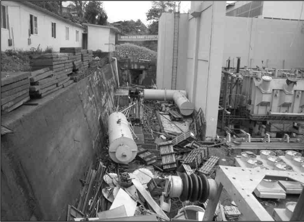
Fig. 4.25. Oil conservator tanks
