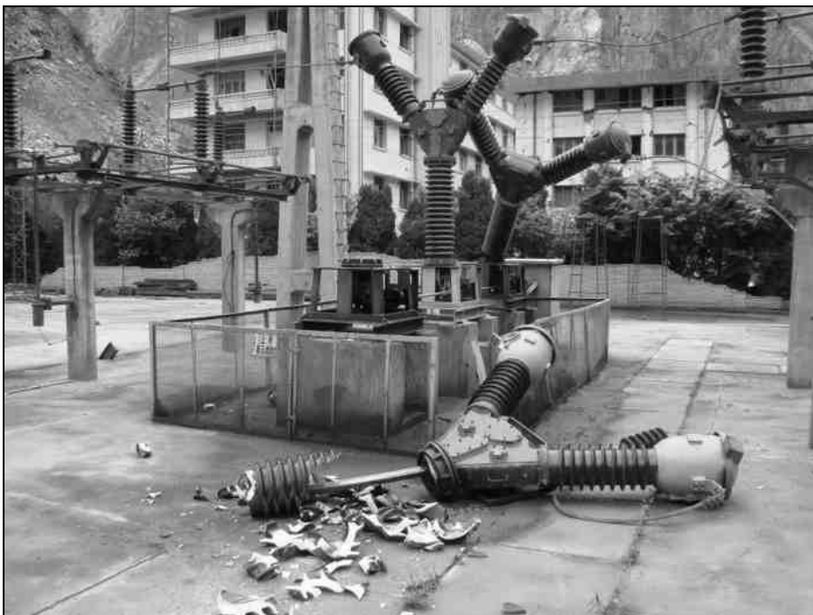
Fig. 4.40. Damage to live tank circuit breakers, Caopo Power Plant
