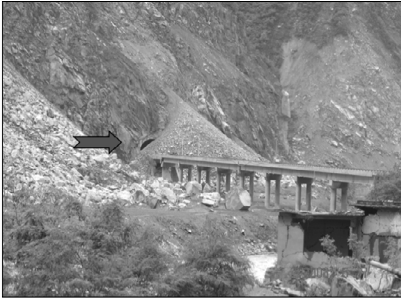
Fig. 3.73. Portal landslide, Futang Tunnel in Duwen (Courtesy CRSWRI)
