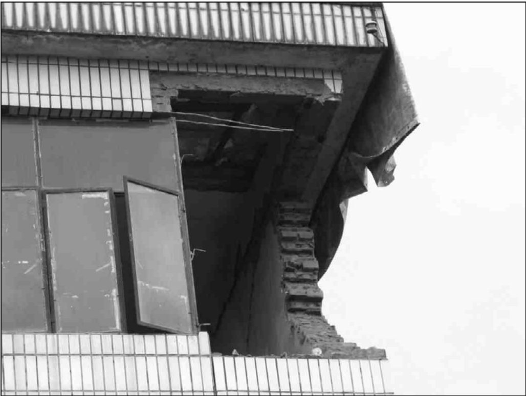
Fig. 9.49. Collapsed brick infill walls, another common scene within Dujiangyan.
