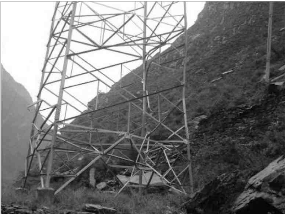
Fig. 4.69. Rockfall impacted tower, #14, Tianjin line, Jinlong Lake area, Wenchuan
