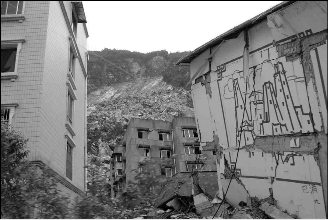
Fig. 9.21 Landslide that damaged and buried a number of buildings along its path.
