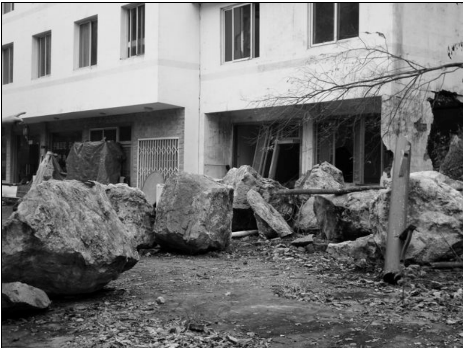
Fig. 9.43. The courtyard the hotel was littered with boulders that rolled down from the mountain above. The house on the right was damaged by the boulders.
