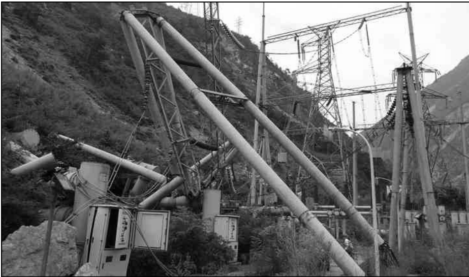
Fig. 4.48. Tubular concrete dead end structure and 110kV GIS were damaged by the landslide
