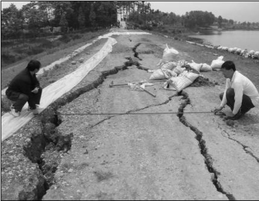
Fig. 8.15 Longitudinal cracks at crest of earthen dam, Fengshou Reservoir, Anxian County (Courtesy IEM)
