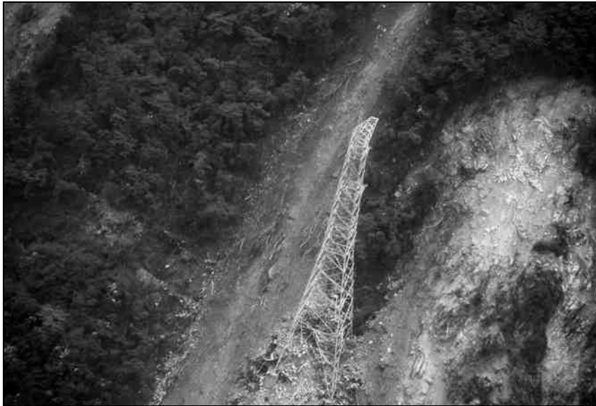
Fig. 4.59. Tower with damaged arm
