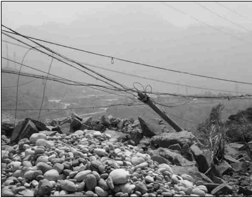
Fig. 4.72. Pull down of power and telecom distribution due to landslide
