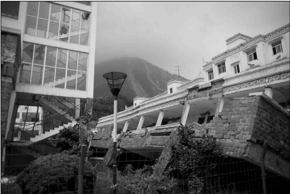
Fig. 9.4. Other building within the school campus sustained extensive structural damage. Many students were injured and killed.
