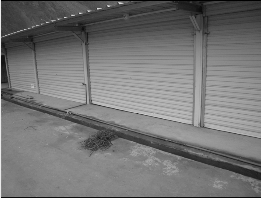
Fig. 5.8. Temporary above ground water pipe with hose bib to temporary housing in Yingxiu
