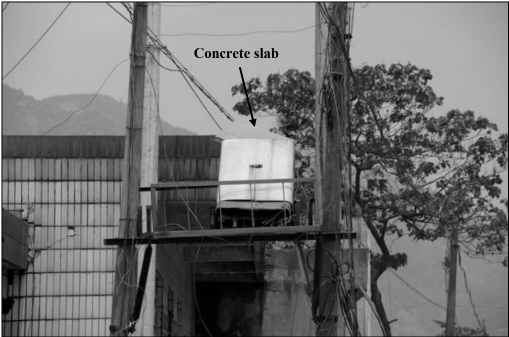
Fig. 6.53. Note the concrete slab on top of the pair gain unit on the platform between the poles.
