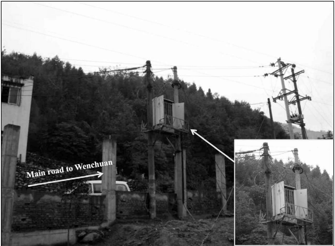
Fig. 6.39. A cross connect box mounted between the utility poles was opened to allow the service crew to remove connections and connect telecommunication service to temporary shelter areas.
