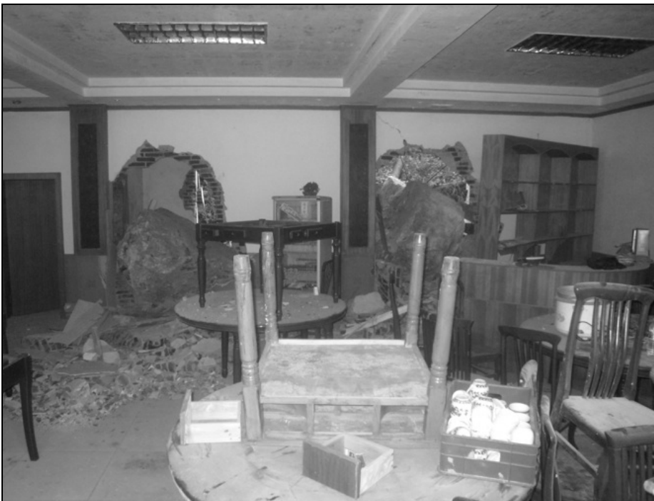
Fig. 9.45. Two boulders entered the hotel dining room through the wall causing lots of damage. Luckily the boulders missed the columns; otherwise, the building would have collapsed.
