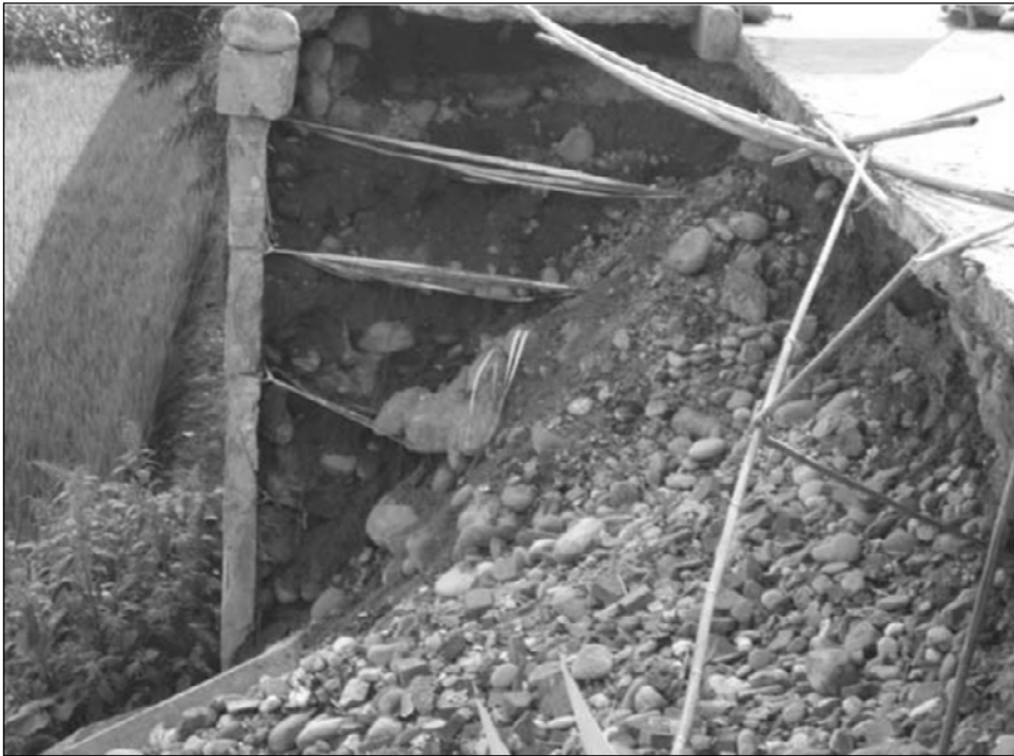
Fig. 3.21. Failure of MSE wall supporting a roadway
