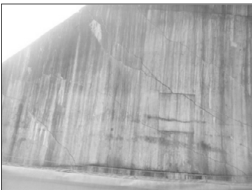
Fig. 3.78. Damage, Longxi Tunnel approach (Courtesy CRSWRI)
