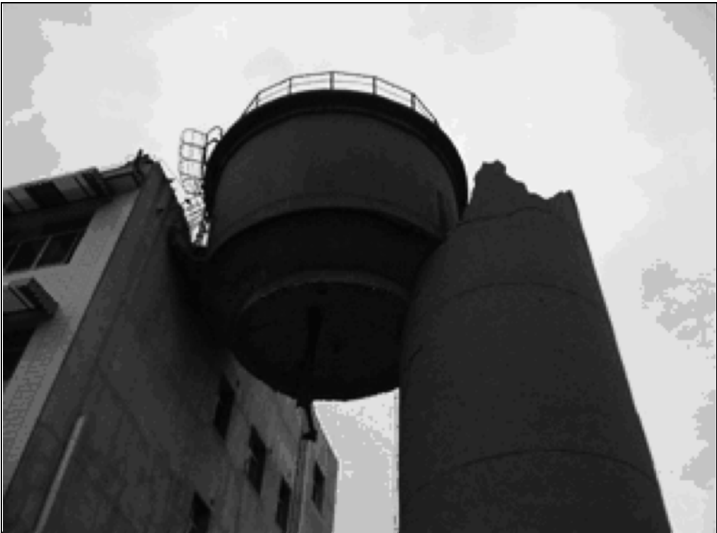
Fig. 5.11. Collapsed elevated concrete water tank
