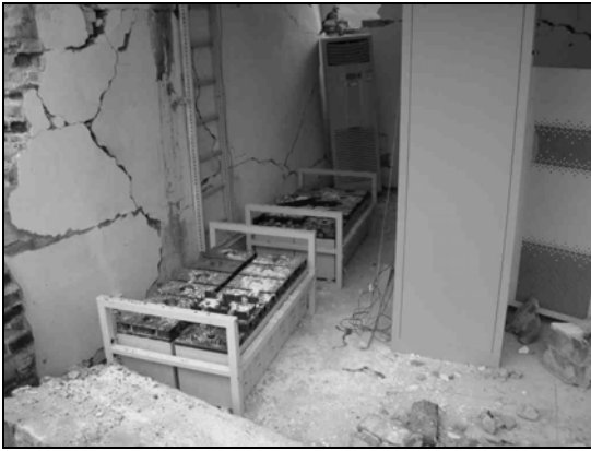
Fig. 6.4. Damaged batteries due to building damage
