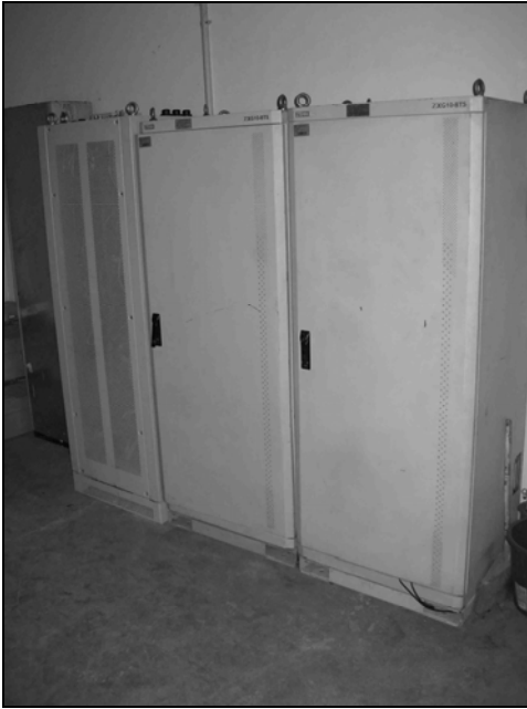
Fig. 6.11. Power equipment in the cell site building
