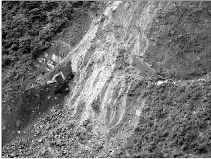
Fig. 3.4. Landslides blocked many roads
