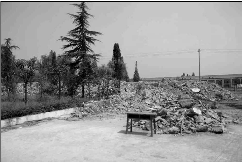
Fig. 9.7. Piles of bricks are the only remains of this primary school. Only a classroom desk indicates that this was a school. The one-story building used for student activities in the background did not collapsed; however, there were cracks on outside walls.
