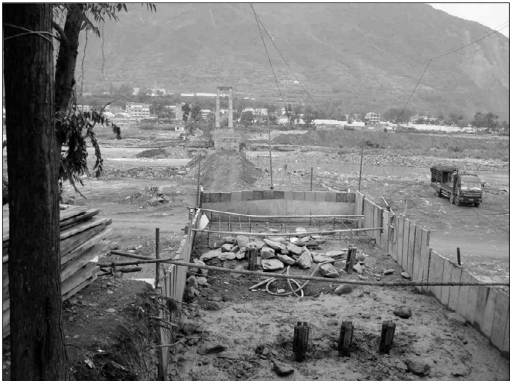
Fig. 3.61. View from Hejiaba towards Nanba of collapsed bridge and construction of new abutment
