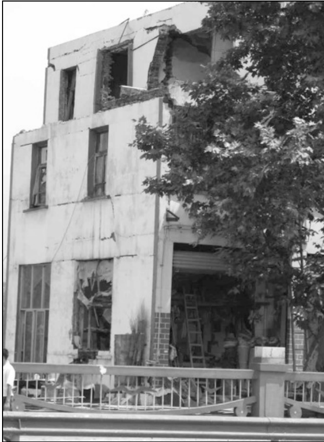
Fig. 9.51. The third floor of this building fell about 1 m to the second floor and shifted to the right.
