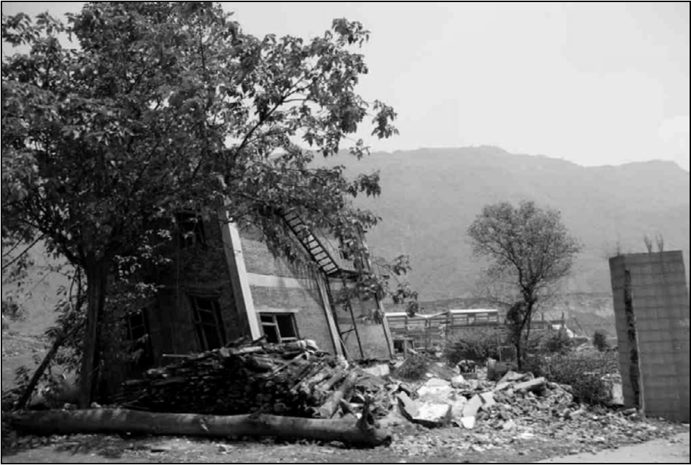
Fig. 9.80. A concrete frame residential building almost tipped over. The structure seems to be in good condition. Most likely the foundation was not properly treated before constructing the building.
