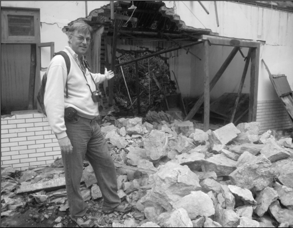
Fig. 9.46. One boulder broke through the back and front wall. It was cut into smaller pieces before the team's visit.
