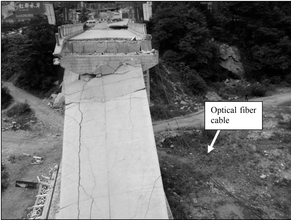
Fig. 6.44. The telecommunication cable on the right side of the collapsed span was damaged.
