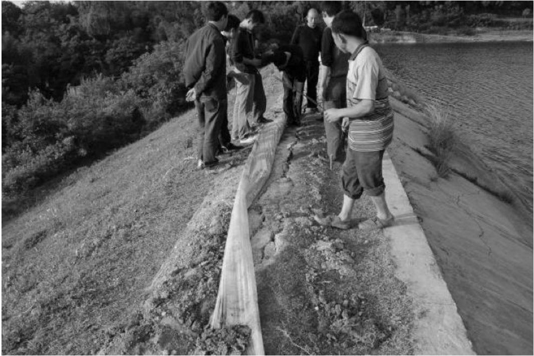
Fig. 8.11. Longitudinal cracks at crest of newly constructed earthen dam, Fenggu Town, Mianyang City (Courtesy IEM)
