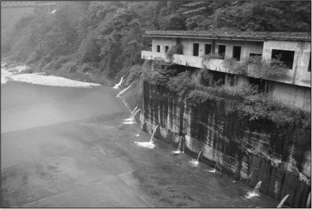
Fig. 8.10. Hongkou Dam right abutment seepage
