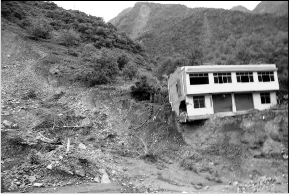
Fig. 9.82. The first house we saw on the road to Nanba was located about 2 km from the center of the town. Note that the foundation is just a concrete pad without footing.
