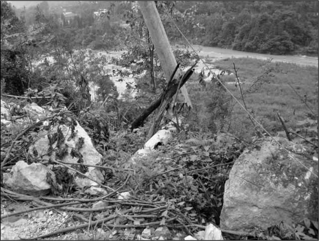
Fig. 6.40. A pole damaged by the rock falling from the slope across the road
