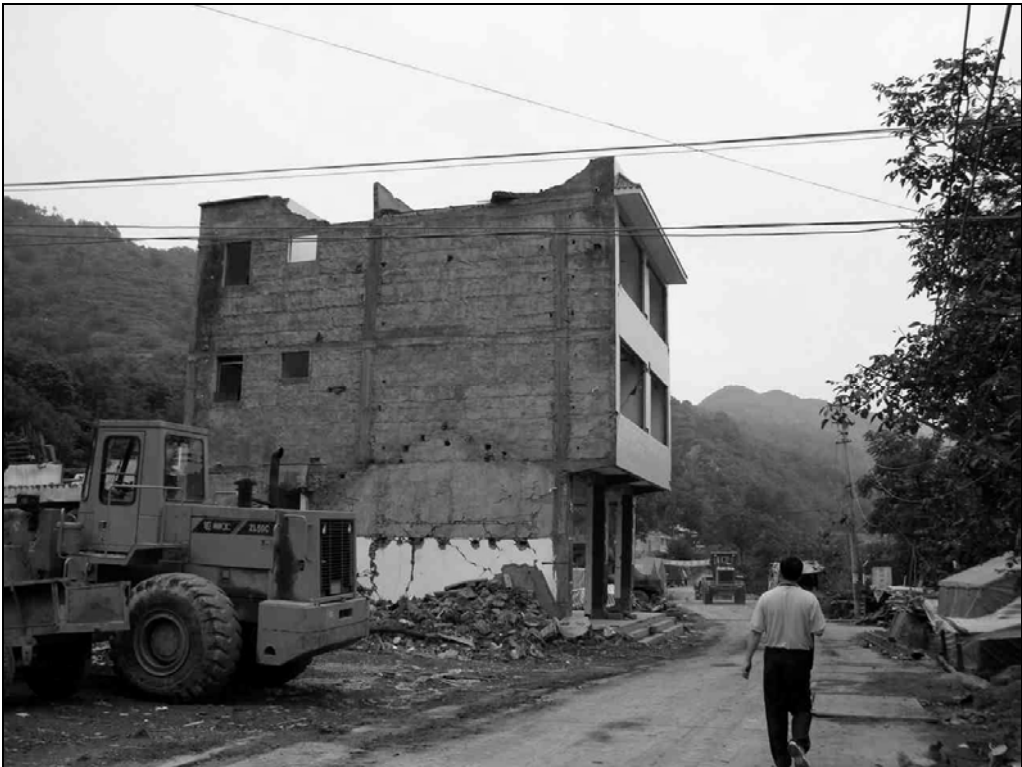
Fig. 9.89. This building is the furthest from the surface rupture, yet it sustained extensive damage and was unsafe to use.
