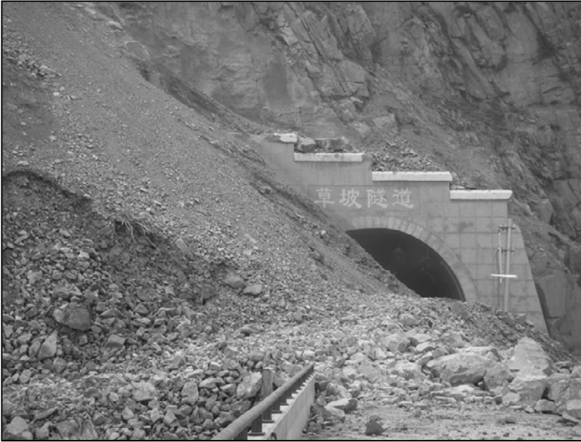
Fig. 3.70. Portal landslide, Caopo Tunnel in Duwen (Courtesy CRSWRI)
