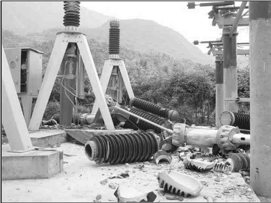
Fig. 4.7. Damaged live tank circuit breaker (220 kV)
