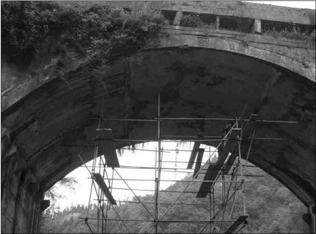
Fig. 3.64. Arch bridge sustained damage, Zhongba Village of Pengzhou City
