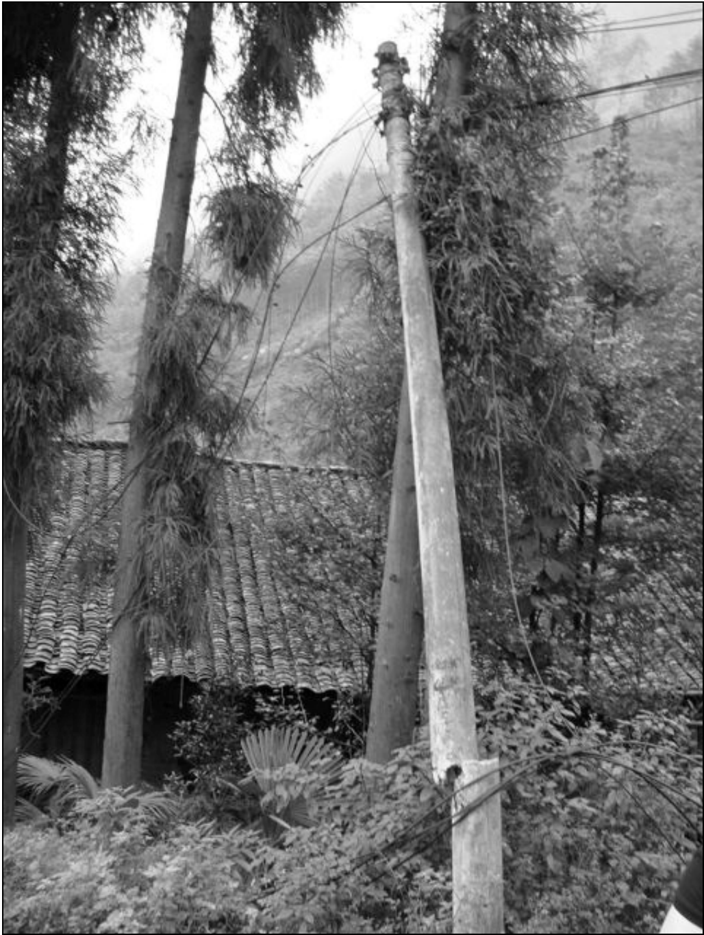
Fig. 6.43. There was no rock fall and no landslide in this neighborhood. Most likely this pole was damaged by the strong shaking as surface fault was observed in this area.
