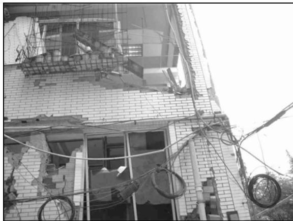
Fig. 6.31. The walls of this cell site building collapsed damaging the equipment inside. (Courtesy of IEM)
