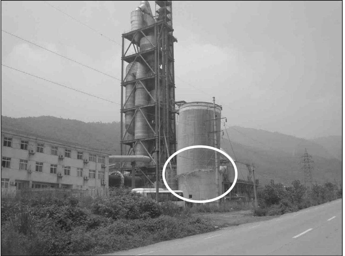
Fig. 9.73. The raw material silo at this chemical processing plant in Shifang collapsed at about mid-height. This is the only silo in this plant that was damaged.
