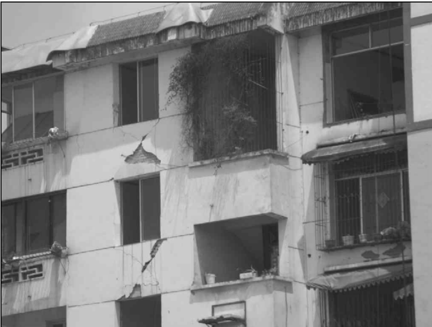
Fig. 9.52. This concrete building performed quite well; only minor stress cracks were observed on the outside. The windows were not broken.
