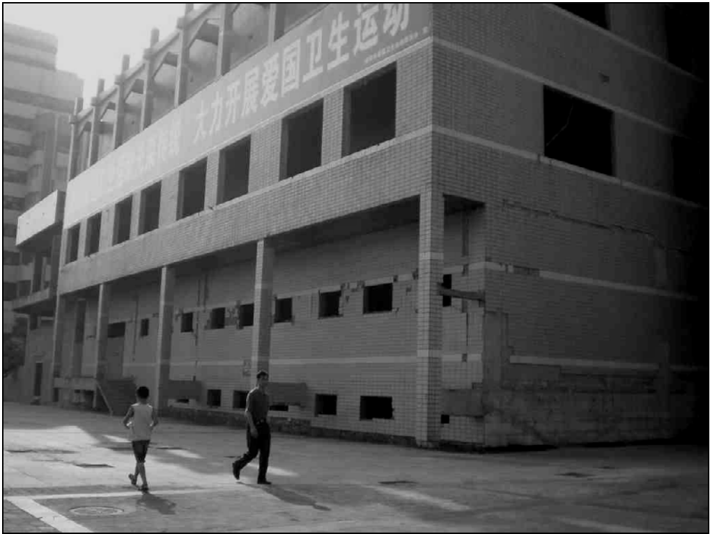
Fig. 9.69. The building next to the hotel ASCE/TCLEE Phase I team members stayed was damaged and closed.
