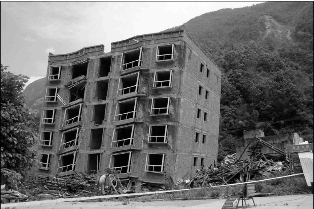
Fig. 9.30. This partially finished building leaned backward along with major structural set back. It was empty with not load on it.
