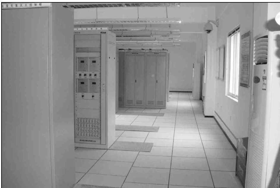
Fig. 4.80. The control room is built with a raised floor. It is not clear whether the equipment on the raised floor is anchored or not.
