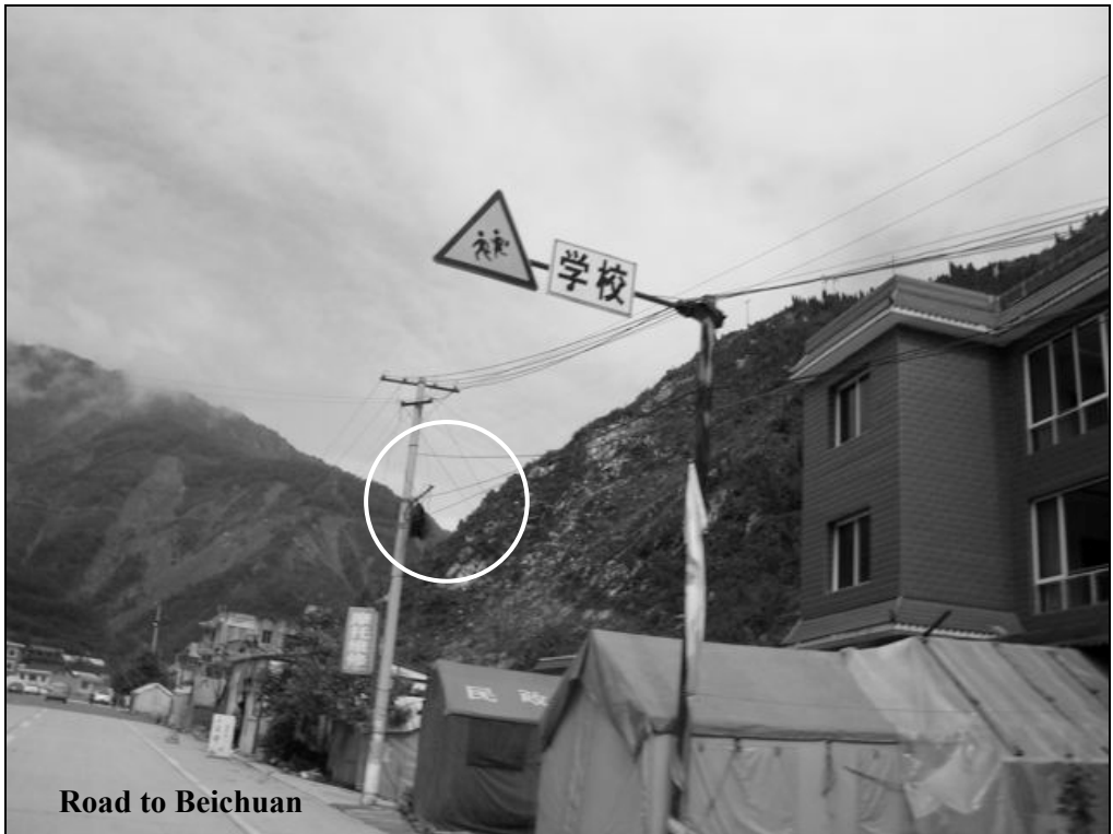
Fig. 6.61 Optical fiber cables (in the circle) for emergency repair were bundling up on the pole.
