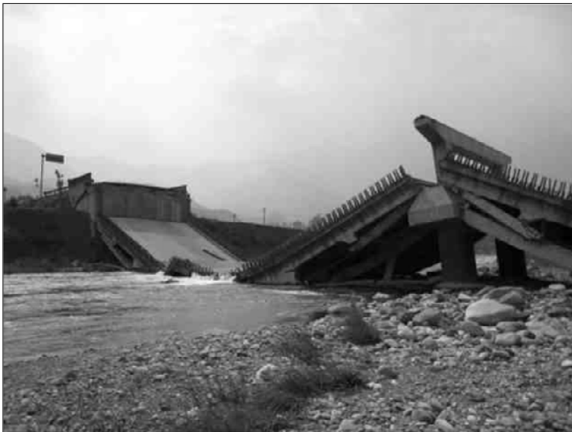
Fig. 3.50. Collapsed Xiaoyudong Bridge span (Longmenshan town and Xiaoyudong town)
