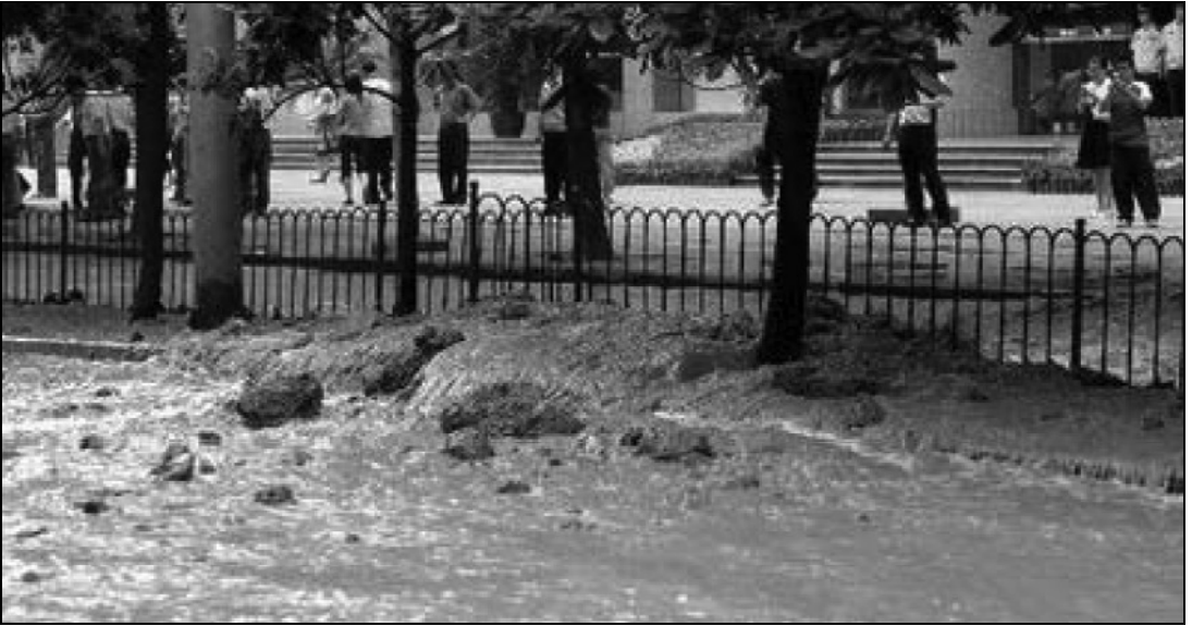
Fig. 5.4. Broken water pipe in Chengdu City
