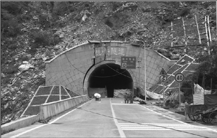
Fig. 3.74. Cracking of Taoguan Tunnel in Duwen (Courtesy CRSWRI)
