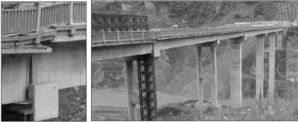
Fig. 3.25. Photos of dropped span at Bent 2 of Shoujian Bridge
