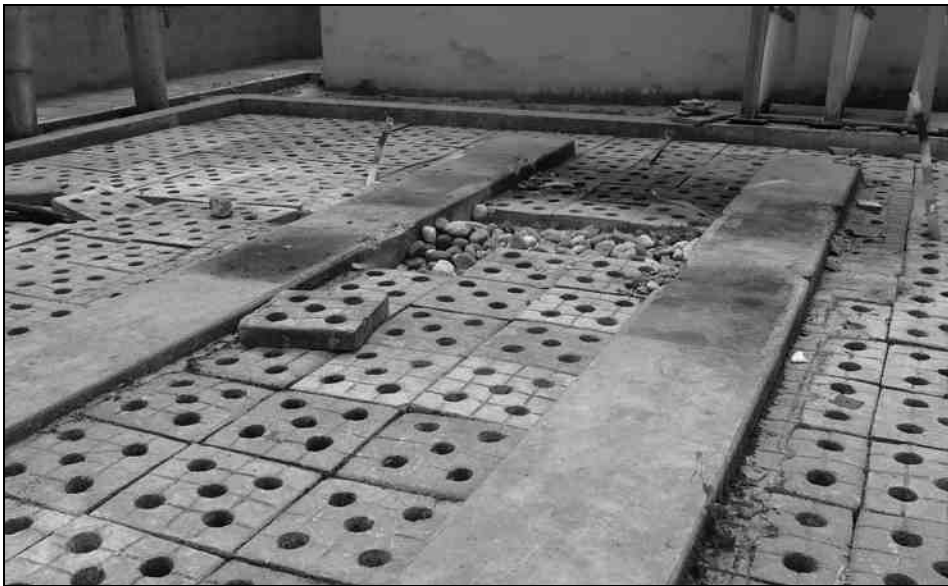
Fig. 4.52. Unanchored transformer slid off this foundation, later relocated.
