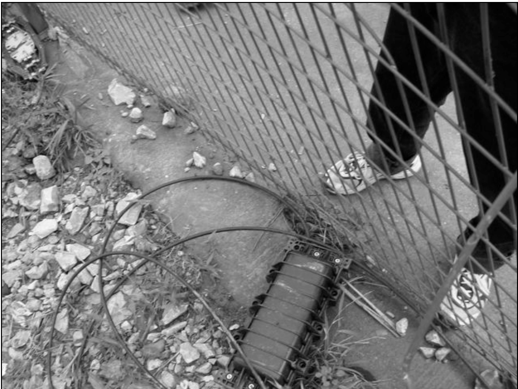
Fig. 6.56. A splice case for a temporary optical fiber cables was placed on the side of the road.
