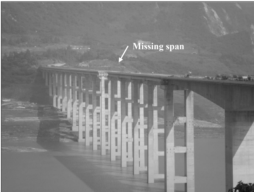
Fig. 3.28. Miaoziping Bridge with Missing Span (13 th span), many other spans shifted (taken in July 2009)
