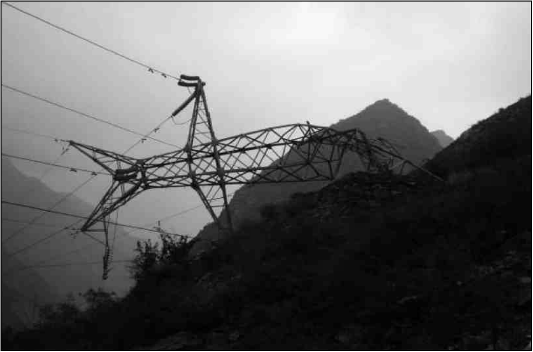
Fig. 4.70. Collapsed tower, #11, Tianjin line, Jinlong Lake Area, Wenchuan
