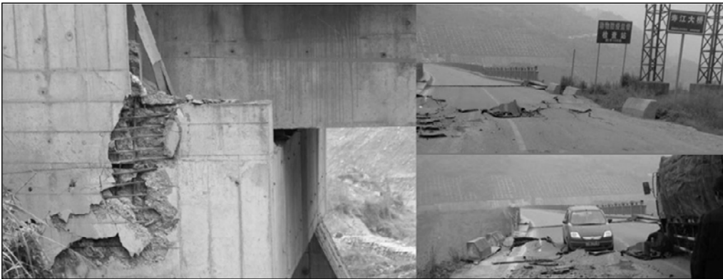
Fig. 3.26. Photos of damage at the north abutment
