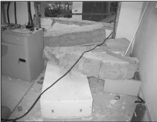
Fig. 6.28. The walls of this cell site building in Dujiangyan collapsed and damaged the equipment. (Courtesy of IEM)
