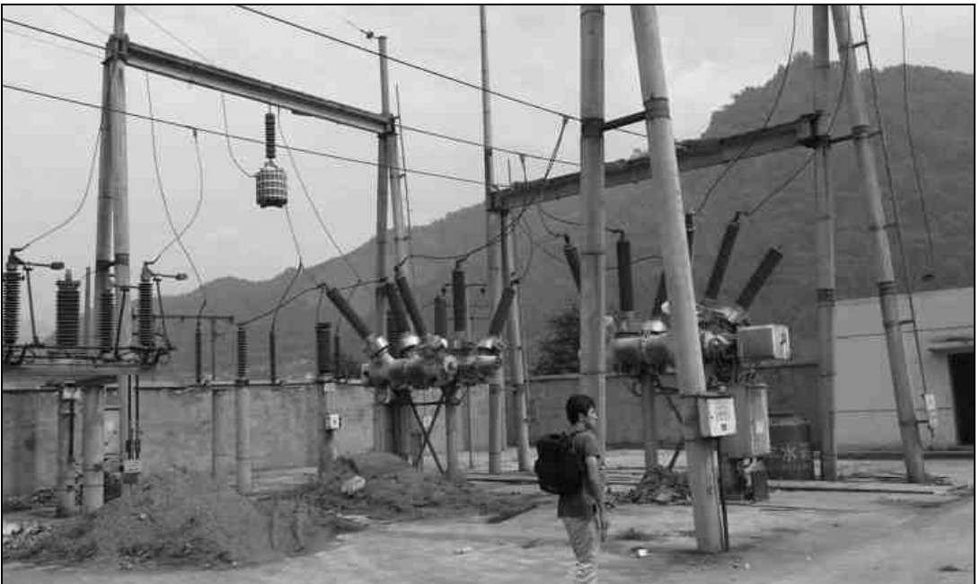
Fig. 4.54. Disconnect switch, bus supports, and SF 6 circuit breakers
