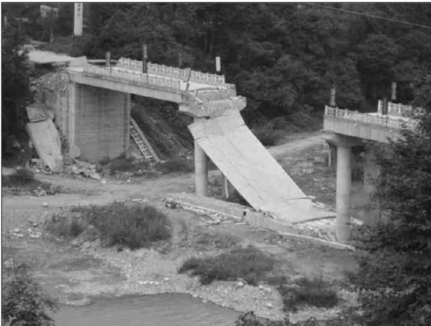
Fig. 3.46. Failed span of the Gaoyuan four-span bridge (Hongkou)
