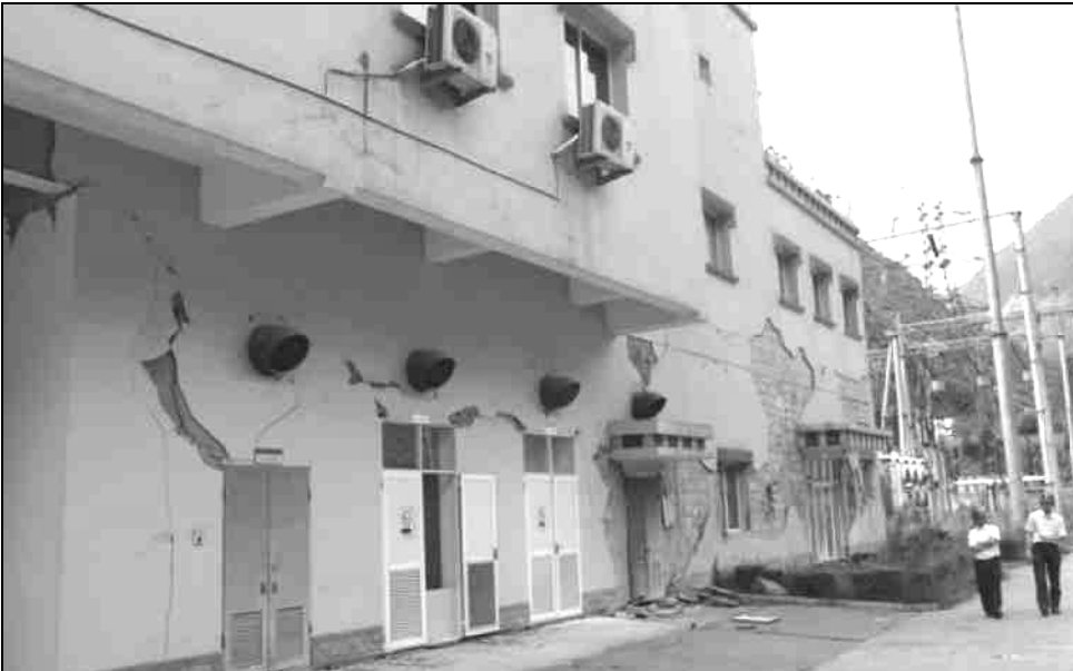
Fig. 4.51. Control building damage
