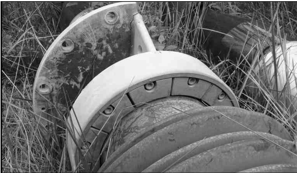
Fig. 4.46. 220kV bushing with cracked flange
