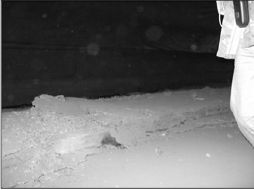
Fig. 3.80. Upheaval damage by 70 cm (Courtesy CRSWRI)
