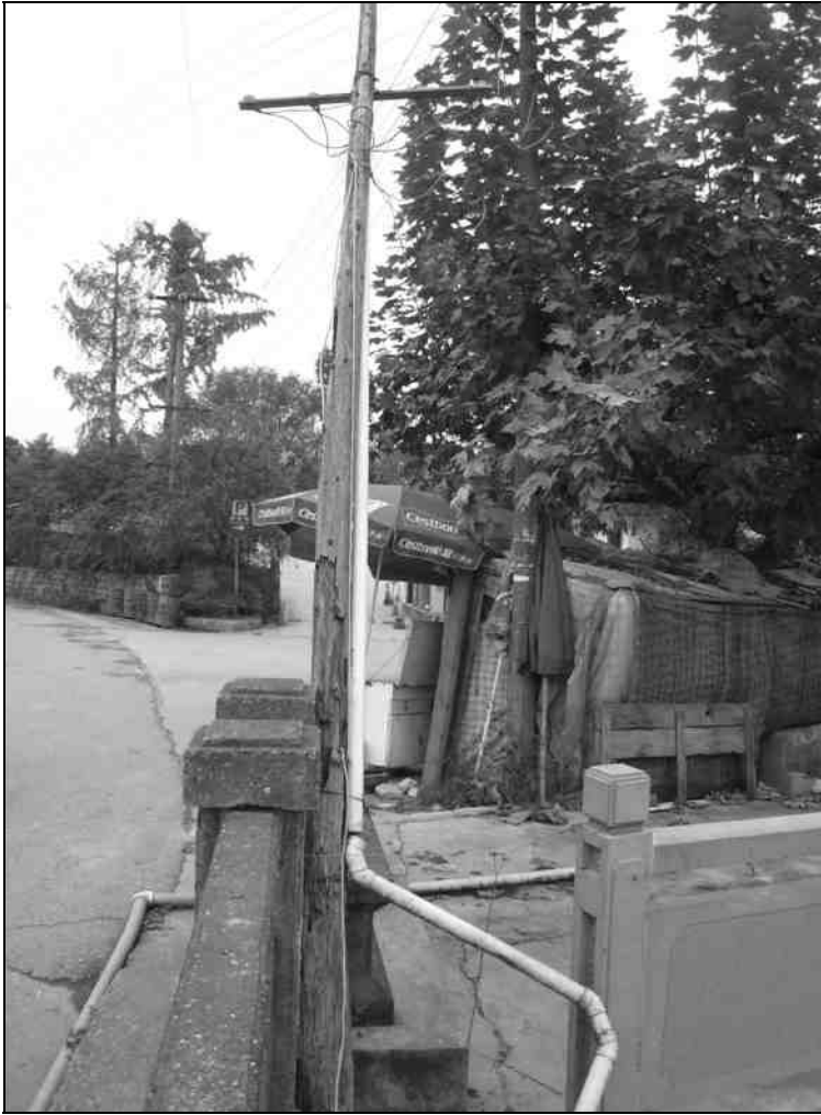
Fig. 4.76. Damage to low-voltage power conduit at bridge abutments
