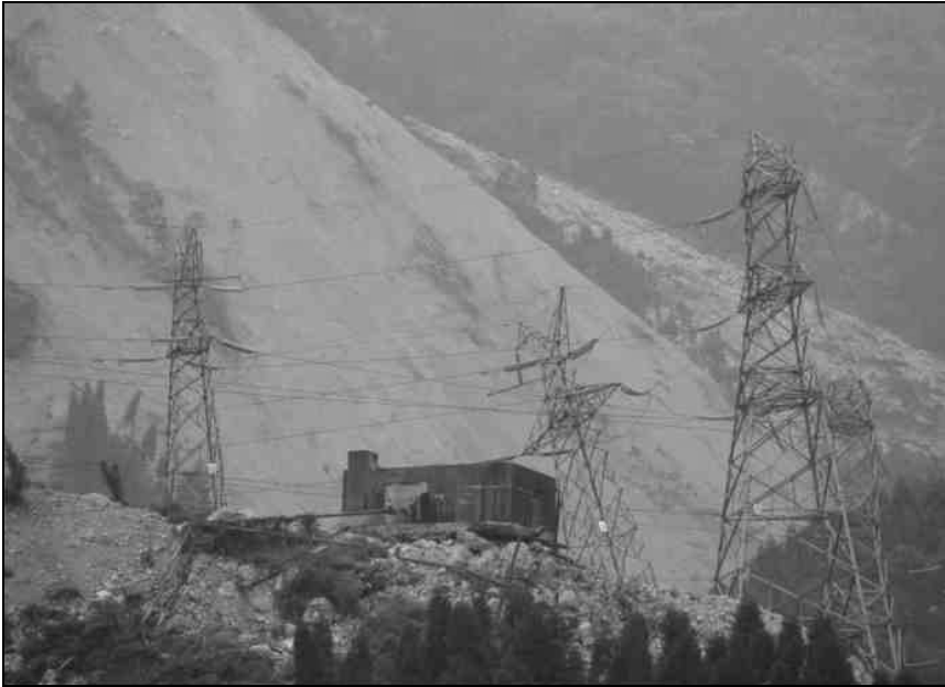
Fig. 4.58. Tilted transmission tower, possibly due to landslide (Yingxiu)
