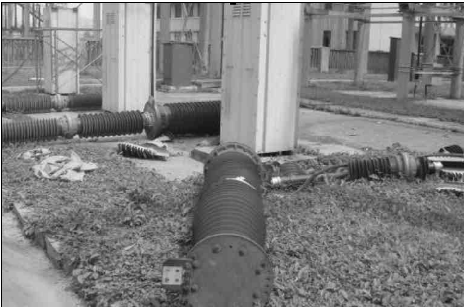
Fig. 4.44. Live tank breaker damage, Jiangyou Power Plant
