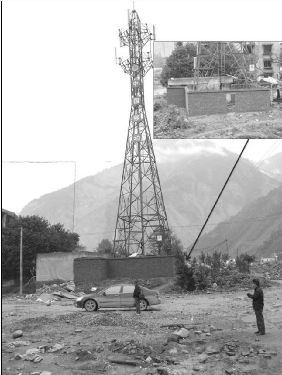
Fig. 6.9. A China Mobile cell site in Yingxiu. Insert shows a missing door in the new wall.
