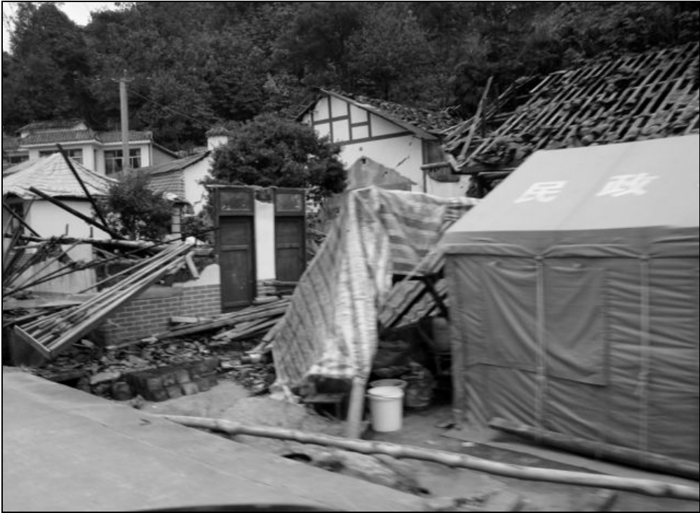
Fig. 9.34. Collapsed timber roofs of the URM houses. The tent was set up by the PLA for the victims and those who did not want to return to their houses due to large number of strong aftershocks.
