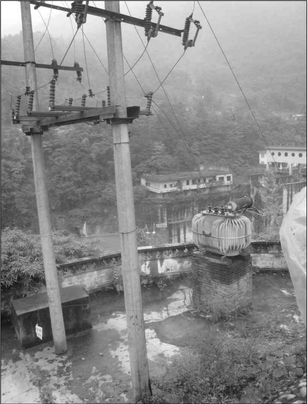
Fig. 4.77. Unanchored distribution transformer
