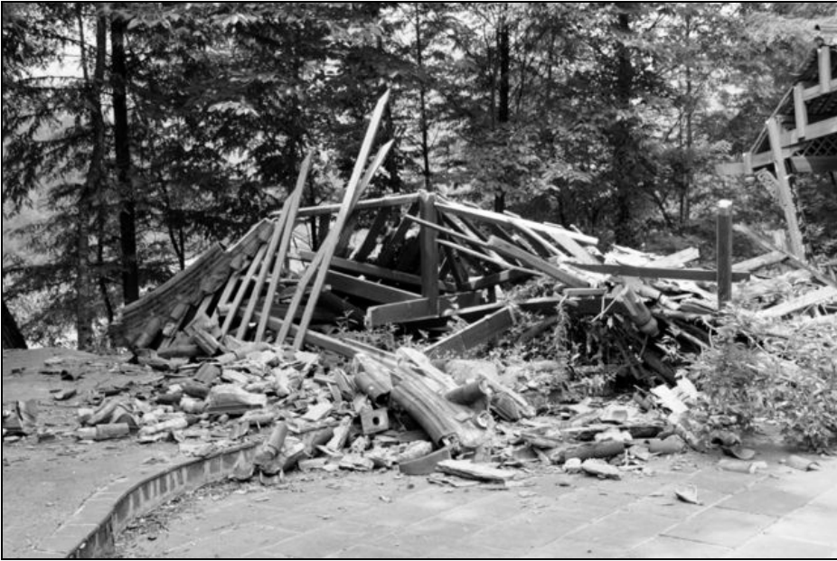
Fig. 9.32. Remains of a rest stop shelter on the road to Hongkou that was demolished by rock fall.
