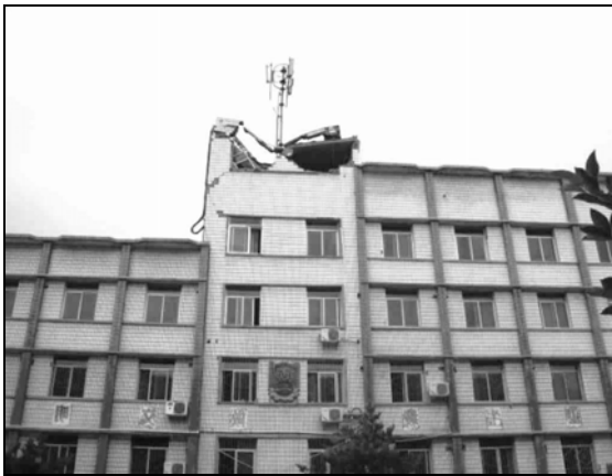
Fig. 6.22. The walls and part of the roof of this cell site in Mianzhu on the top floor of this commercial building collapsed and damaged the equipment inside. (Courtesy of IEM)
