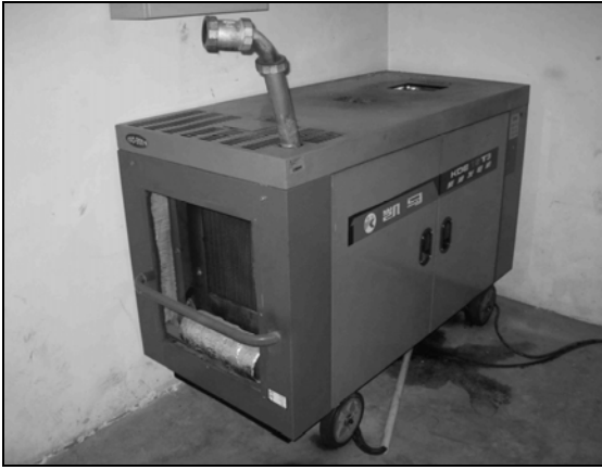
Fig. 6.15. This new power generator for the cell site was not anchored. The exhaust pipe was not connected to the outside.
