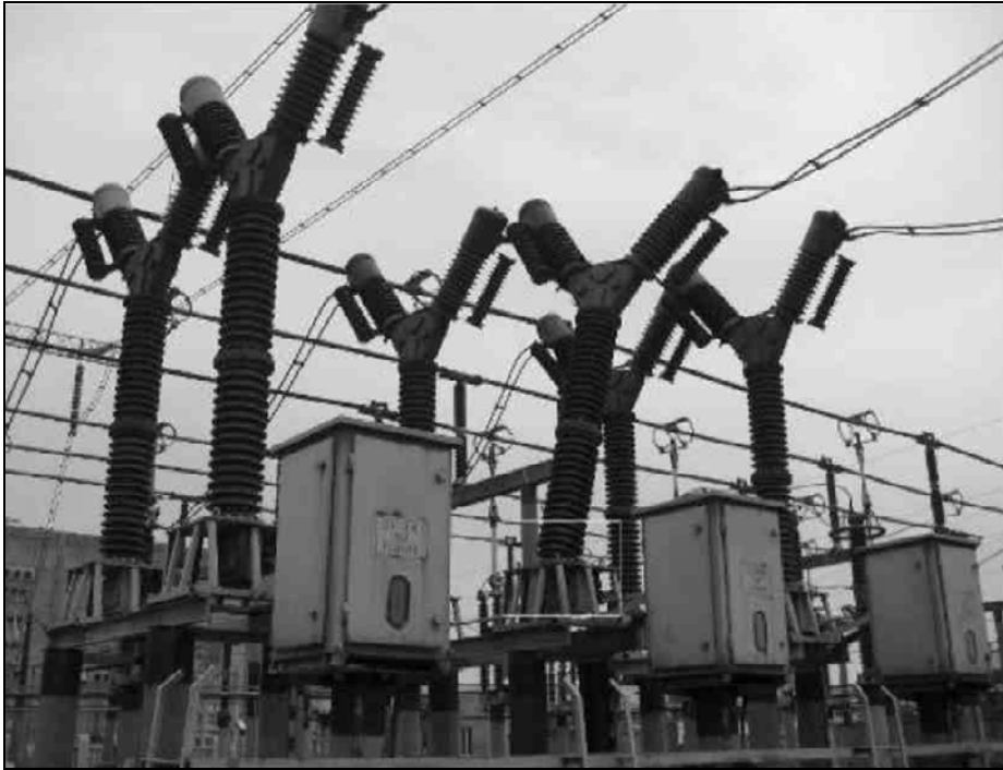
Fig. 4.43. 220 kV live tank circuit breaker damage, Yongxing Substation, Mianyang
