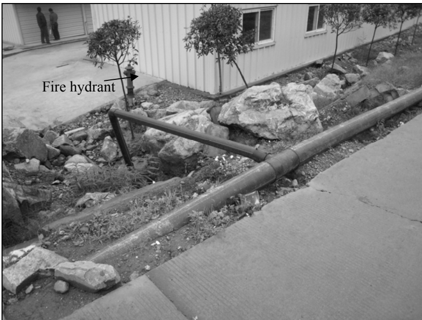
Fig. 5.7. Temporary above ground water pipe in Yingxiu for temporary shelters
