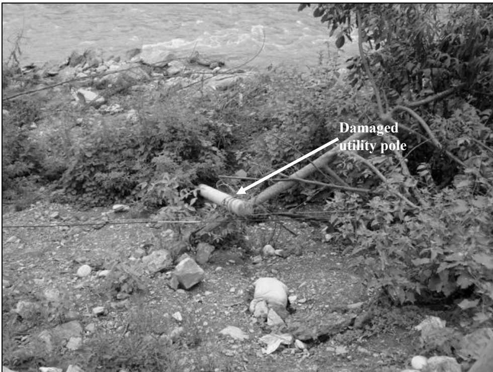
Fig. 6.47. Extensive landslides along the steep slopes of riverbank toppled many utility poles
