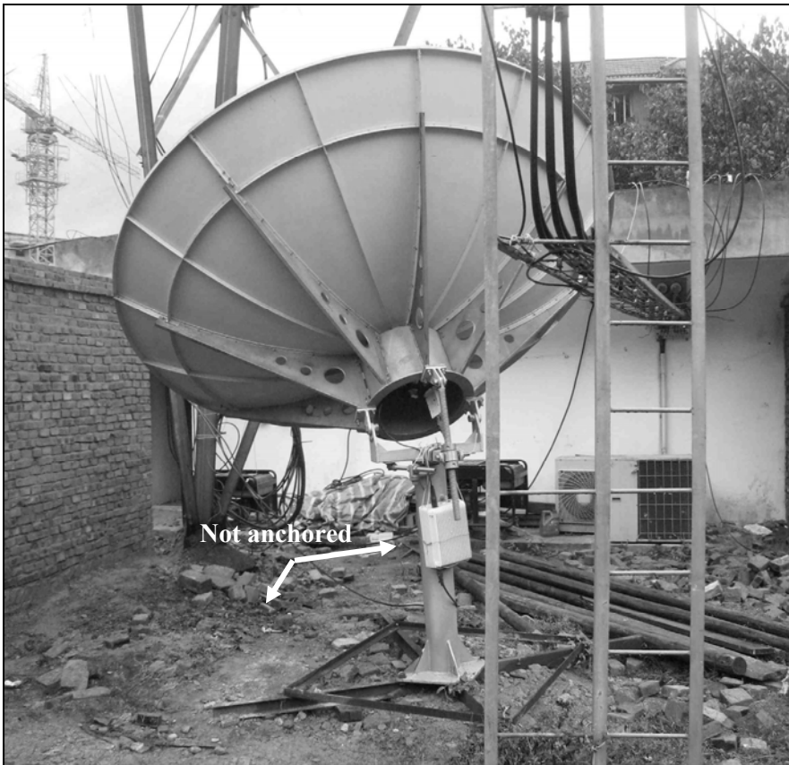
Fig. 6.17. A temporary satellite dish was used to communicate with other nodes in the network. Note that there were two portable power generators and a new air conditioning unit on the outside of the equipment building. This equipment was brought in after the building was repaired.
