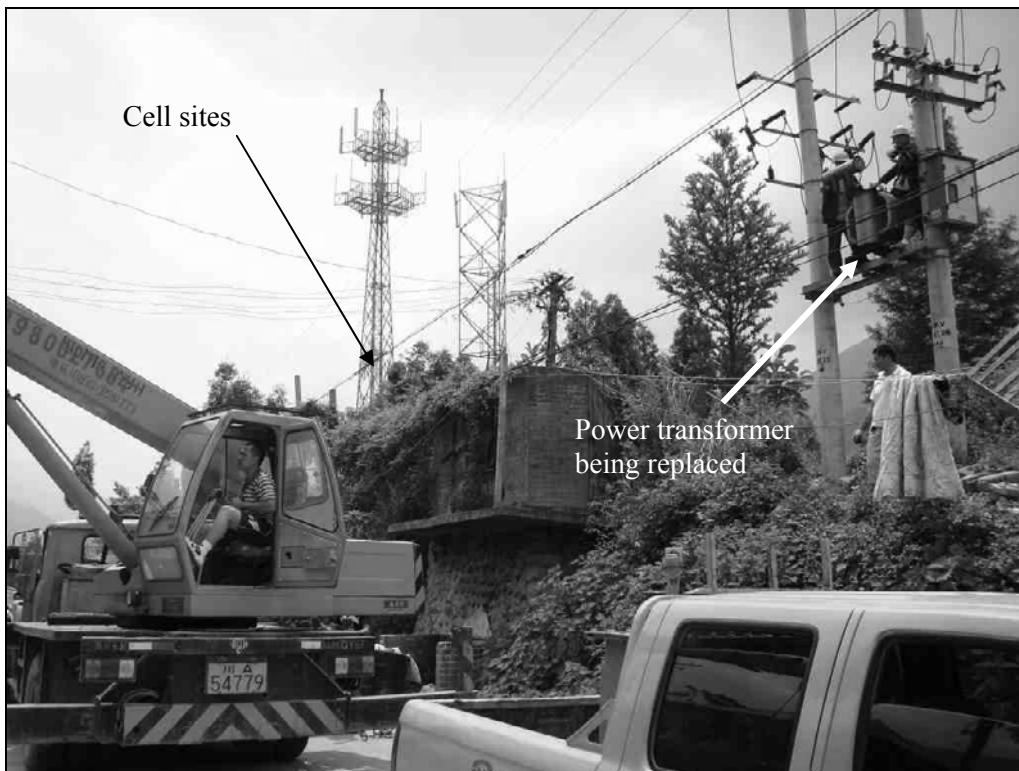
Fig. 6.7. The damaged 10-kV pole mounted transformer was being replaced during our site visit on July 17, 2008. Note the location of the cell site with towers showing.
