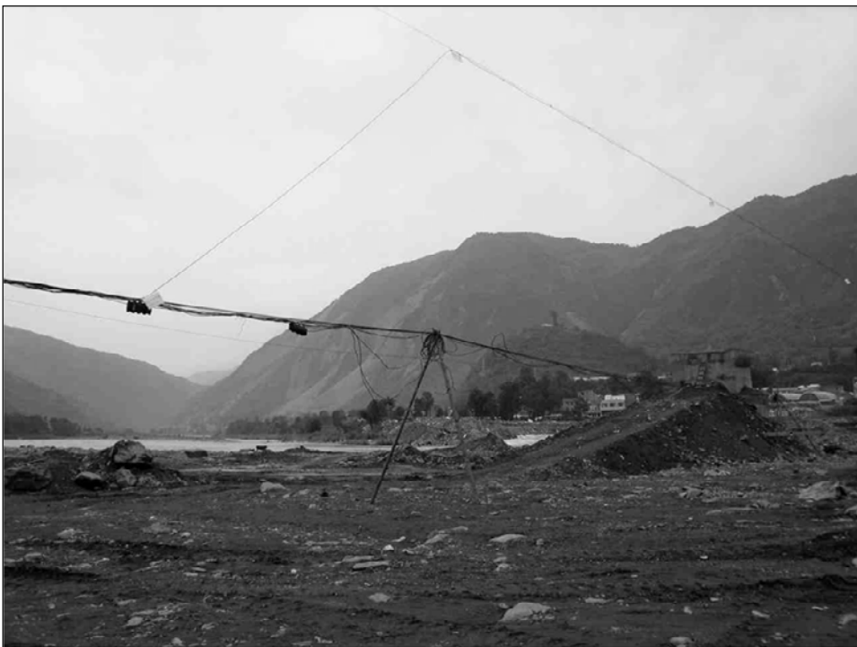
Fig. 3.63 Temporary fiber optic cables for telecommunication were installed to replaced the damaged cables due to bridge collapse (Fig 3.76)
