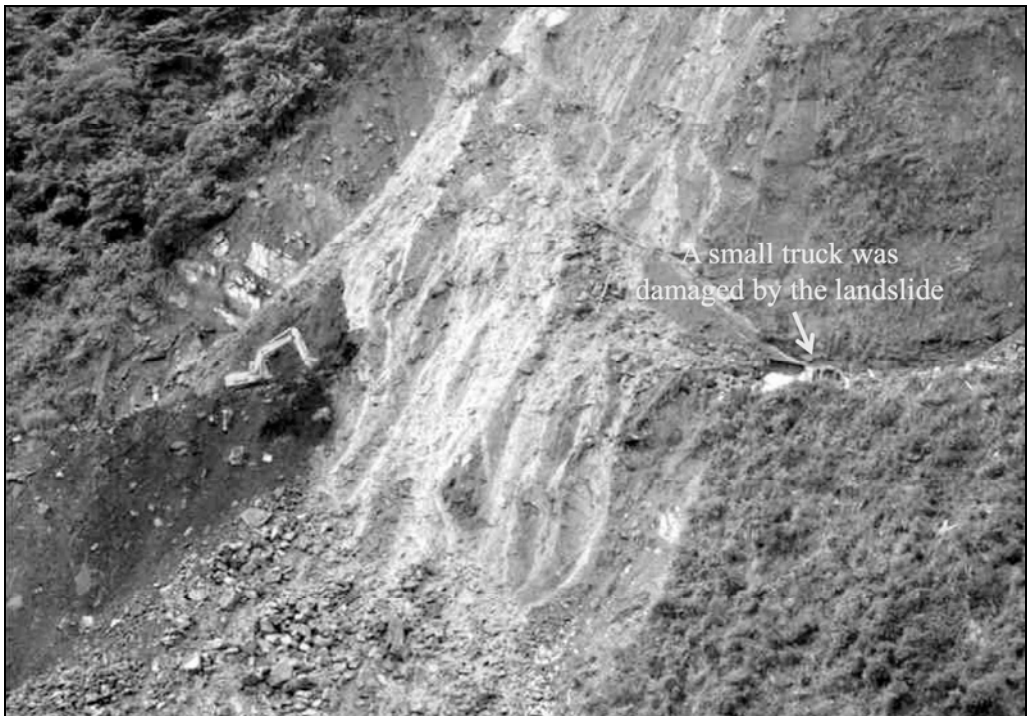
Fig. 2.24. Failed roadway due to landslide
