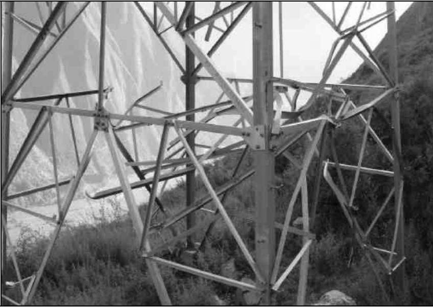
Fig. 4.66. Rack fall-impacted tower, #123, Hongxue line of Yingxiu Town
