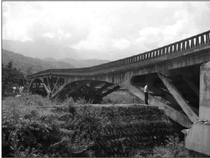
Fig. 3.49. Damaged Xiaoyudong Bridge (Longmenshan town and Xiaoyudong town)
