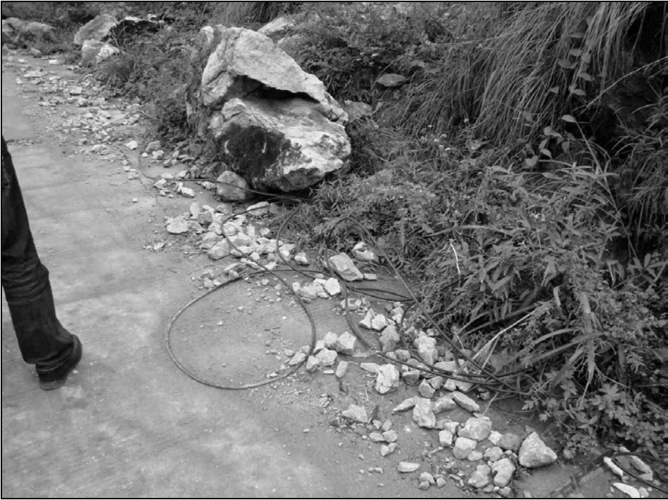
Fig. 6.57. Severed optical fiber cables were left on the side of a road. Note the size of the rock that rolled down the slope above, some cable was under it.
