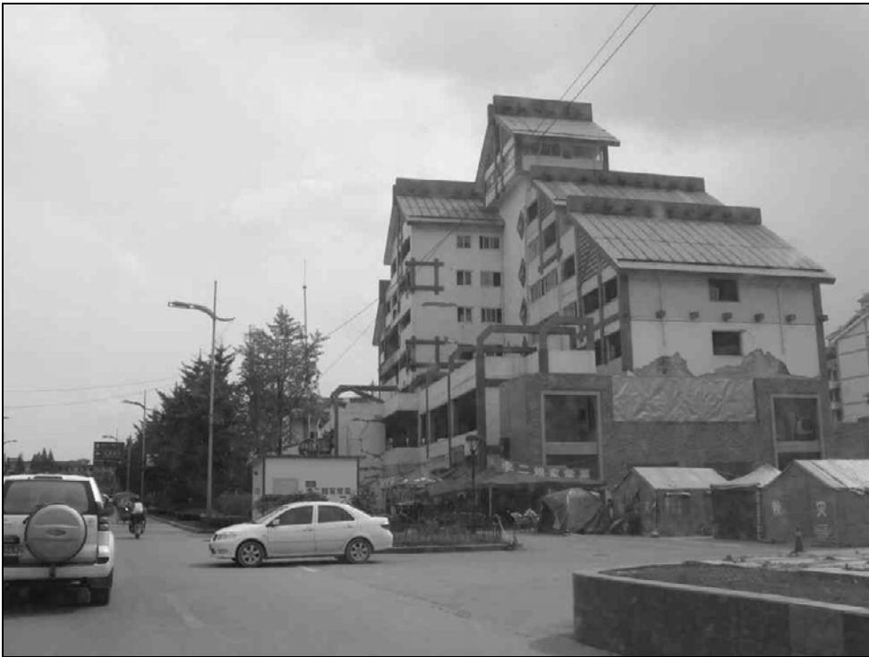
Fig. 9.53. This concrete frame building also performed well. There were stress cracks, and the plaster wall fell off the outside of the building.
