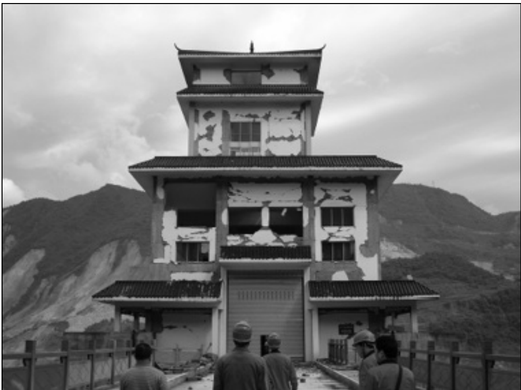
Fig. 8.6. Gate lifting equipment building sustained serious damage but did not collapse (Courtesy IEM)
