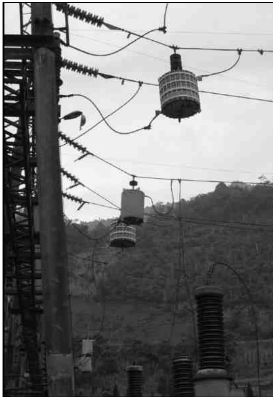
Fig. 4.22. Hanging wave traps and damage to bus connections to PTs. 15 percent of DS adjacent to hanging WTs were damaged due to pulldown
