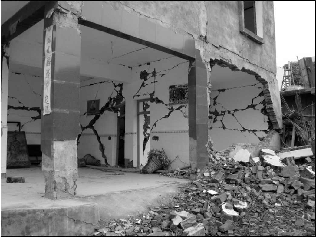
Fig. 9.90. Details of the damage to the ground floor of the building shown in Fig. 9.90
