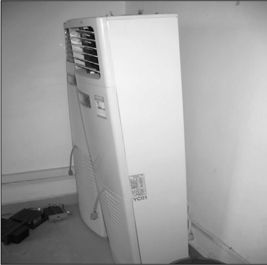
Fig. 6.34. Damaged air conditioning units. The small equipment fell from the top of the units onto the floor. (Courtesy of IEM)
