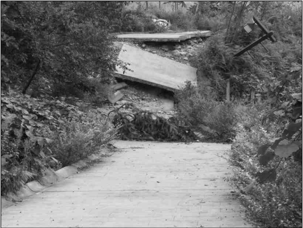
Fig. 2.26. Surface faulting through road at Gaoyan Village
