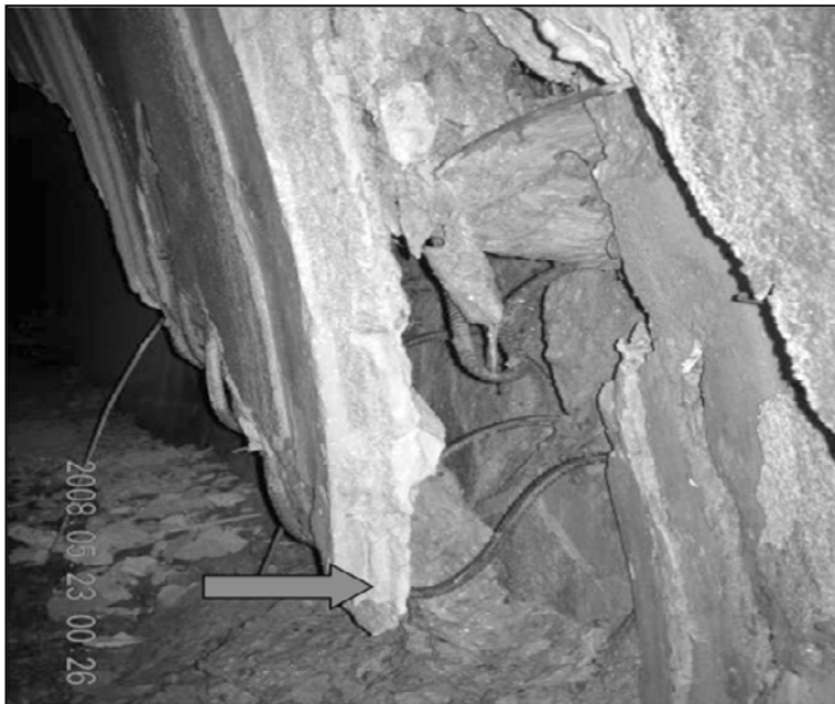
Fig. 3.76. Damage to liner, Baiyunding Tunnel (Courtesy CRSWRI)
