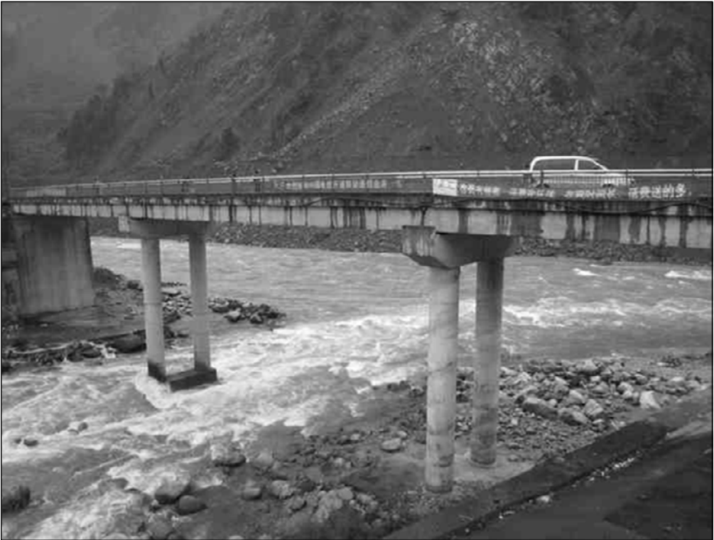
Fig. 3.39. Damaged but in-service three-span bridge at Yingxiu
