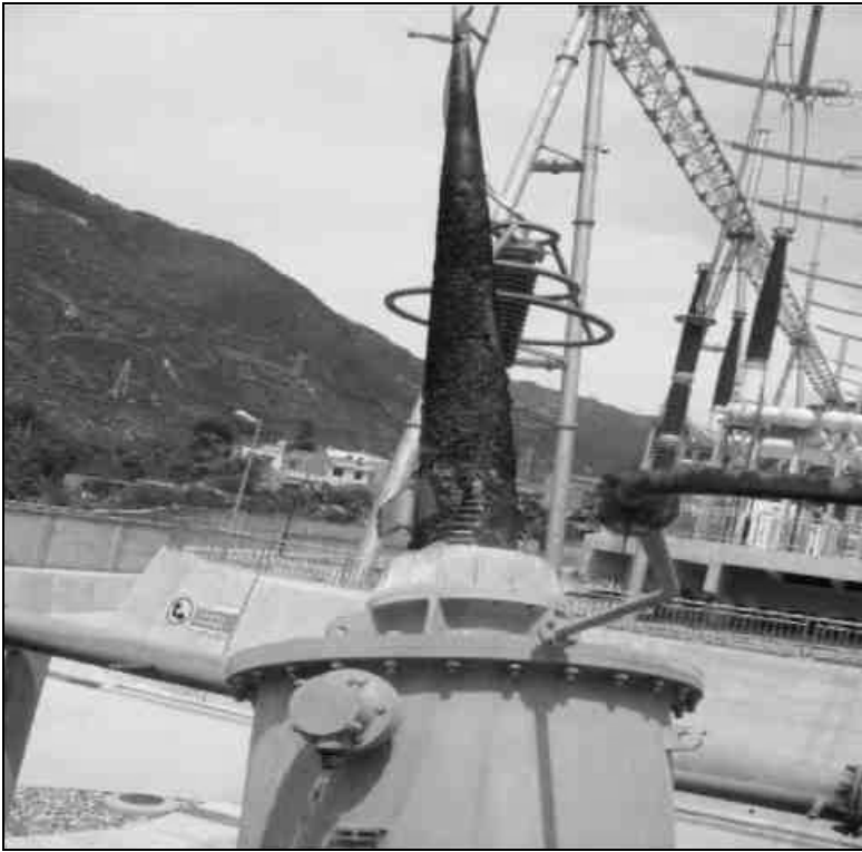
Fig. 4.14. Bushing, 500 kV transformer (Phase C burned)
