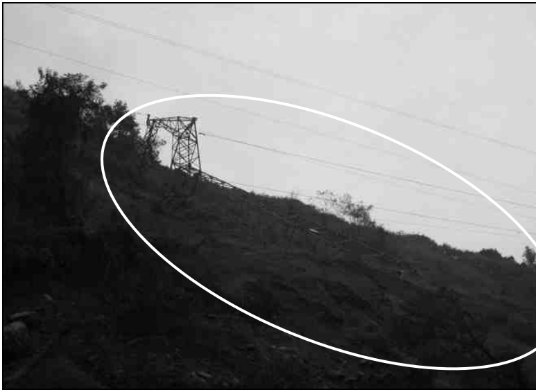
Fig. 4.60. Collapsed 220 kV transmission tower
