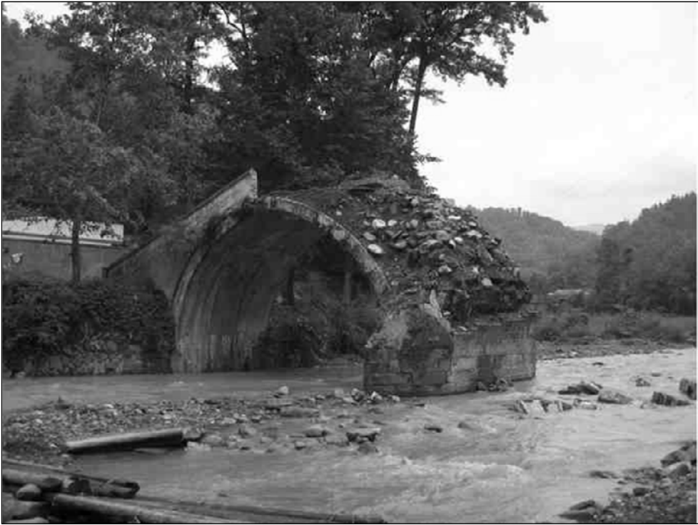
Fig. 3.53. Collapsed stone-and-earth bridge (Bailu town of Pengzhou City)
