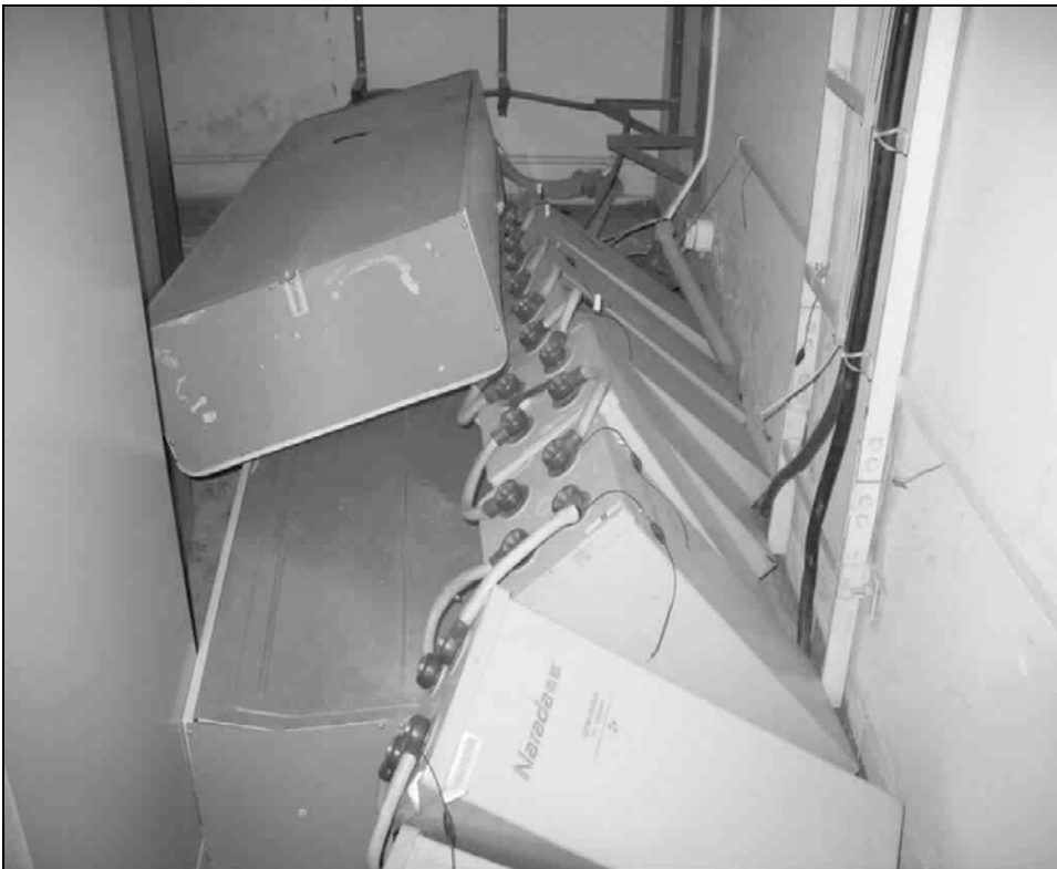
Fig. 6.33. Battery damage caused by fallen cabinets in a switching office in Dujiangyan (Courtesy of IEM)
