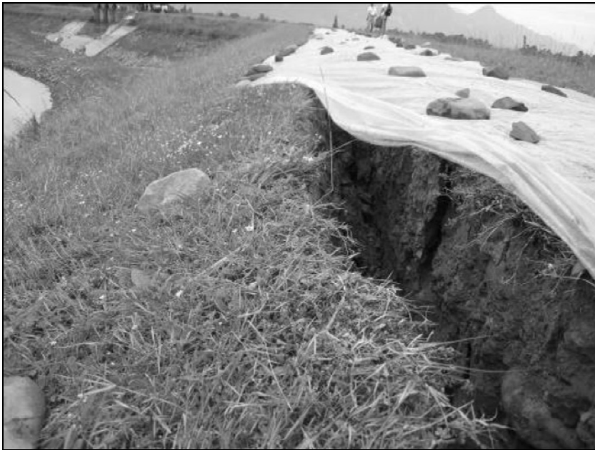
Fig. 8.14. Upstream slope movement of earthen dam, Bailin Reservoir, Hanwang Town, Mianzhu City (Courtesy IEM)
