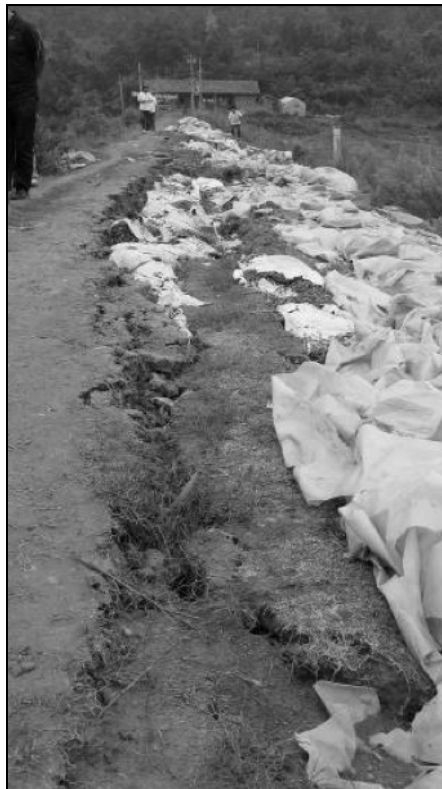
Fig. 8.12 Longitudinal cracks at crest of earthen dam, Changdaogou Reservoir, Mianyang City (Courtesy IEM)
