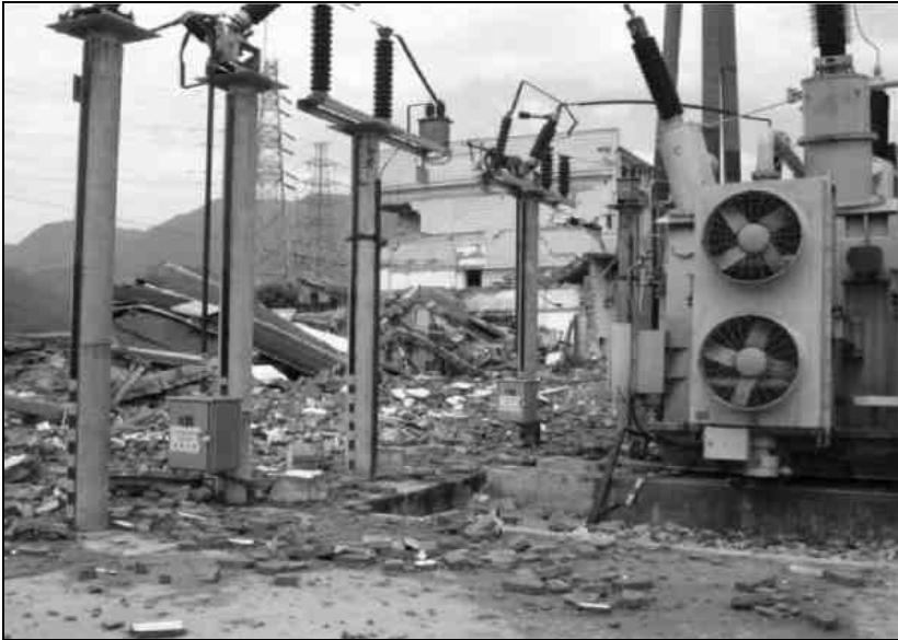
Fig. 4.13. Collapsed control building
