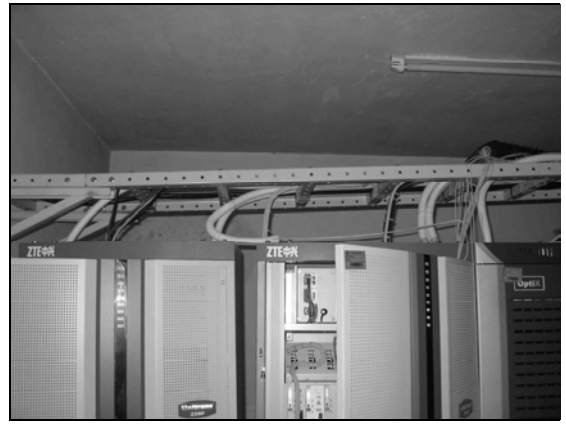
Fig. 6.14 New cable rack above the base station controllers
