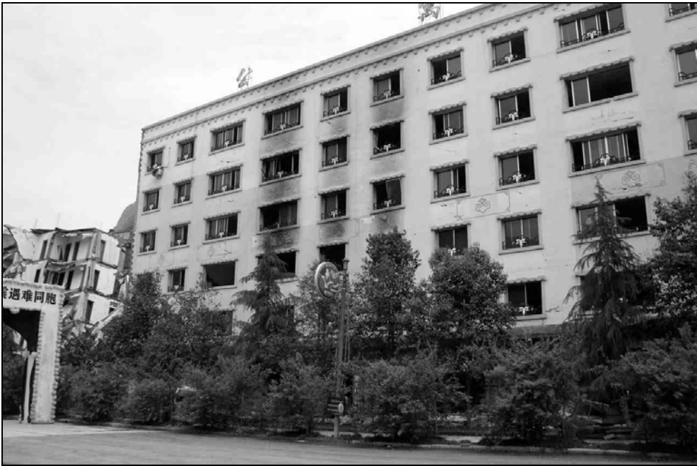
Fig. 9.31. Soot marks the location of a fire, which most likely started on the third floor.
