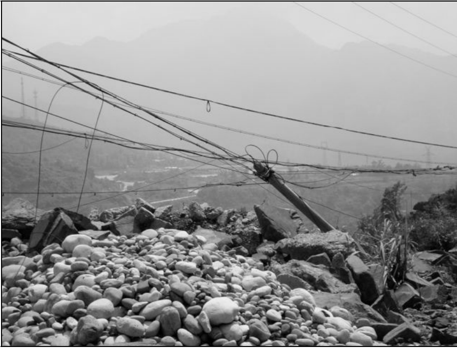
Fig. 6.35. Damaged utility pole on the road to Yingxiu and a close look at the cables, which are all optic fiber cables.
