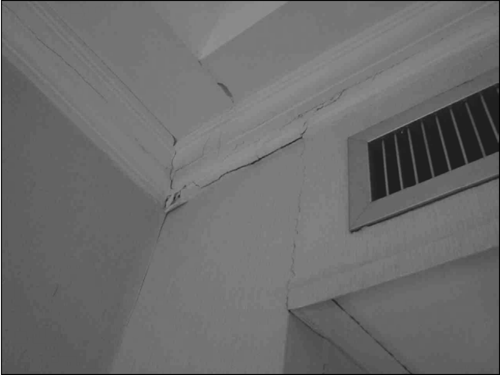
Fig. 9.68. Cracks on walls inside the hotel rooms were evident of strong shaking in this city.
