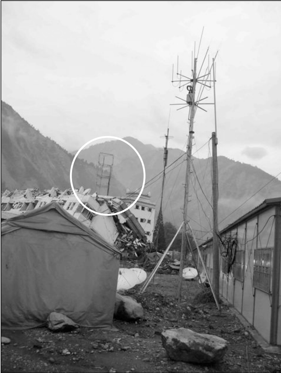
Fig. 6.18. Cell site antennae tower (circled) slanting about 10° from its vertical position. It might be leaning against one of the collapsed buildings.
