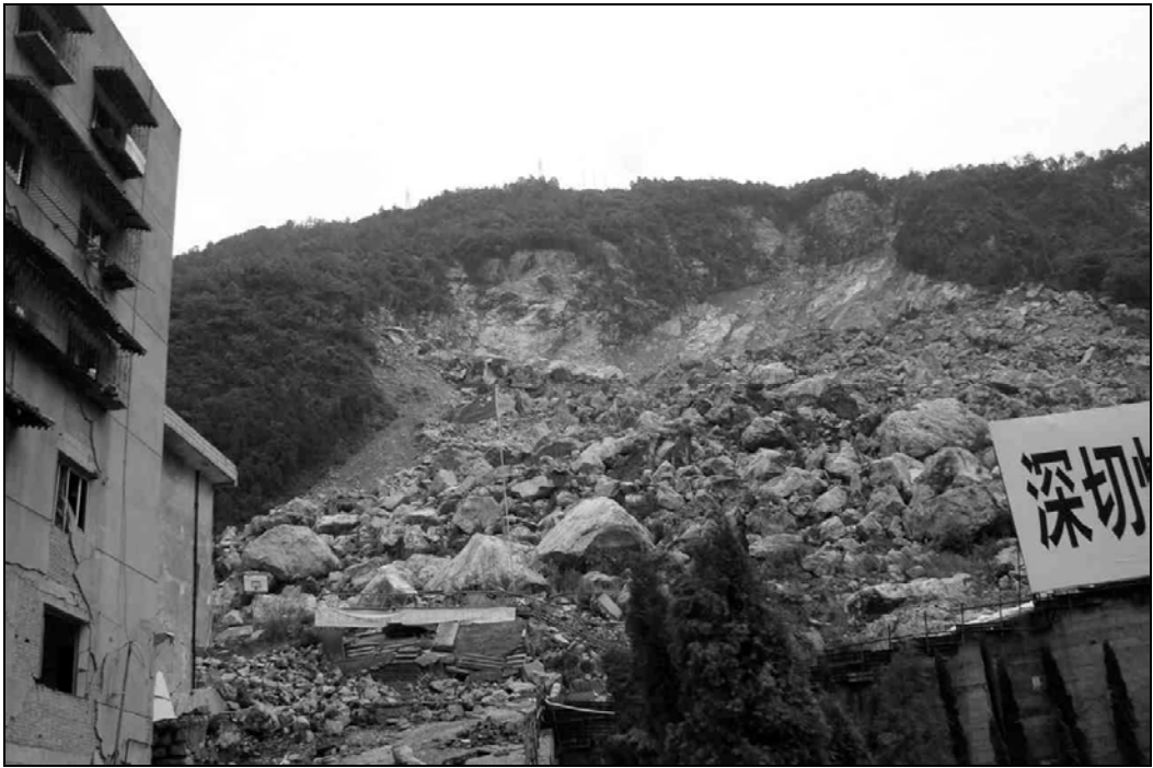
Fig. 9.19. The buildings along this foothill are under the pile of rock that fell from the top of the hill.
