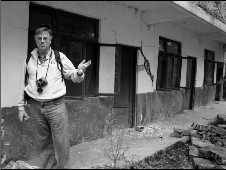
Fig. 9.42 The front of the building in Fig. 9.42 shows significant structural damage; however, it did not collapse.
