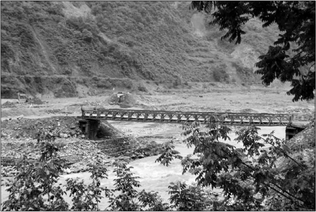
Fig. 3.58. The temporary bridge built by the PLA was simply supported on both ends
