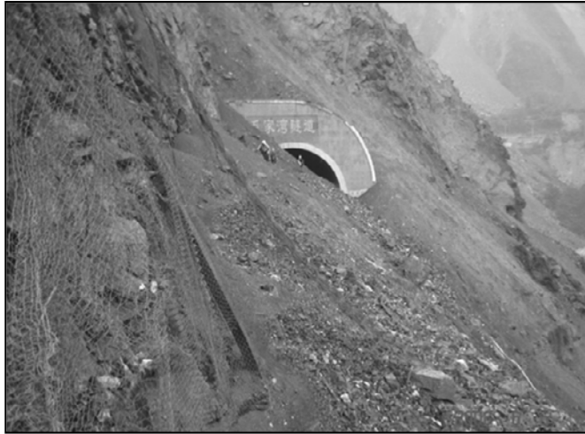
Fig. 3.71. Portal landslide, Maojiawan Tunnel in Duwen (Courtesy CRSWRI)
