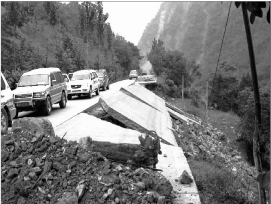
Fig. 3.5. A landslide carries a roadbed downhill near Pengzhou
