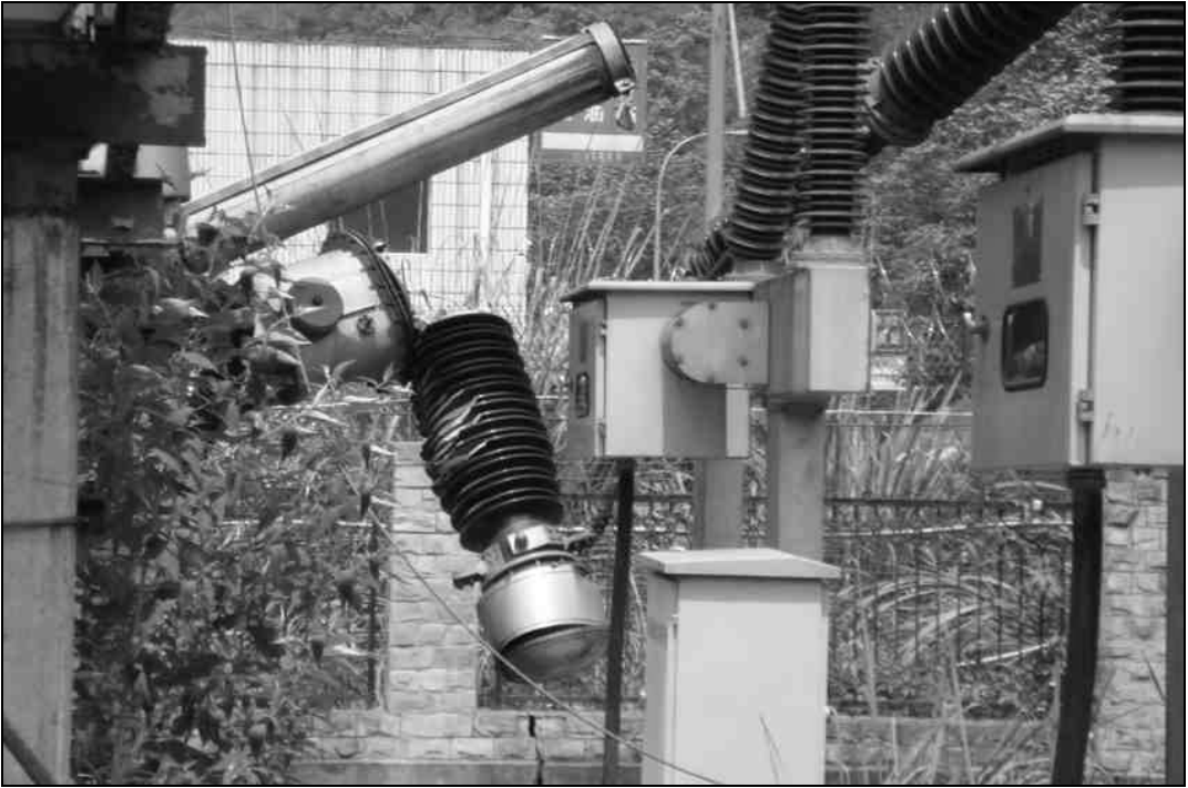
Fig. 4.35. Damage to Beichuan substation, 110 kV (May, 2009 photo)
