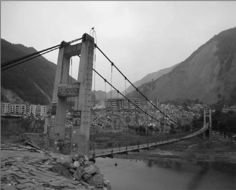
Fig. 3.55. Beichuan Bridge after the Wenchuan Earthquake
