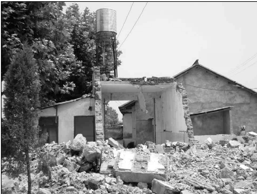
Fig. 5.14. Local storage tank atop damaged URM structure (Shifang)
