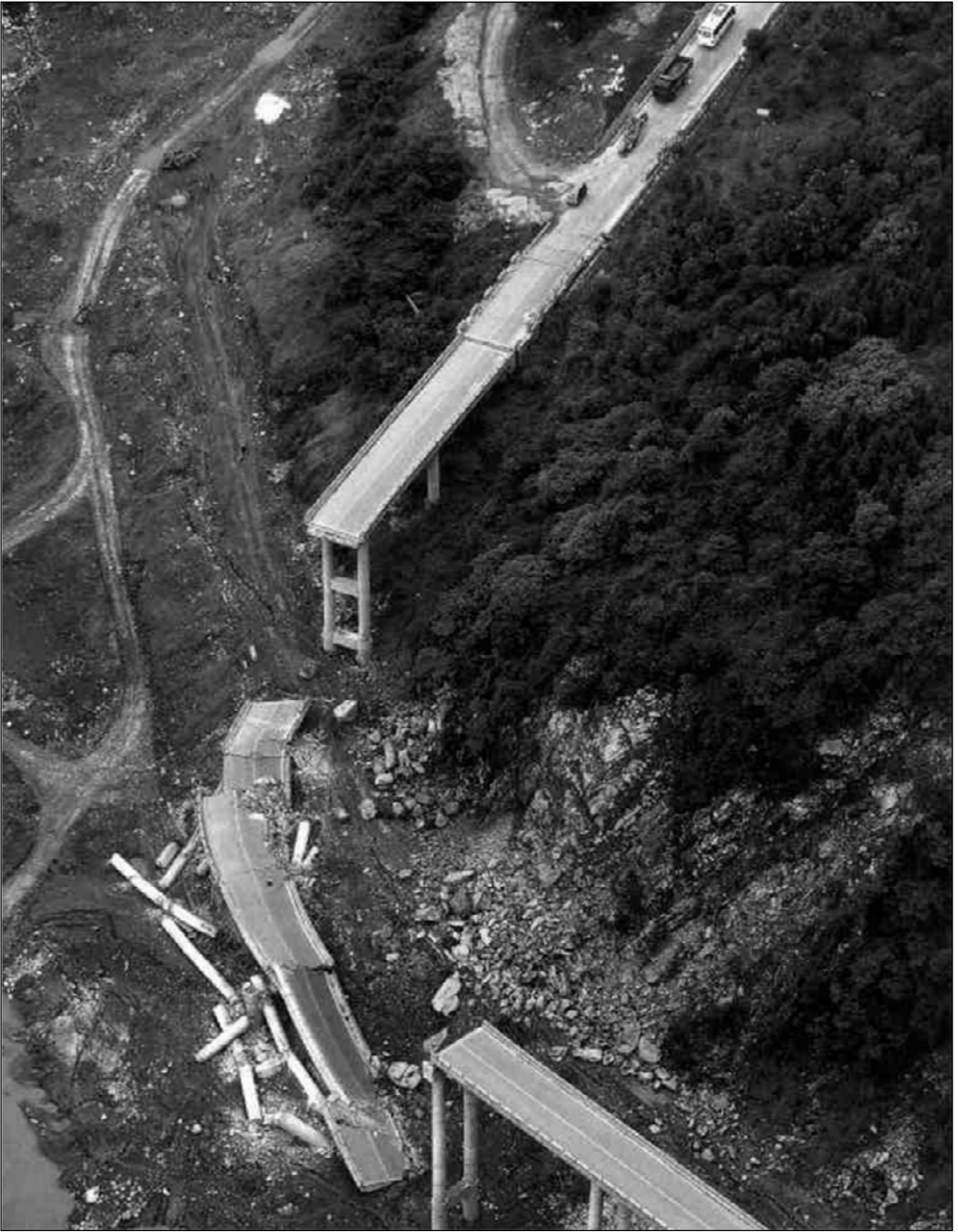
Fig. 3.42. Collapsed Baihua Bridge
