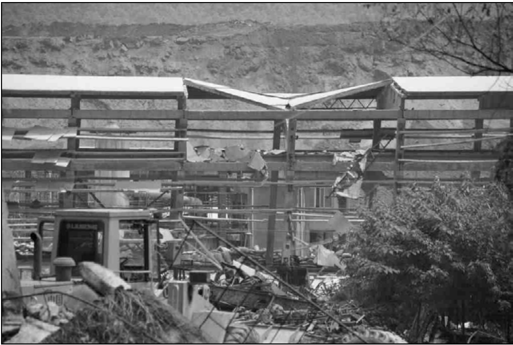
Fig. 9.77. Extensive damage at another chemical processing plant in Shifang.
