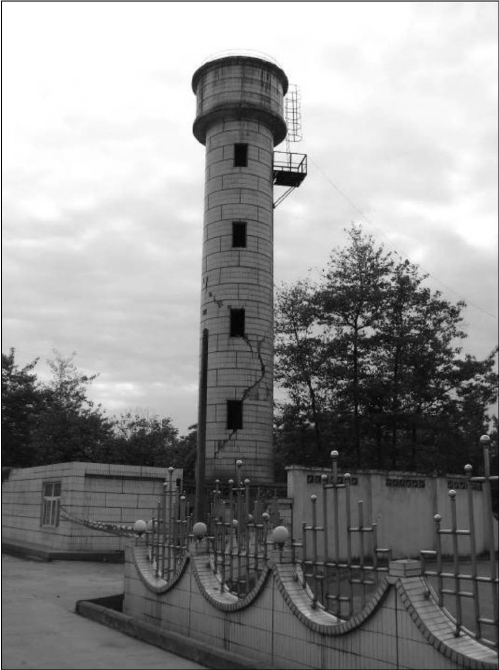
Fig. 5.12. Elevated concrete water tank with heavy damage to tower
