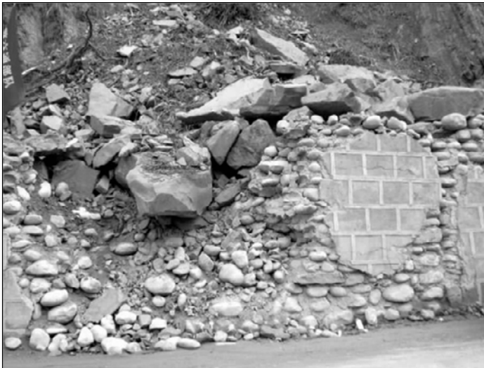
Fig. 3.19. Typical retaining wall failure along roads in Sichuan
