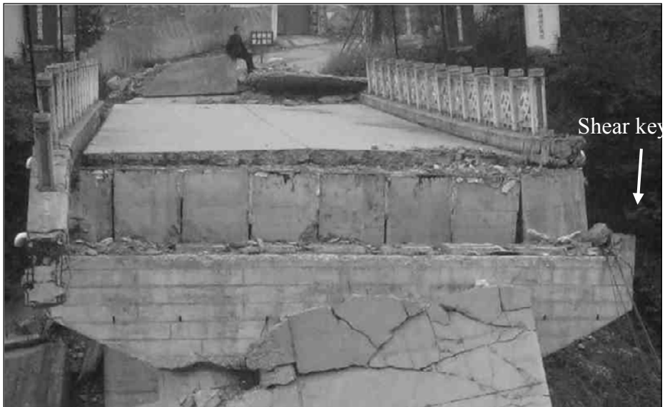
Fig. 3.48. Close up view of Gaoyuan Bridge's failed span (Hongkou)
