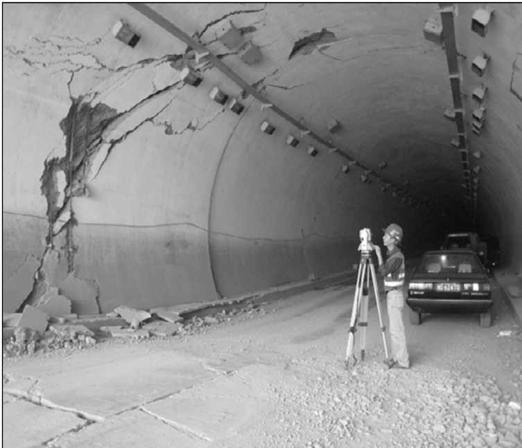
Fig. 3.84. Liner damage (Courtesy CRSWRI)
