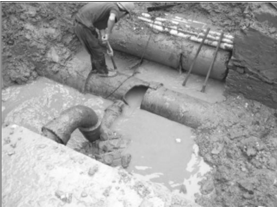
Fig. 5.9. Damaged cast iron pipe, Mianzhu
