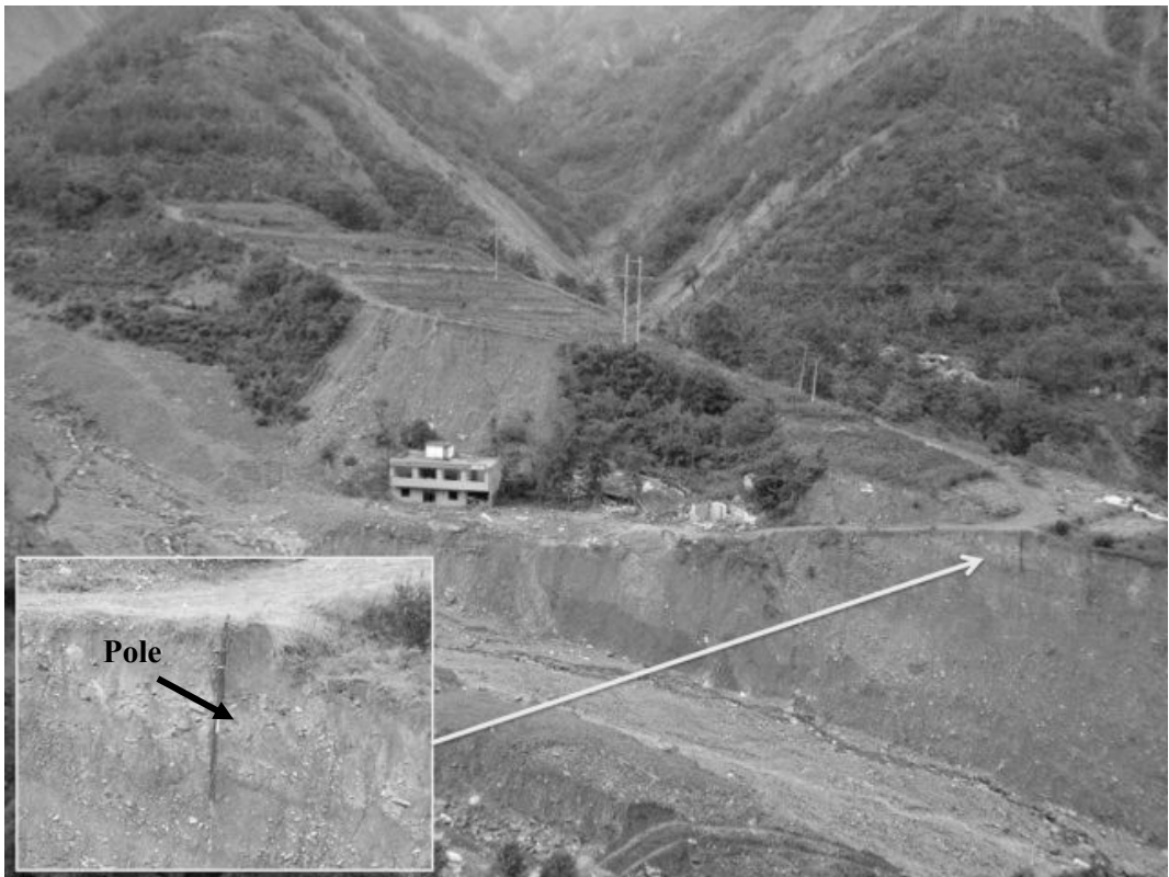
Fig. 6.54. Due to landslide a pole was hanging by the cables along the edge of the slope failure.
