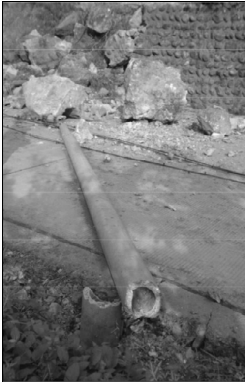
Fig. 3.13. Colocation damage, such as the retaining wall and telephone pole blocking access to the roadway, is very common after earthquakes
