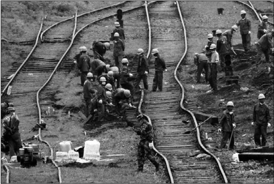
Fig. 3.86. Soil liquefaction damage to tracks (Courtesy of Prof. Mei and Dr. Zhang)
