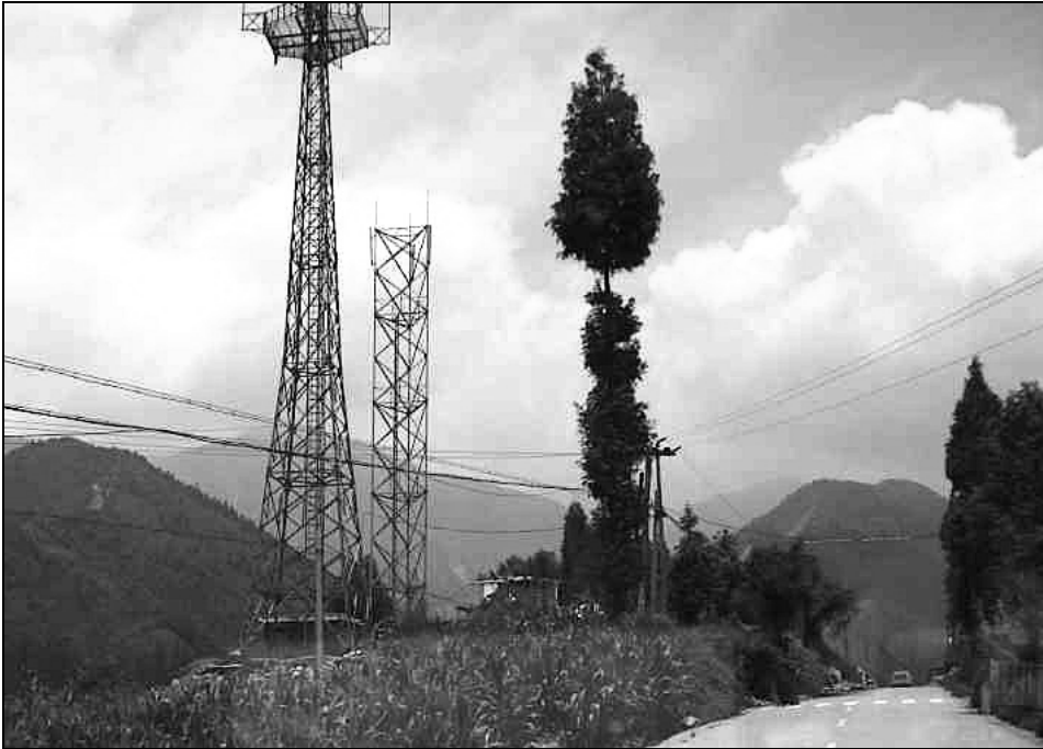
Fig. 6.1. Hongkou cell sites: the taller tower belongs to China Mobile, the other to China Telecom.
