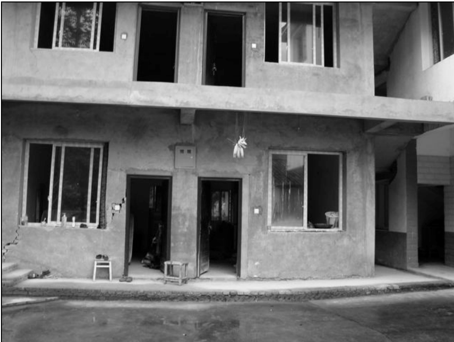
Fig. 9.44. This new building on the north side of the court yard showed some minor cracks. The second floor was not yet occupied, and the railing had not been installed.
