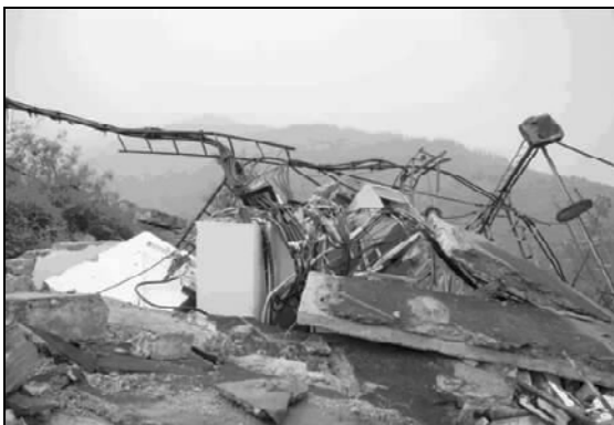
Fig. 6.24. This cell site building in Jianshi, Shifang, collapsed and damaged all the equipment inside. (Courtesy of IEM)
