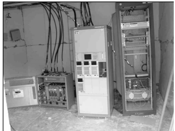
Fig. 6.3. New equipment was temporarily installed to restore service
