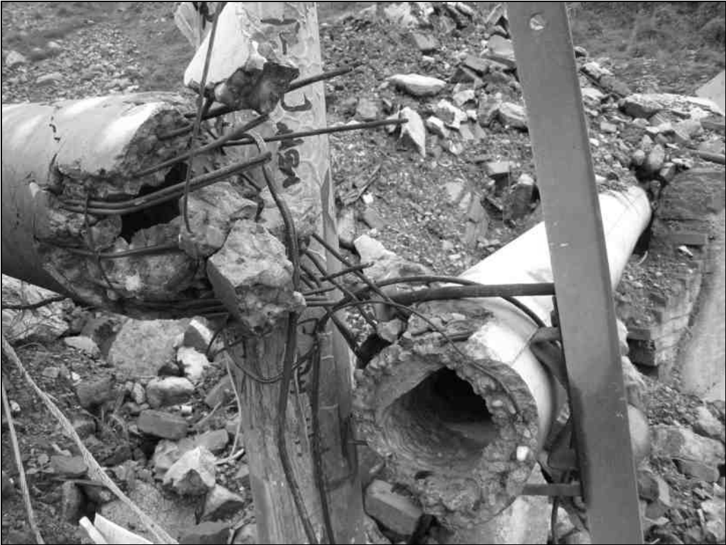
Fig. 4.71. Collapsed 10 kV distribution pole (10-in. diameter, 2.5-in. wall thickness)
