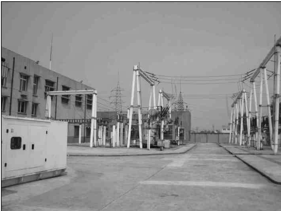
Fig. 4.9. 110 kV substation located between Deyang and Shifang
