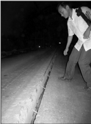
Fig. 3.82. Vertical movement damage to road surface in the tunnel (Courtesy CRSWRI)
