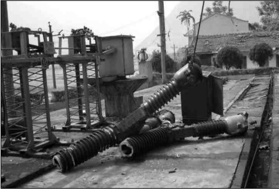
Fig. 4.41. Live tank breaker damage, Yuanmenba Substation
