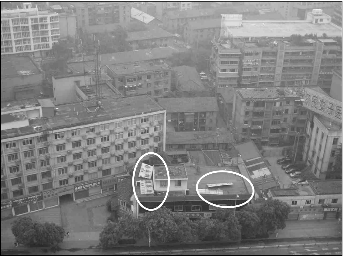
Fig. 9.72. A few large advertisement signs fell on the roof of this building in Chengdu.
