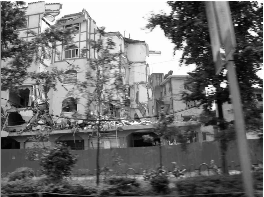
Fig. 9.56. More than one-third of this five-story apartment building collapsed. The remaining structure was condemned as unsafe.
