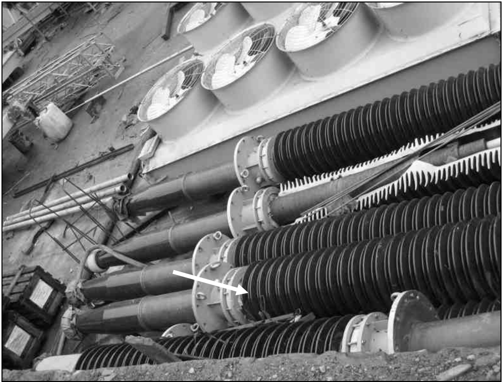
Fig. 4.29. Slipped porcelain bushing is fourth from top
