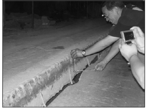
Fig. 3.81. Upheaval damage by 70 cm (Courtesy CRSWRI)
