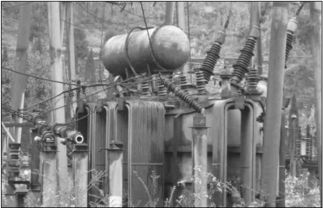
Fig. 4.19. Damage to current voltage transformer (CVT) and three lighting arrestors
