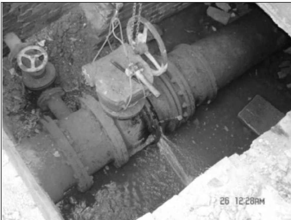
Fig. 5.10. Damaged cast iron pipe, Guangyuan City
