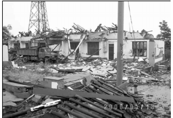
Fig. 6.25. The roof of this cell site building in Wudu, Shifang, collapsed on the equipment inside. (Courtesy of IEM)
