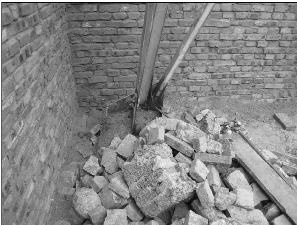
Fig. 6.10. Bricks from the damaged wall all over the yard under the tower
