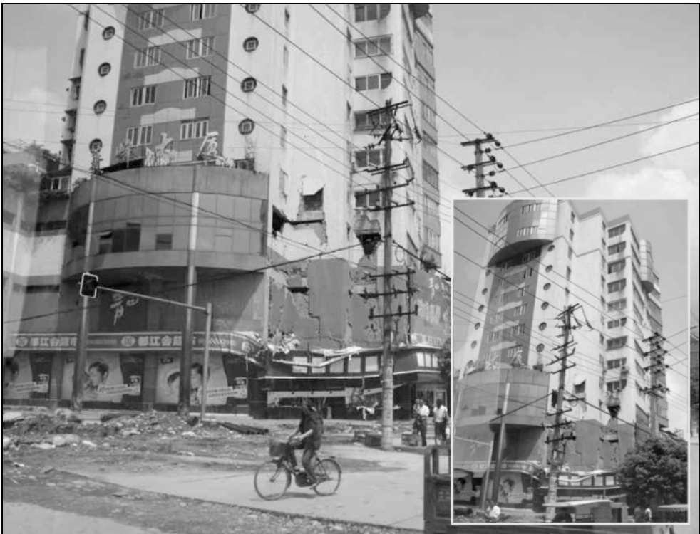
Fig. 9.58. The second and third floor of this apartment building is a shopping mall with a high ceiling, creating a soft-floor effect. Most of the damage is on these two floors. Note the windows above are not damaged.
