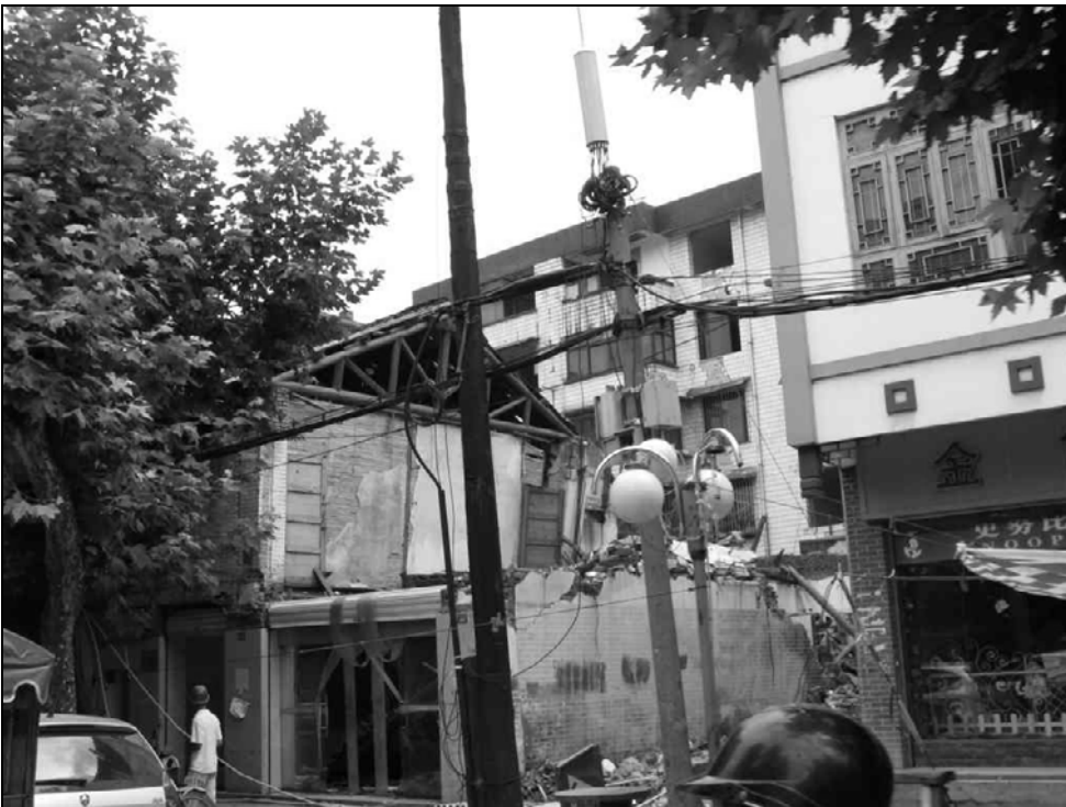
Fig. 9.54. A two-story URM building collapsed. The building behind and next to it sustained minor damage. A window was broken on the top floor the building in the background.
