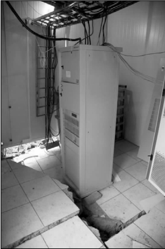
Fig. 6.26. The concrete floor of this cell site in a metal panel building in Dujiangyan cracked causing equipment failures. (Courtesy of IEM)
