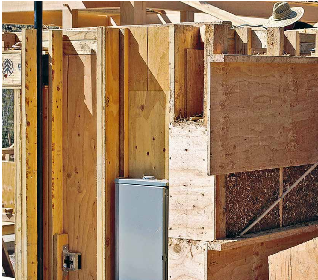
Vent stack tucked into window buck. Electrical panel chase shown beside it.
