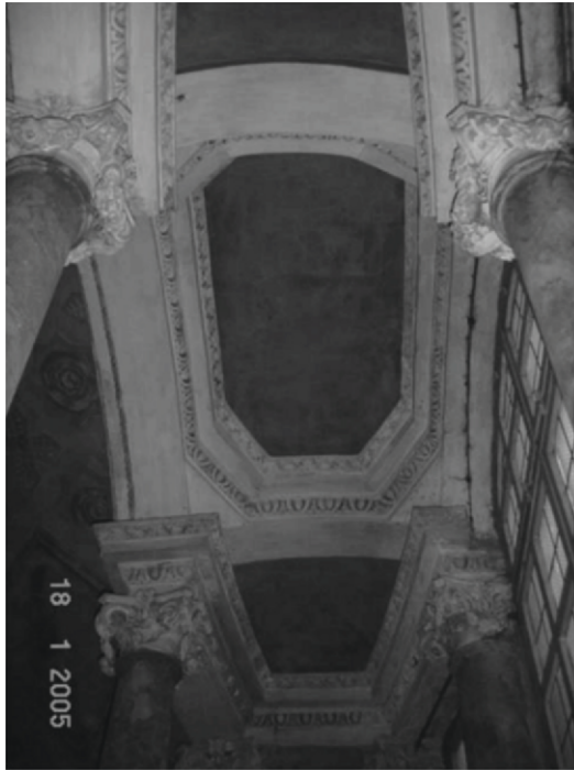
Fig. 25. View from underneath of the small reinforcing vaults built in the lenticular structure of the Serlian window
