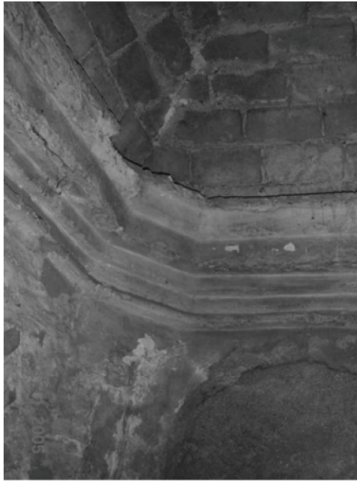
Fig. 27. Inside the double structure (no longer visible from the main space of the church); note the moulded cornice, finished because it was exposed to view
