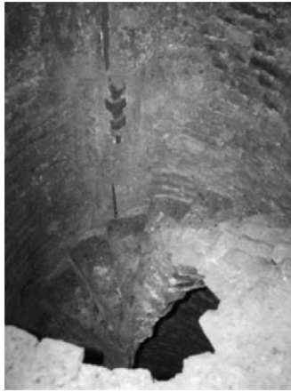
Fig. 15. Spiral stairway inside the corner tower where the vertical bar that acts as a hinge and connection between two tie-rods and the insertion of bolts to put them in tension can be seen, as shown in the detail of drawing no. 295/1 shown in fig. 14
