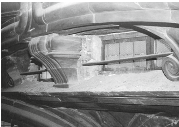
Fig. 20. Detail showing “point of contact” between the keystones of the arches and the modillions which are actually separated by a layer of poor quality masonry
