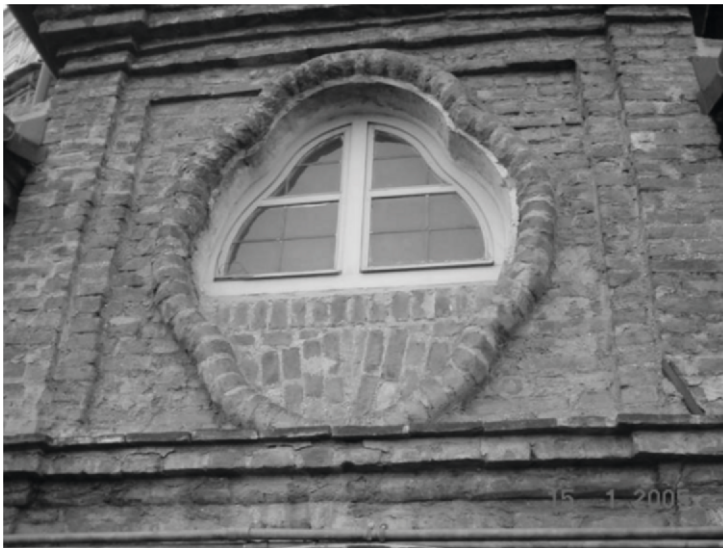
Fig. 26. Photograph of the exterior facade of the space over the Serlian window; note the obstruction of the lower part by the reinforcing vault
