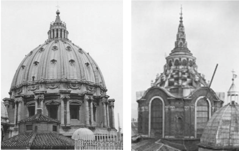
Fig. 8. The masonry ring that usually resists the outward thrust of a dome. Comparison of the dome of St. Peter's (left) with that of the Chapel of the Holy Shroud (right), where the masonry ring is interrupted by the arches of the large windows (indicated by the arrow)
