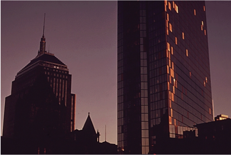
Figure 1: Window breakage on the facade of Boston’s John Hancock Tower in the mid-1970’s
