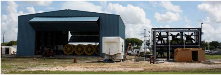
Figure 1. New 12-fan WoW (under construction) beside the 6-fan WoW (on the right) at FIU.
