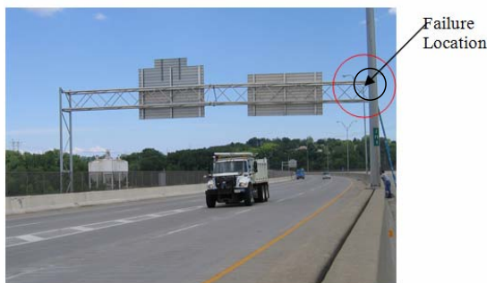
Figure 3: The failure location of the sign support structure
