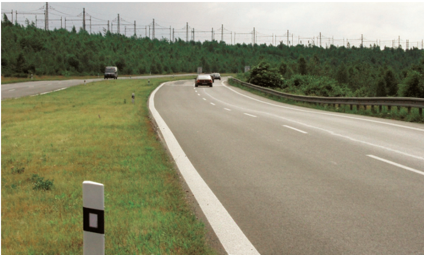
Fig. 8.22 Ervěnice corridor – photo of motorway with visible signs of differential settlement
