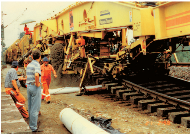
Fig. 6.75 Photo of reconstruction technology without removing rail grid; application of reinforcing geosynthetics
