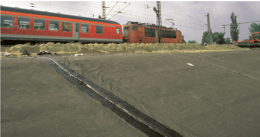
Fig. 6.87 Photo of GCL installation to protect environment from spillage from. (a) Road. (b) Railway
