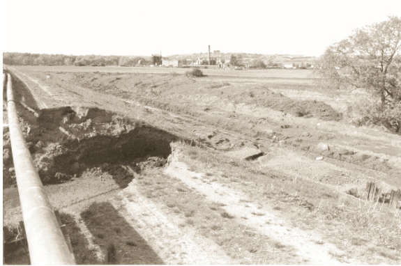
Fig. 8.33 The gash in the main dam constructed from ash
