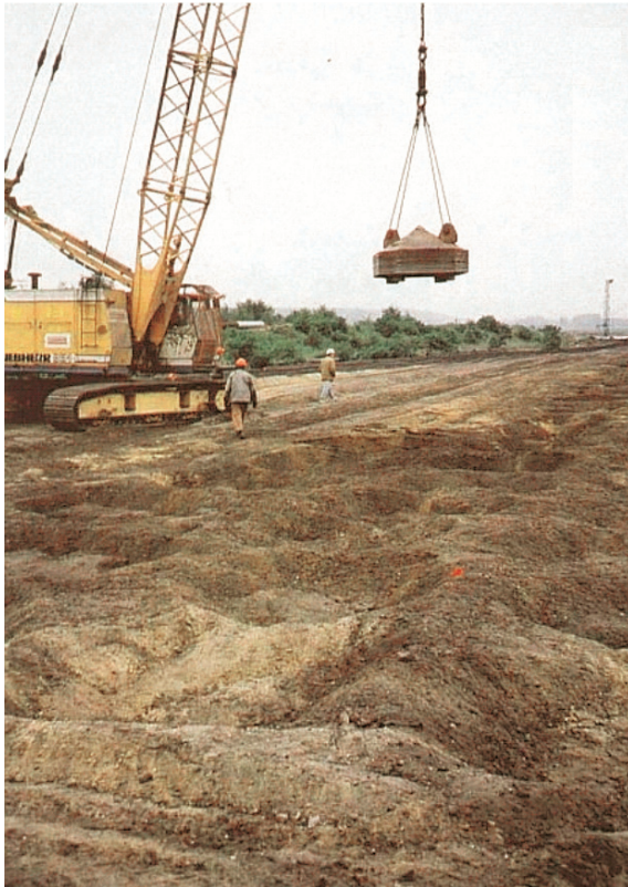
Fig. 8.76 Application of dynamic consolidation. (a) Compaction performance. (b) “Ironing” stage of compaction
