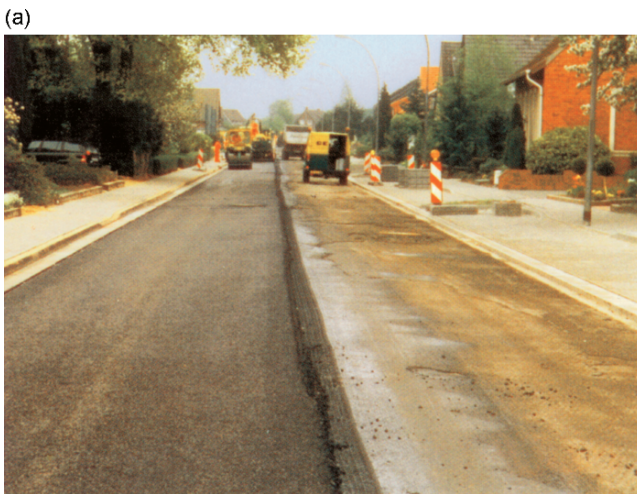
Fig. 6.68 Photos of road before treatment with asphalt reinforcement and after 7 years of use (according to Elsing)
