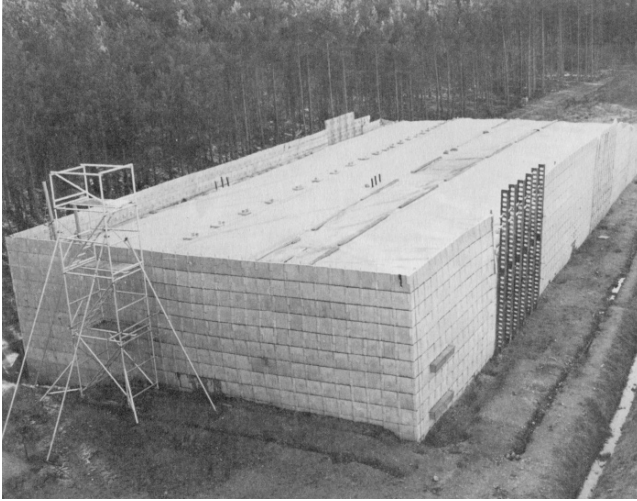
Fig. 5.64 Full scale structure at completion of the second stage (according to Boden et al.)
