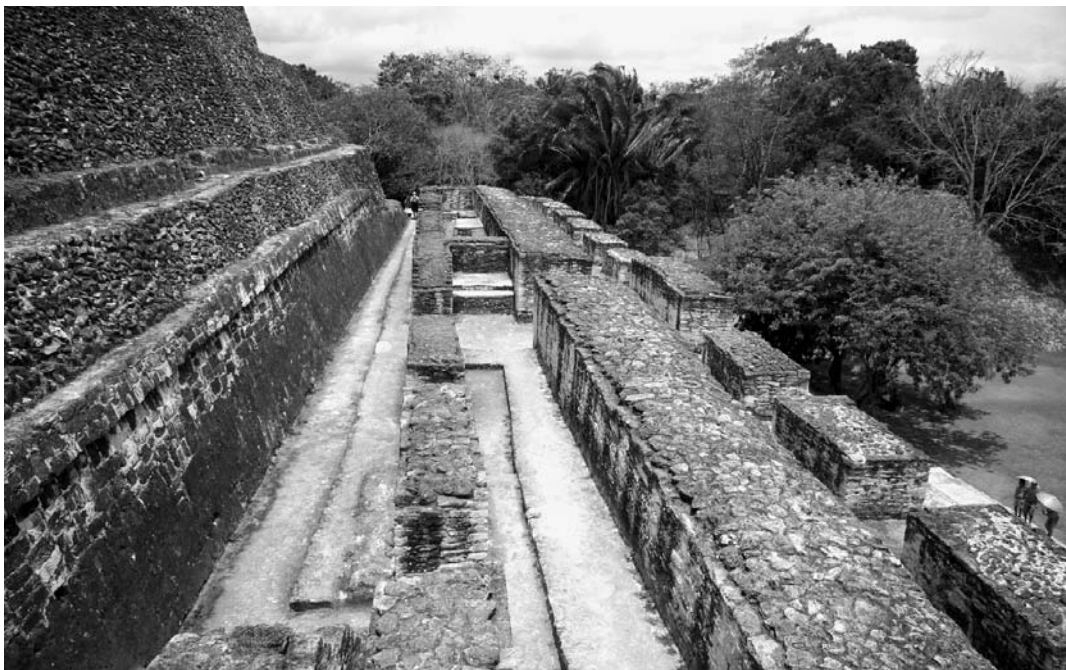
Figure 2.3. Structure A-32 on the north face of the Castillo at Xunantunich, facing west. Note the thickness of the spinewall in comparison to the two outer walls on this once vaulted building (photograph by the author).
