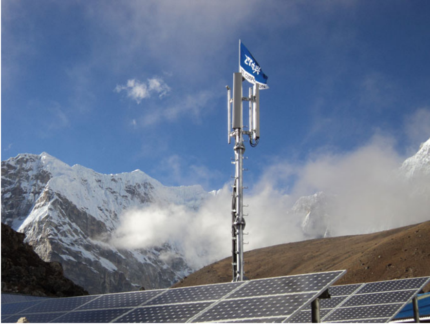
Fig. 2.17 ZTE's highest altitude 3G-communication tower
