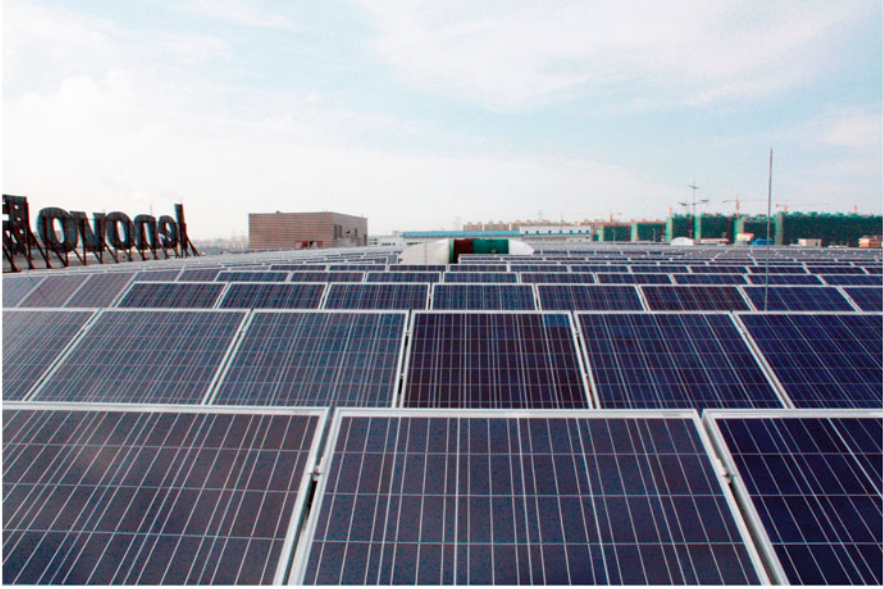
Fig. 2.14 Lenovo's Shanghai golden sun photovoltaic system project
