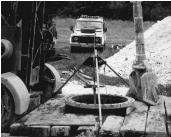
Figure 6.18 Photograph of the geophysical logging of a Chalk well in Southern England. Note the chisel of the cable-tool percussion drilling rig. Note also the logging cable emerging from the front of the vehicle and running over a pulley into the well. Photo by David Banks
