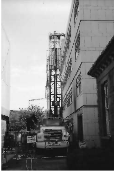
Figure 1.5 Drilling rig being set up for constructing a well in a gravel aquifer used as a source of geothermal energy, Dublin, Ireland. Photo by Bruce Missteart
