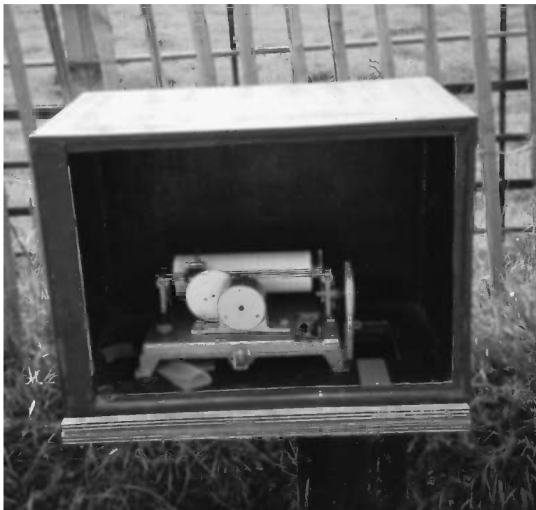
Figure 7.5 A float-operated clockwork chart recorder for groundwater level monitoring, mounted on top of an observation borehole in the Chalk aquifer at the Gatehampton site, southern England. A chart recorder such as this will have produced the hydrograph shown in Figure 7.22. Photo by David Banks
