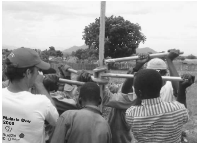
Figure 3.26 Removal of pump rods during hand-pump maintenance, Lower Nile province, Sudan. Photo reproduced by permission of Laurence Gill
