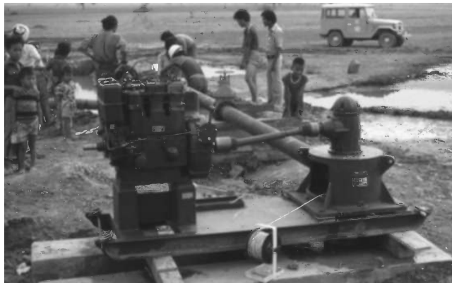
Figure 3.19 A vertical turbine pump installed in an irrigation well in Myanmar. The diesel prime mover is connected to the pump by a right-angle gear drive. This pump installation is temporary for the purpose of a pumping test. Photo by Bruce Misstear
