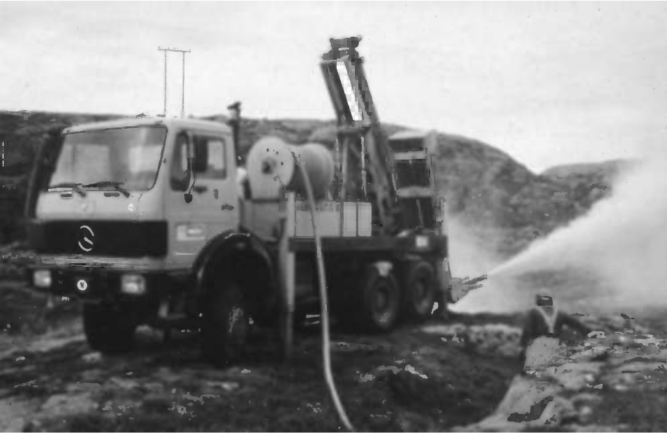
Figure 5.17 An inclined borehole being drilled by the DTH hammer method, Norway. Photo by David Banks
