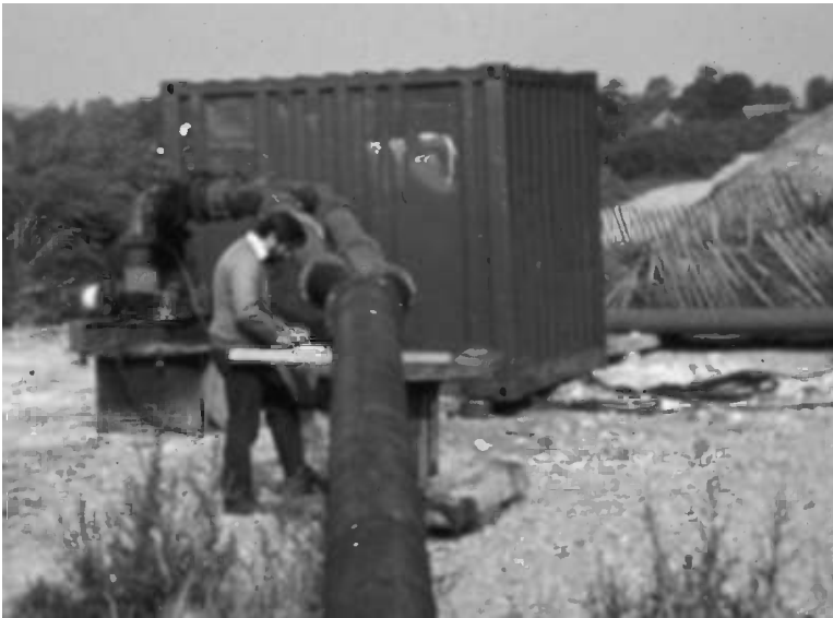
Figure 7.3 Two large submersible pumps (and two rising mains) are installed for test pumping of this abstraction well in the Chalk aquifer at Gatehampton, southern England. The pumped water is discharged to the River Thames. Photo by David Banks
