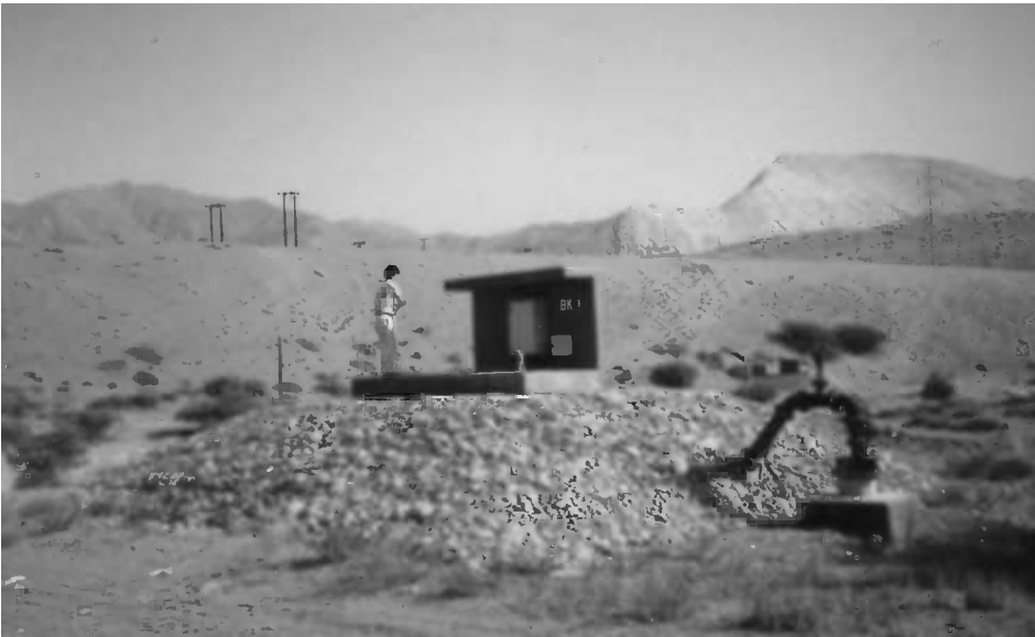
Figure 5.29 A wellhead arrangement at a wadi site in northern Oman which is susceptible to occasional flooding. The valves and other pipework are located in a gabion-protected concrete chamber, whilst the electric control panel is on top of the chamber (where the hydrogeologist is standing) to keep it as high as practicable above anticipated flood levels. The well, which has a watertight cover, is outside the chamber, so as to be accessible for maintenance. Photo by Bruce Misstear
