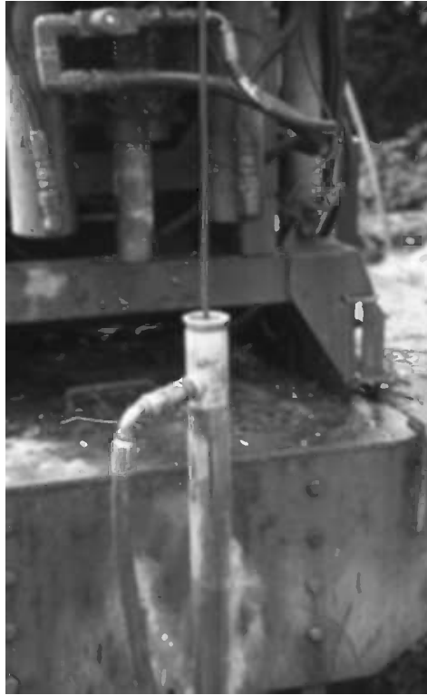
Figure 5.11 Retrieving core using the wire-line system, western Ireland. Photo by Bruce Misstear
