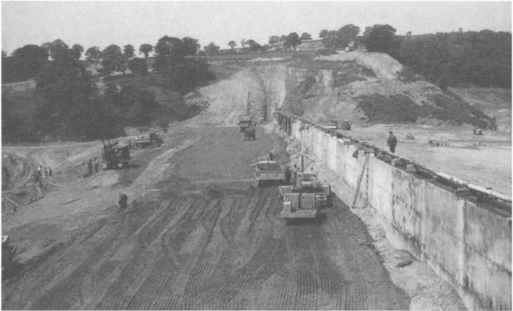
Tittesworth 33 m high earth dam of crushed sandstone under construction 1962, showing articulated concrete corewall. (Engineers: Binnie & Partners)
