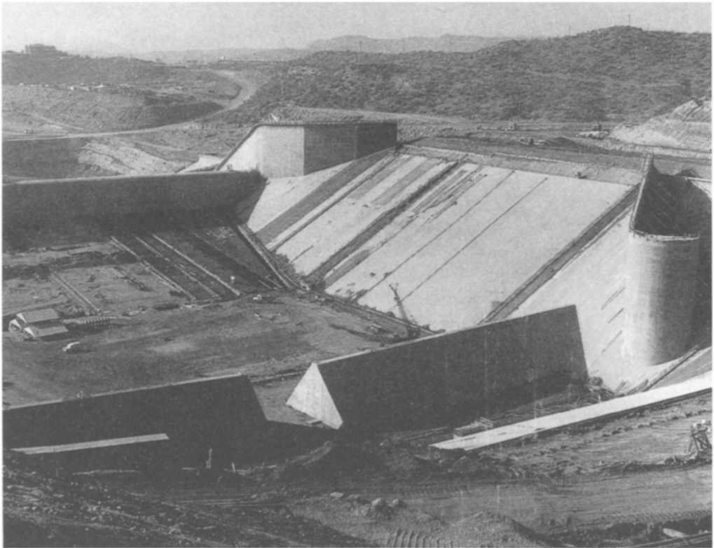
The 138 m high Mangla earth dam main spillway, Pakistan, under construction 1967, designed for 25\,000\text{ m}^3/\text{s} overflow rate. (Engineers: Binnie & Partners)
