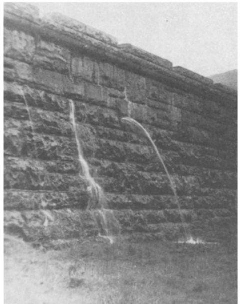
Leakage through the masonry joints of the Upper Neuadd dam, 1963, due to acid moorland impounded water attacking the lime constituent of the mortar
