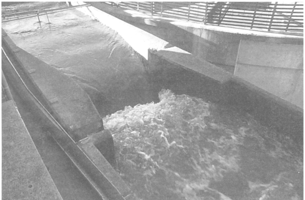
A 140 Ml/day flume for flow measurement and mixing of injected coagulation chemicals upstream in the downstream hydraulic jump, Lartington treatment works, Northumbrian Water, UK
