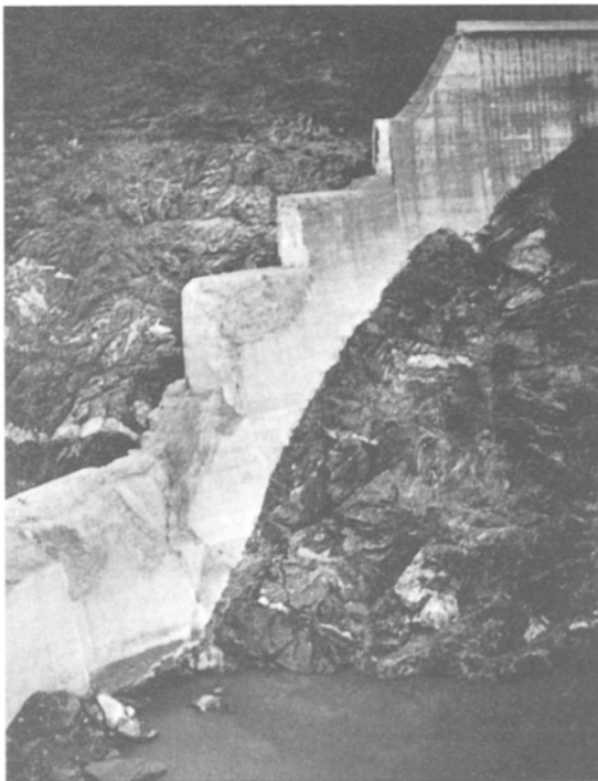
The failed left abutment of the Malpasset concrete arch dam, France, 2 December 1959 showing the crushed concrete due to weakness and movement of the abutment. (Photo: Water Power)
