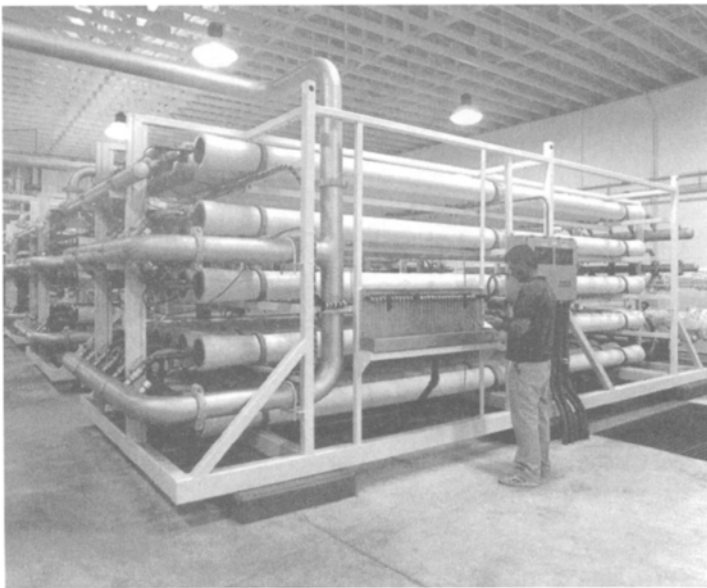
An 11 Ml/day reverse osmosis desalination plant at Kill Devil Hills, North Carolina USA, 1989. (Engineers: Black & Veatch USA)
