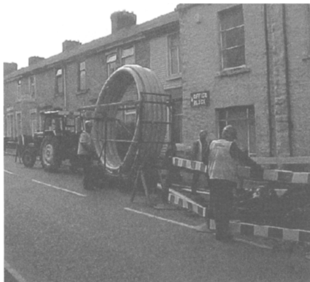
Relining 150 mm (6 inch) diameter cast iron main with 160 mm MDPE coiled pipe using the pipe bursting method
