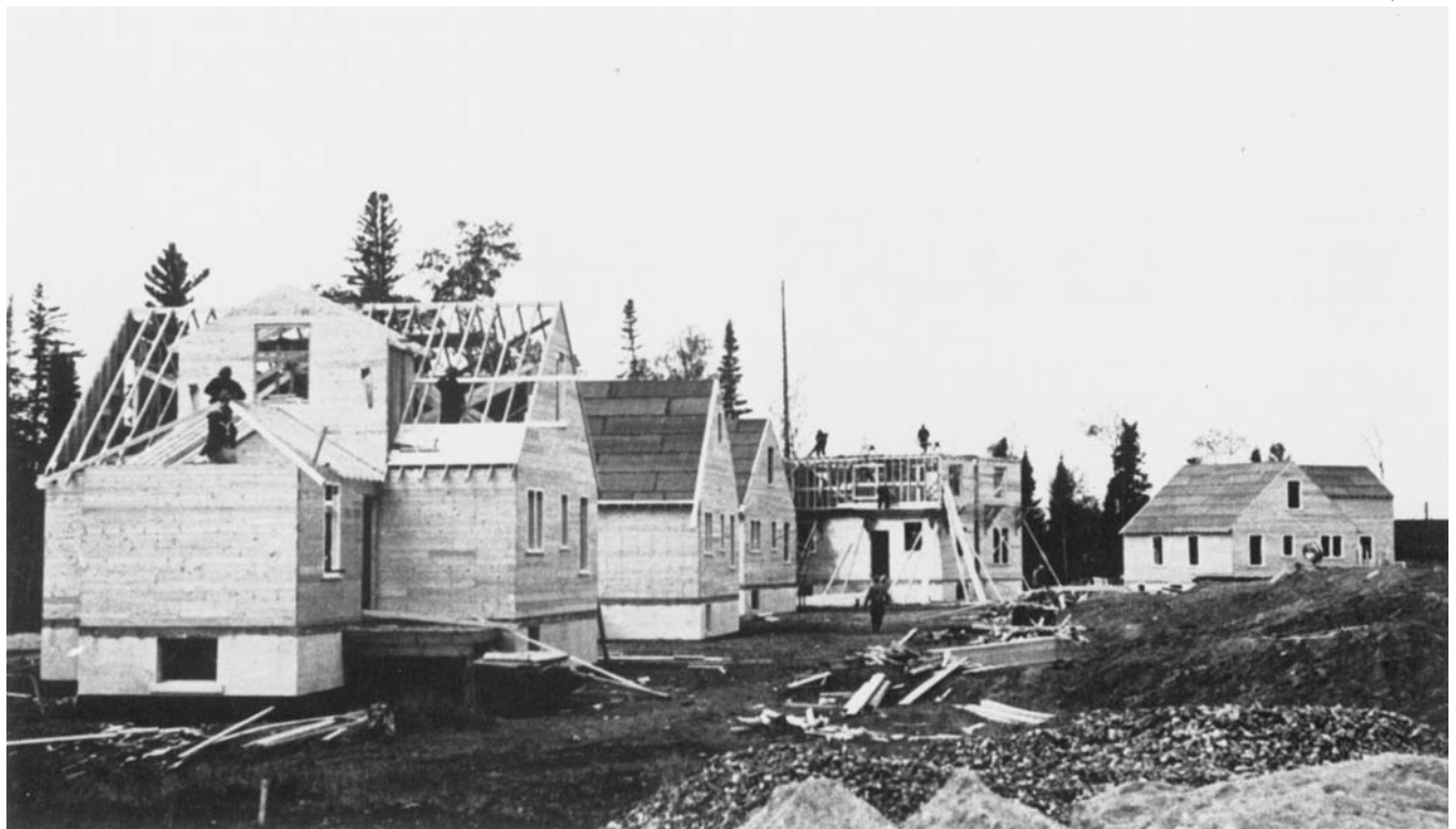
Construction of homes for the staff at the Ear Falls colony was in progress when this photo was taken.
