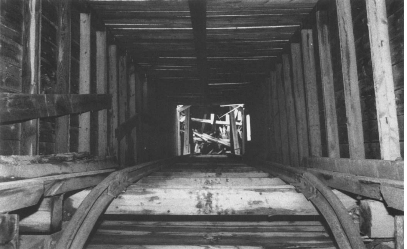
Desolate silence prevails in the incline shaft of the St. Anthony Gold Mine headframe, located on the north end of Sturgeon Lake.
