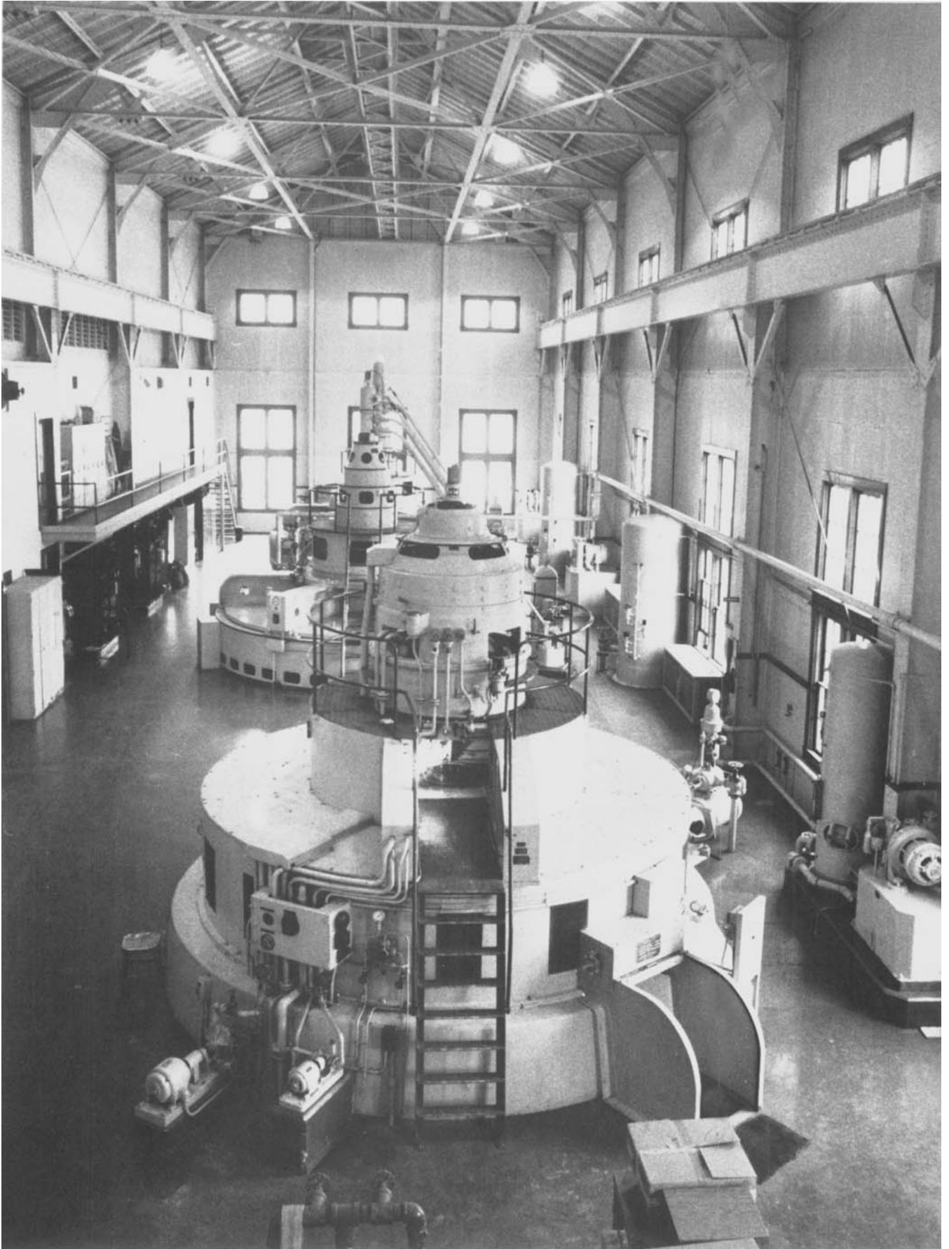
The Ontario Hydro generating station at Ear Falls continues to function smoothly today.
