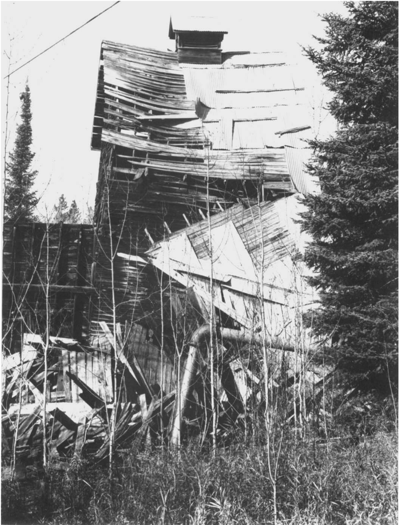
Looking like a crumpled accordion, this abandoned shafthouse at the Laurentian Mine is slowly succumbing to climate and structural fatigue.
