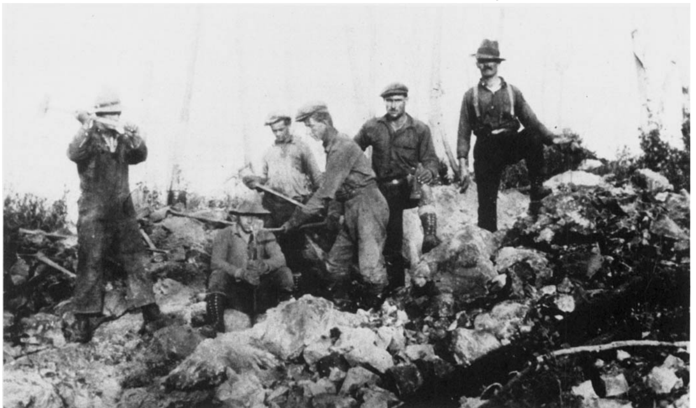
Bushwhackers here are shown punching out by hand the "coyote holes" for dynamiting the boulders while building the CNR north of Lake Superior. One man held a steel hand drill in position while three or four others swung sledge hammers in rhythm to dig out
