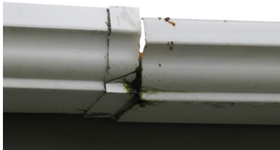
Fig. 16 Gutter joint failure
