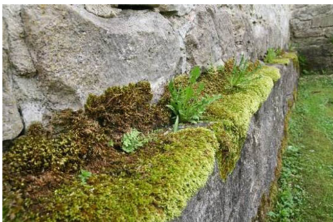
Fig. 4 Protruding foundation wall ought to have sufficient slopes and a cornice to lead the water away safely. Foundation wall has been wet enough to facilitate the growth of moss
