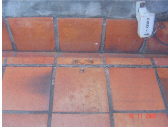
Fig. 17 Monitoring station and pins fixed to the south terrace, fifth floor (Nov 2005 —Cerme Engenharia)
