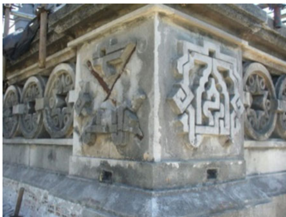
Fig. 34 Ornament on the fifth-floor terrace, north wing, external wall—the damage goes deep into its metallic structure (Mar 2014)
