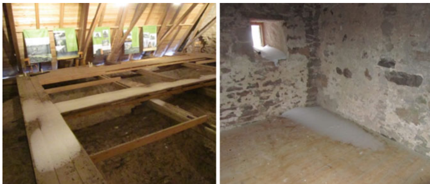
Fig. 26 Left Snow has penetrated the roofing and will cause an additional moisture load on the structure once it melts. Right Snow has penetrated a window
