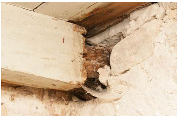
Fig. 14 Wooden beam has become a suitable habitat for rot. Wooden cladding on the interior surface has speeded up the process
