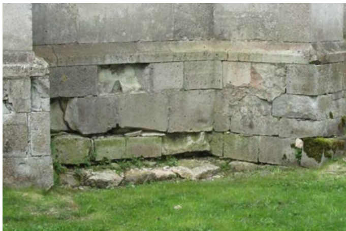
Fig. 3 Ground around the church is sloped towards the building and leads water to the structure, frost damage caused by excess moisture is also visible
