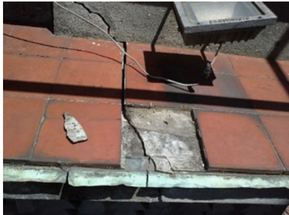
Fig. 30 Structural damage seen at the seventh floor, north wing, eave: crack opening, affecting also the copper plaque (Feb 2014)
