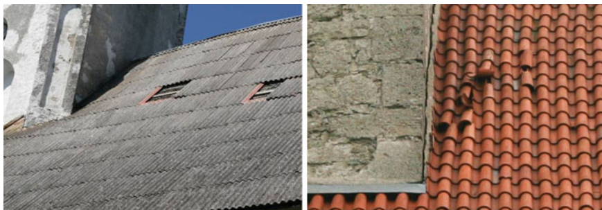
Fig. 24 Left Loss of already one sheet of cement fibreboard roofing causes a serious problem—large area of the roof is exposed to the elements. Right Displaced monk and nun type of tiles cannot be refitted from the inside and due to the lack of specialized equipment, the leaks in rural areas might be exist for a long time
