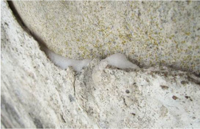
Fig. 11 Damaged plaster contributes to wetting of the wall and accelerated corrosion of the building components
