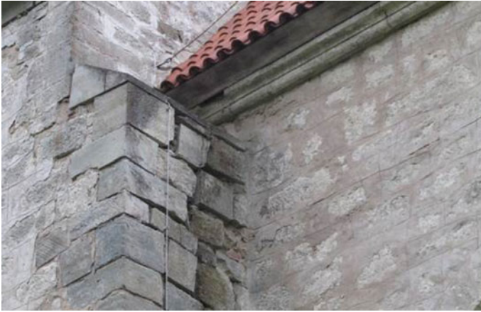
Fig. 9 Due to incorrectly designed details, concentrated amounts of rainwater are able to penetrate the wall
