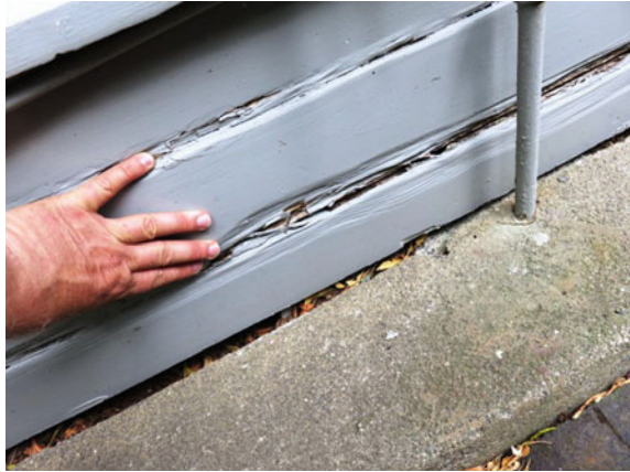
Fig. 20 Weatherboard decay probably due to ground moisture
