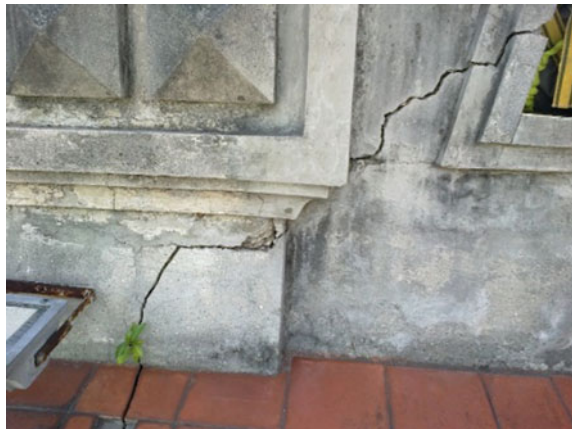
Fig. 21 Pathologies: cracks on the parapet, fissures on mortar and biological growth (Feb 2014)
