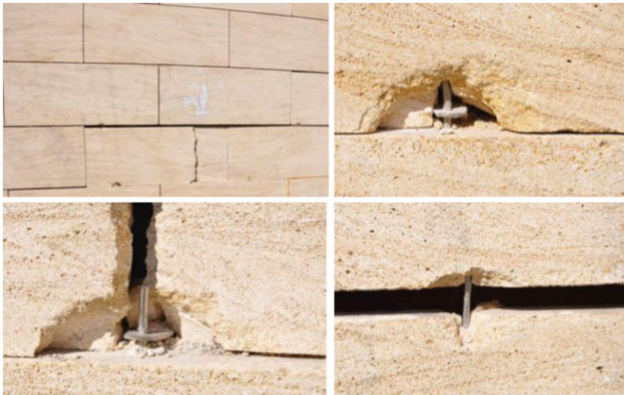
Fig. 6 Panel break around the anchor points
