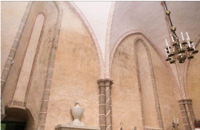
Fig. 17 Growth of mould and pink bacteria can indicate moist surfaces and cause discoloration.
