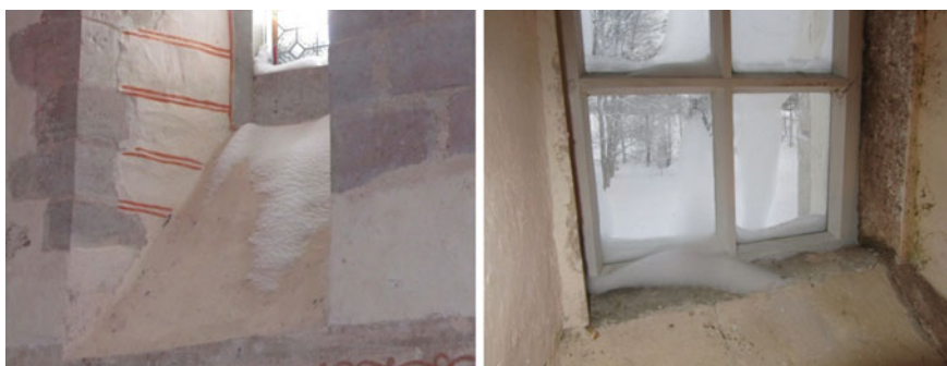
Fig. 19 Snow has penetrated the windows due to low airtightness, possibly wetting the structure once it melts
