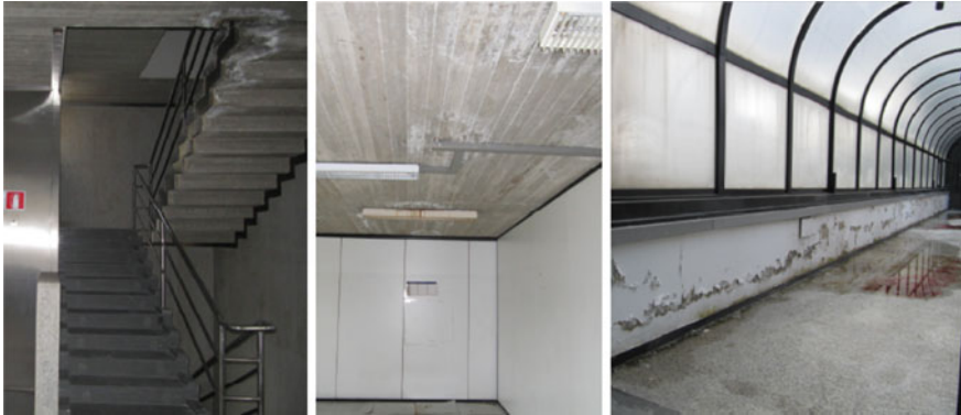
Fig. 7 Efflorescence and surface wash in the stairwells (on the left ) and on the floors of the higher levels corrosion (on the center ); gallery decay (on the right )
