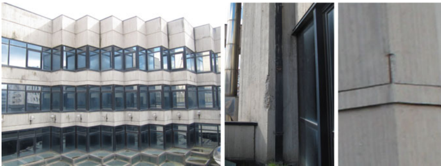
Fig. 6 Leaching on the surfaces of facing reinforced concrete (on the left ); corrosion of reinforced steel (on the center ); exposure of reinforcing bars (on the right )
