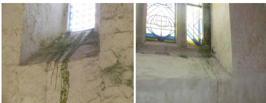
Fig. 20 Results of surface condensation and leaks on the interior surfaces of window sills: growth of algae, salt efflorescence
