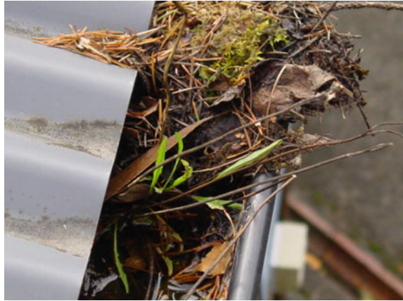
Fig. 15 Guttering blocked by vegetation
