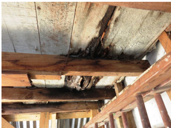
Fig. 19 External deck timber decay
