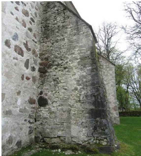
Fig. 6 Roof covers only part of the buttress resulting in discoloration, frost damage, and wetting of the wall
