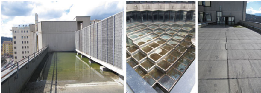
Fig. 5 Design errors and defects of the cover: water stagnation (on the left and center ) and decay of the roof waterproofing (on the right )
