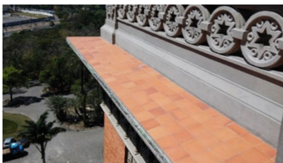
Fig. 37 External aspect of the parapet and the eave after the intervention—fifth-floor terrace (Sep 2014).
