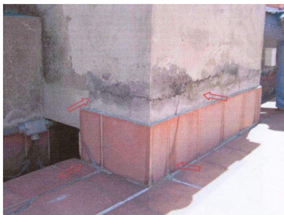
Fig. 19 Cracks on the mortar indicating the displacement of the waterproofing blanket (Nov 2005 —Cerme Engenharia)
