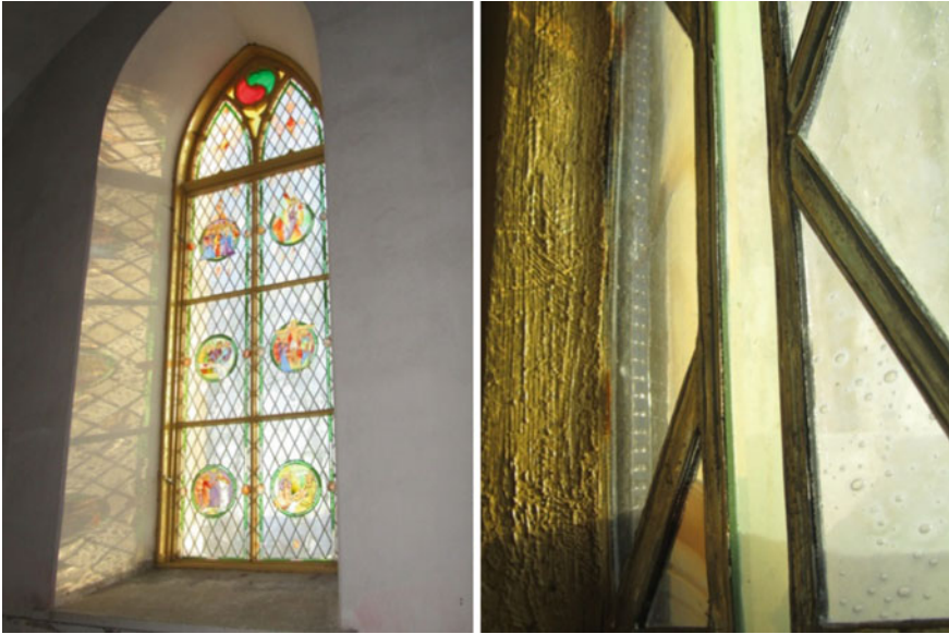
Fig. 21 A modern glazing unit on the exterior side of the historic window preserves the original appearance while reducing thermal conductivity and air leakages
