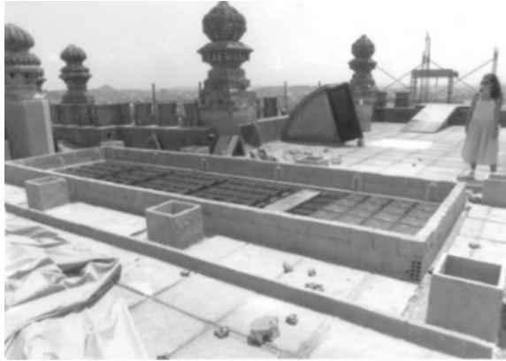
Fig. 14 Construction of the shelter dome for the skylight on the seventh-floor terrace (1990)
