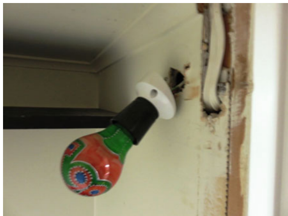
Fig. 27 Exposed live wiring
