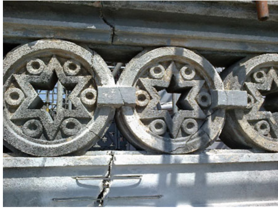
Fig. 29 Wide cracks in the structure, treated with stainless steel clamps (Apr 2014)
