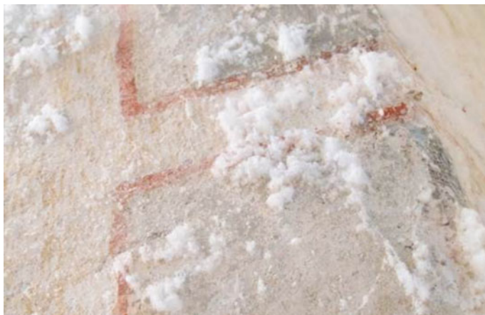
Fig. 12 Efflorescence of salts can disfigure and ruin historic paintings
