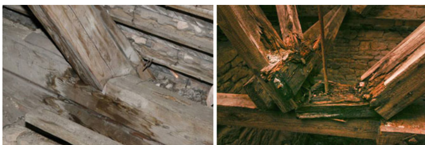
Fig. 29 Left Leaks and contact with a moist wall cause wood decay. Right Almost fully decayed connection needs prompt repairs
