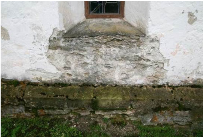
Fig. 10 Proper detailing of façade elements has an important role in the service life of the whole wall. Window flashing made of mortar has failed to lead the water away safely
