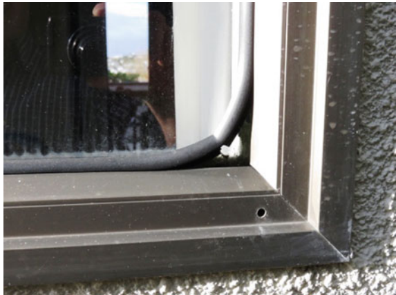
Fig. 23 Aluminum window frame rubber seal has moved
