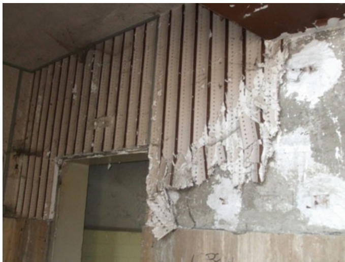
Fig. 11 Degradation of walls in the circle area
