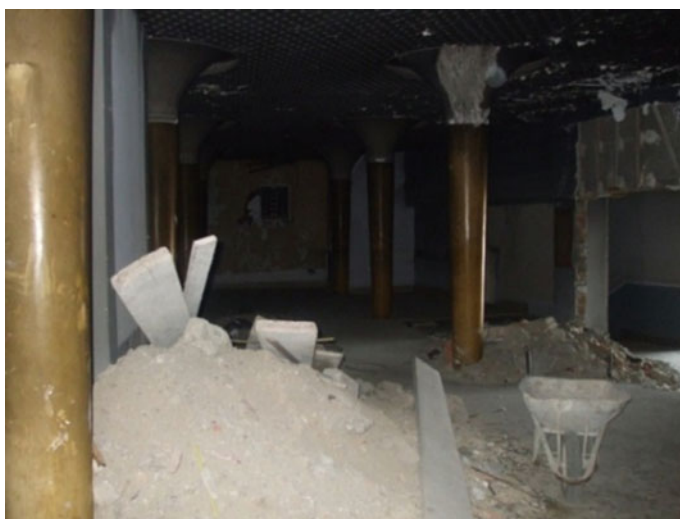
Fig. 10 Degradation of the foyer
