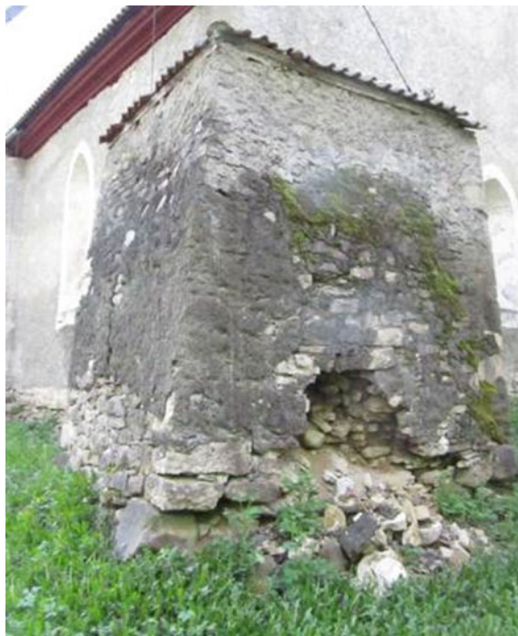
Fig. 7 Only surface layers of the masonry wall were built using binder, damage to these layers can cause collapse
