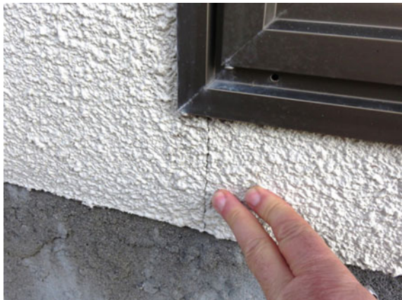
Fig. 26 Crack in monolithic cladding allows water ingress
