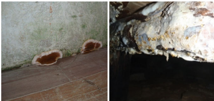
Fig. 31 Wooden floor infected with rot causing fungi from the top ( left ) and below ( right )
