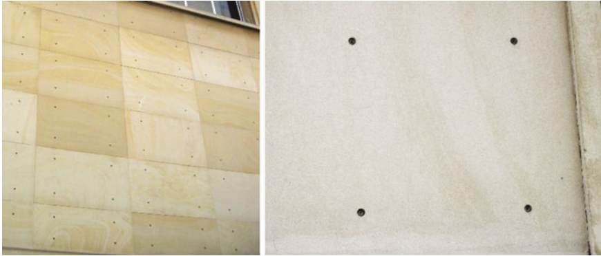
Fig. 11 Stone panels previously taken with mortar and repaired with screws
