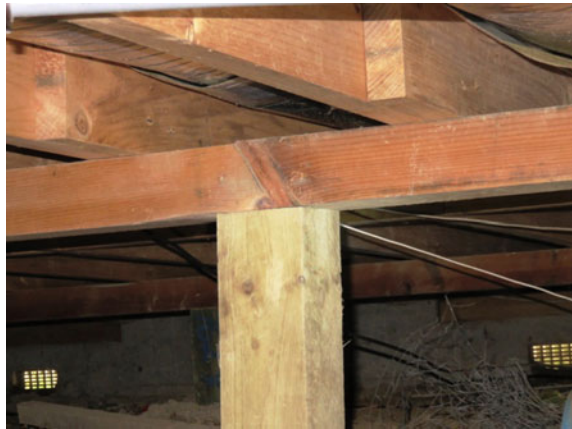
Fig. 7 Untreated floor bearer rests on treated pile
