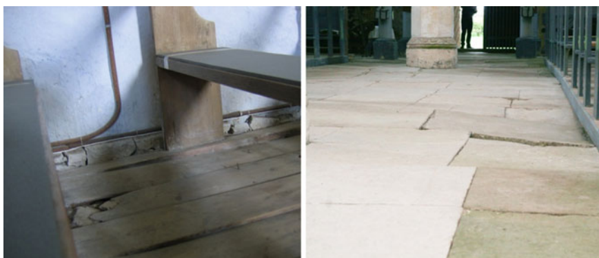
Fig. 32 Left Wooden floor with fungal infection. Right Uneven stone floor
