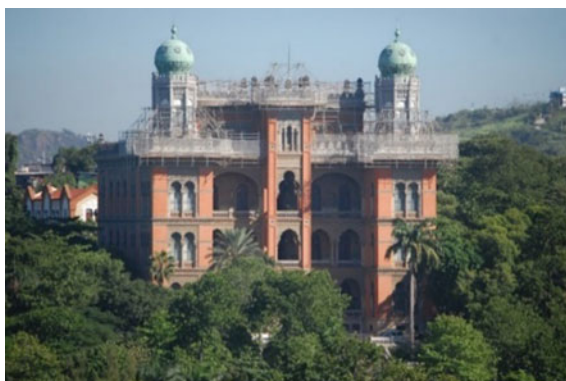
Fig. 23 Suspended scaffolds covering the front of the Pavilhão Mourisco's terraces, on the intervention's first phase (Apr 2014)
