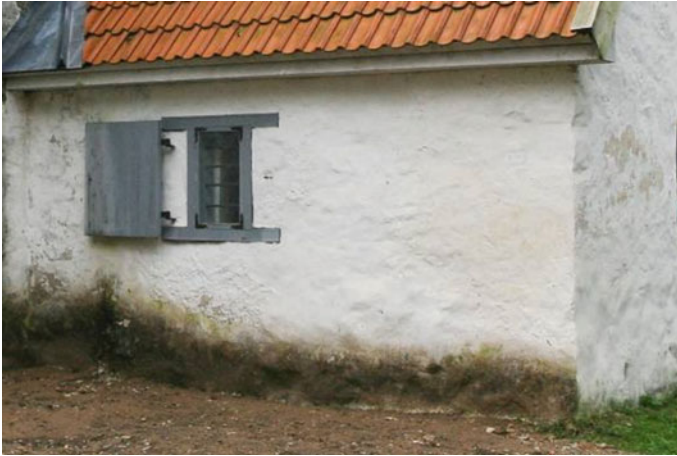
Fig. 5 Water falling from the gutterless eaves moistens the façade while exhausting the frost resistance of the plaster, splashing water also carries soil—the foundation wall is dirty and suitable habitat for algal growth
