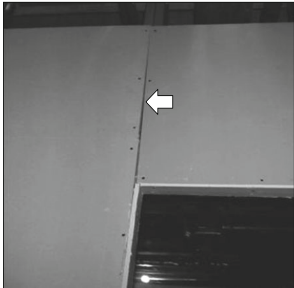
Fig. 16 The vertical crack on the corner of doors in plasterboard walls (not original—just for example)
