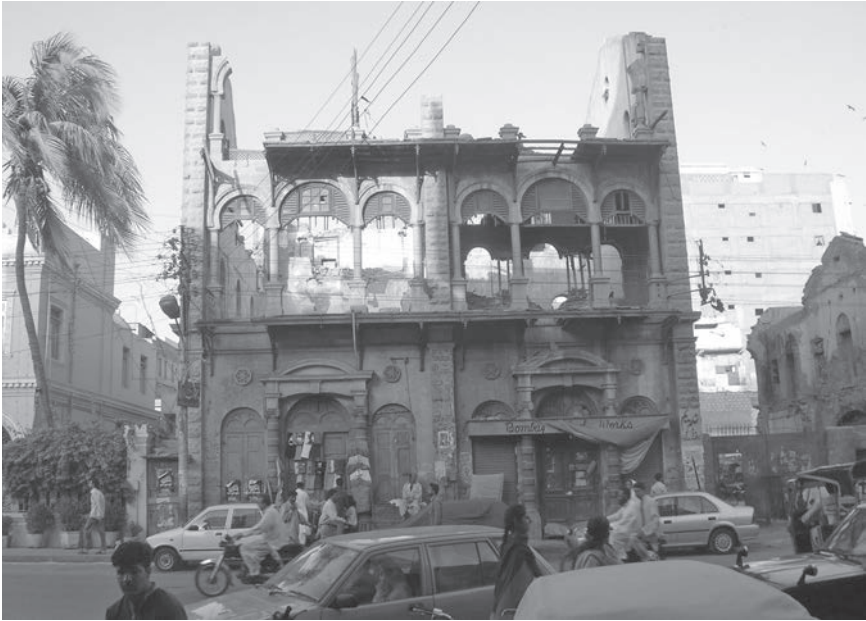
Figure 3.4 Gol Wala Building in Dr. Daud Pota (Frere) Road/Sharah-e-Iraq (Clarke Road), Karachi. Issues such as multiple private ownership with several shares make it more difficult for these disused colonial commercial buildings to be preserved. Courtesy Ayesha Agha Shah, University of Bahrain.
