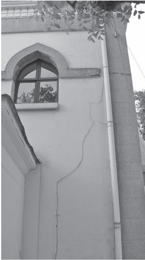
Figure 5.1 Cracks in the courtyard and minaret of the sixteenth-century Hüseyin Ağa Mosque. The cracks occurred due to the movement of the foundations of the mosque, a consequence of the deep excavations to build the subterranean levels of the shopping mall next to it. Image courtesy Emel Ardaman, Mimar Sinan Fine Arts University.
