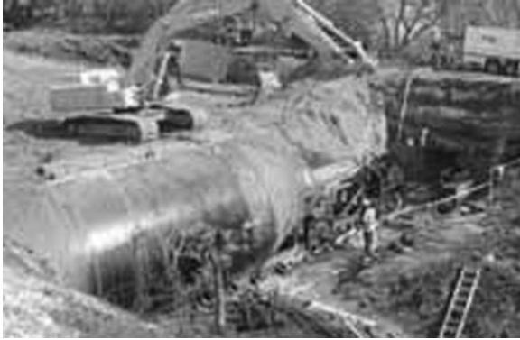
FIGURE 6-8. This giant casing was rammed 60 ft (18 m) under Iowa Interstate Railroad tracks.
