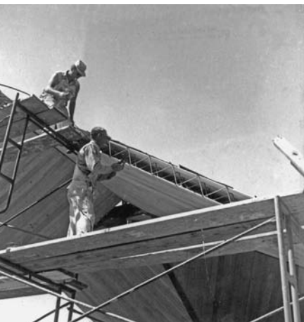
Construction of the Phillips house using Trus Dek, Boise, Idaho, 1958. Photos: Art Troutner. Used with permission.
