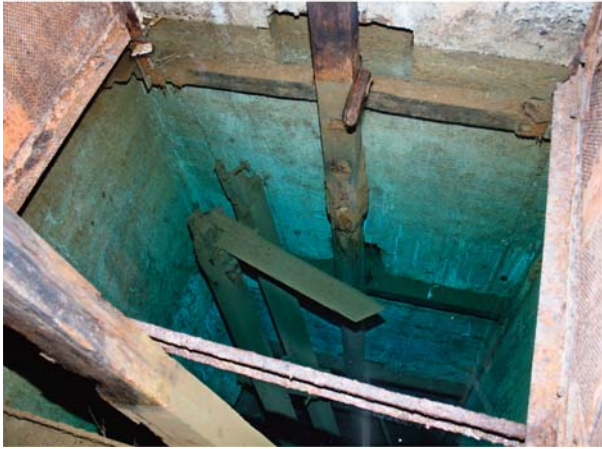
Fig. 36. Rotten shaft furniture in a flooded shaft of the closed Schwaz/Austria dolostone mine. The water surface is just a little bit below the left corner of the shaft.
