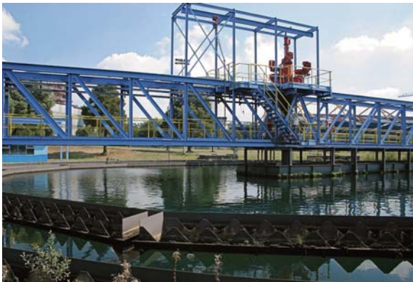
Fig. 88. Radial flow clarifier of an active mine water treatment plant at As Pontes lignite mine (Spain).
