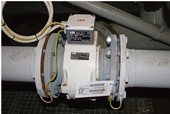
Fig. 60. Magnetic-inductive flow meter in the Schwarze Pumpe /Germany mine water treatment plant.
