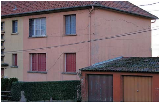
Fig. 33. Damaged house because of surface subsidence above an abandoned iron ore mine in Roncourt, Lorraine/France.
