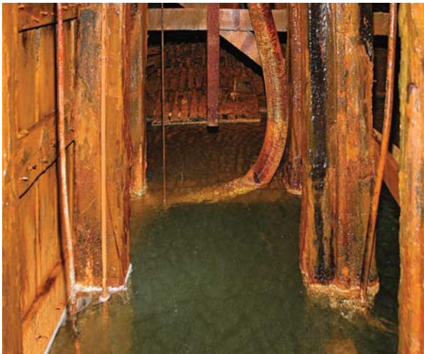
Fig. 15. The flooded Reiche Zeche shaft of the Freiberg/Saxony mining field (2 March 2006). The brown colour is a result of ochre precipitates as a consequence of the catastrophic flooding of August 2002. Width of picture approximately 2 m.
