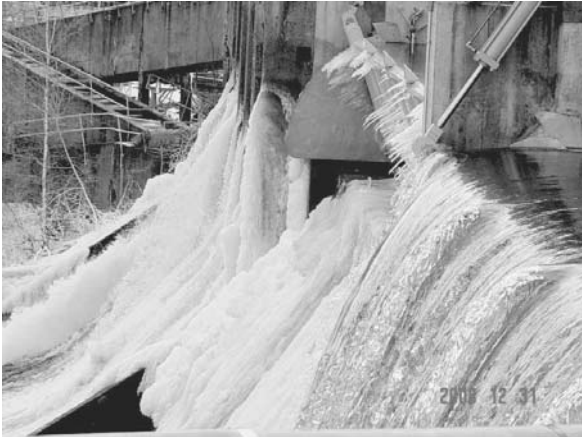
Figure 3-3. Icing of spillway gates.
