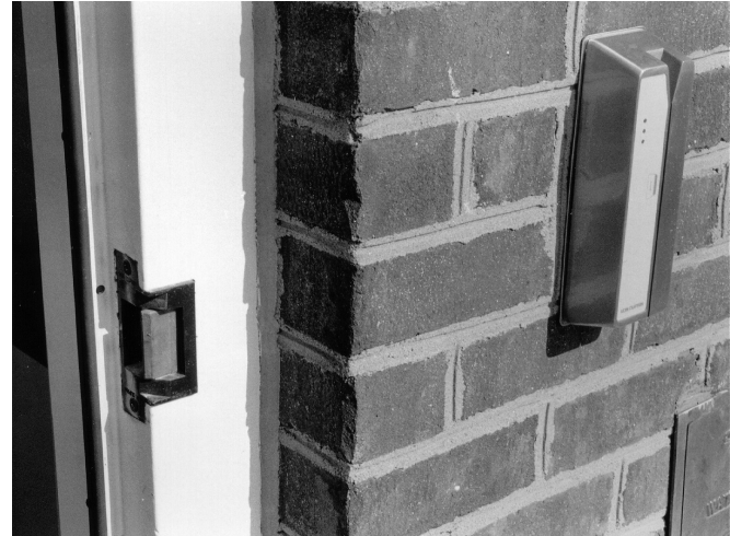
Fig. 8. Swipe card reader for building access (Courtesy: Von Duprin Co.)
