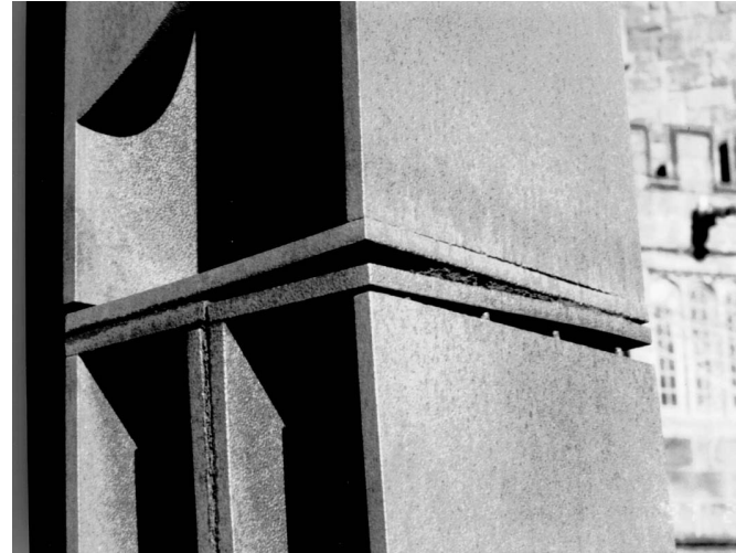
Fig. 7. Corrosion between bolted steel plates.
