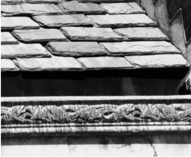
Fig. 1. Built-in gutter. Yale University Hall of Graduate Studies. 1932. James Gamble Rogers, Architect.
