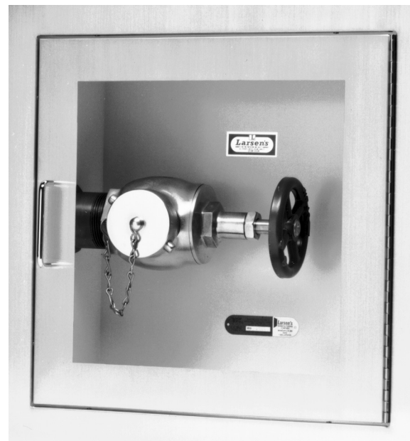
Fig. 1. Standpipe valve in recessed cabinet
