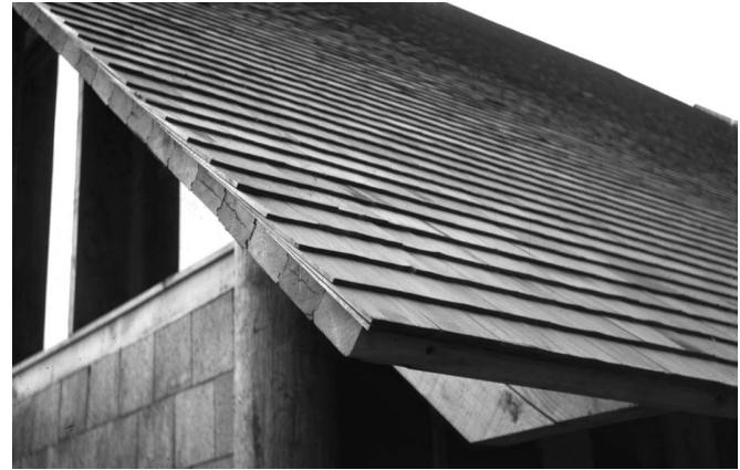
Fig. 11. Western redcedar shingle roof on First Presbyterian Church, New Haven, CT. John Dinkeloo, Architect. 1966.
