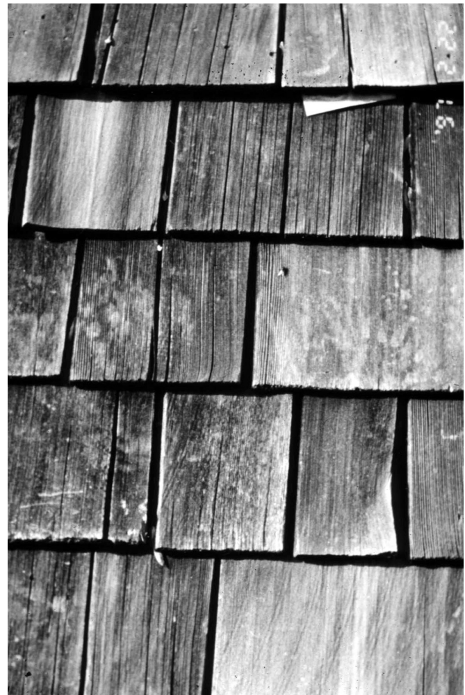
Fig. 12. Split shingles: the first and third course joints lined up in many places. When the intermediate shingles split, there was a clear path through the shingles for rain water.)
