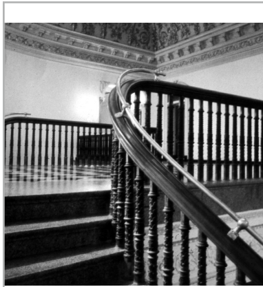
Special attention to top of stairs
