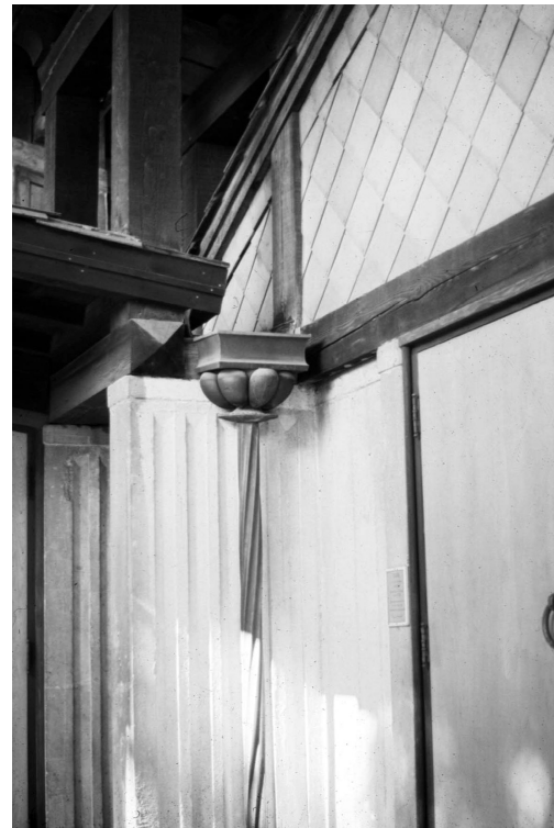
Fig. 7. Scupper and leader head, First Church of Christ, Scientist, Berkeley, CA. Bernard Maybeck, Architect.
