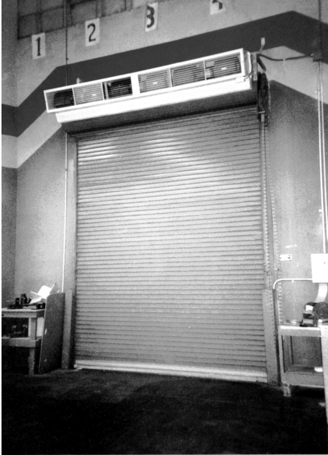
Fig. 4. Air curtain installed over bay door on interior of loading dock. (Courtesy: Mars Air Door)
