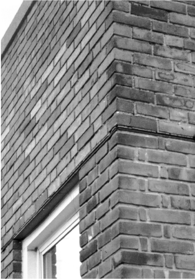
Fig. 5. Brick masonry cracked by expansion of carroding
