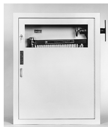
Fig. 2. Listed rack for fire hose
