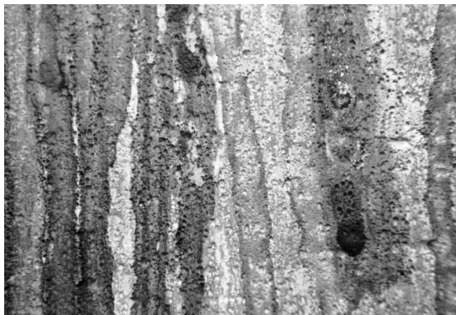
Fig. 6. Pitting and corrosion of copper flashing as a result of runoff from membrane roof.
