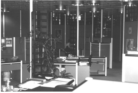
Fig. 9. Modular reconfigurable ceiling with plug-in capability to add or subtract fixtures with various workstation layouts. Colonia Headquarters, Cologne, Germany (ABSIC).
