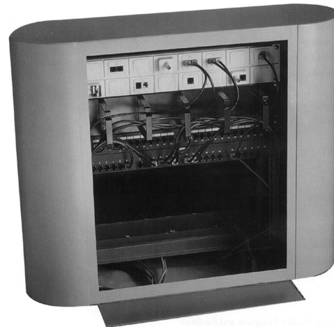
Fig. 13. Distributed satellite closet serving 10,000 sq. ft. (930 sp. meters) offer greater control, reliability and flexibility to meet individual needs (POWERFLOR™).
