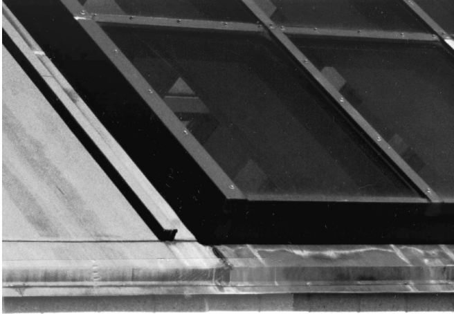
Fig. 13. Copper roof with well-developed light green patina. Below the glass and aluminum skylight, the patina has been removed by acid runoff.
